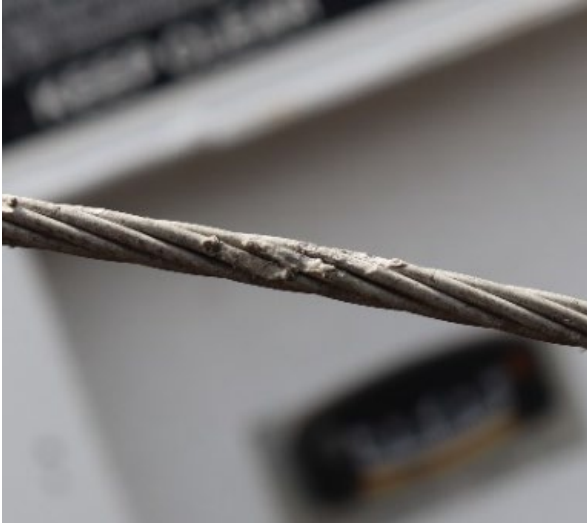
Figure 4: Pitting on the south conductor.
