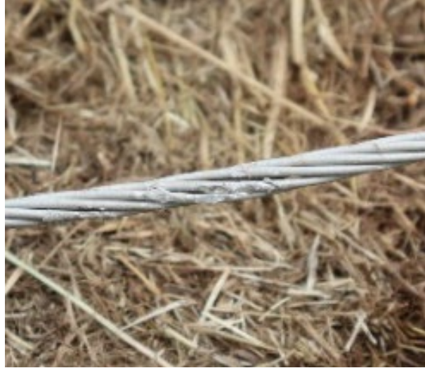
Figure 5: Pitting on the middle conductor.
