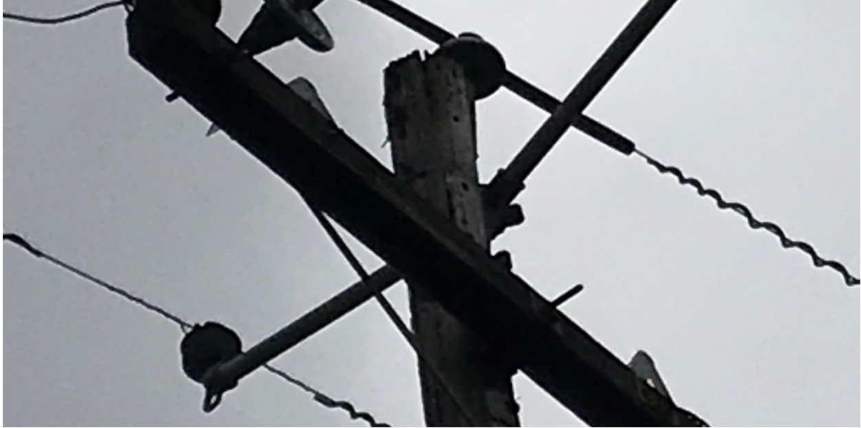
Figure 14: Damaged Top of Pole 102286081. 62
