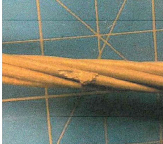
Figure 13: Arcing evidence on conductor, as photographed by EFI Global.
