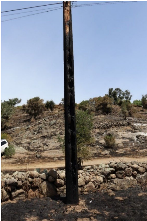
Figure 6: Burnt pole at east end of span.
