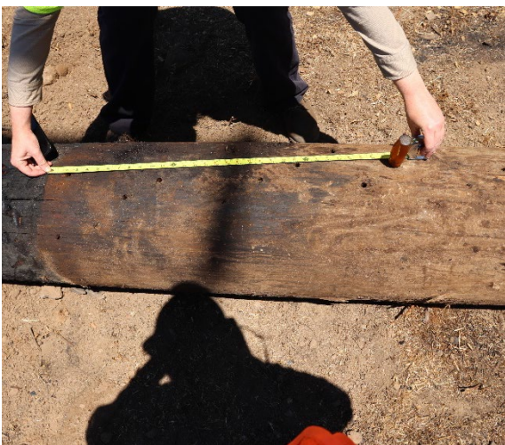
Figure 9: Probing Pole 103949547 below grade.
