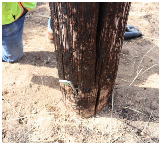
Figure 10: Probing Pole 102286081 above grade.
