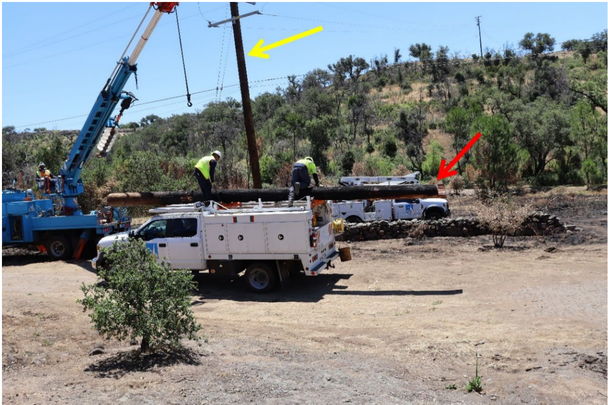
Figure 8: Burnt pole on east end of span (Pole #103949547) being removed and loaded into truck (red arrow). A new pole replacement installed directly adjacent to original pole location (yellow arrow).
