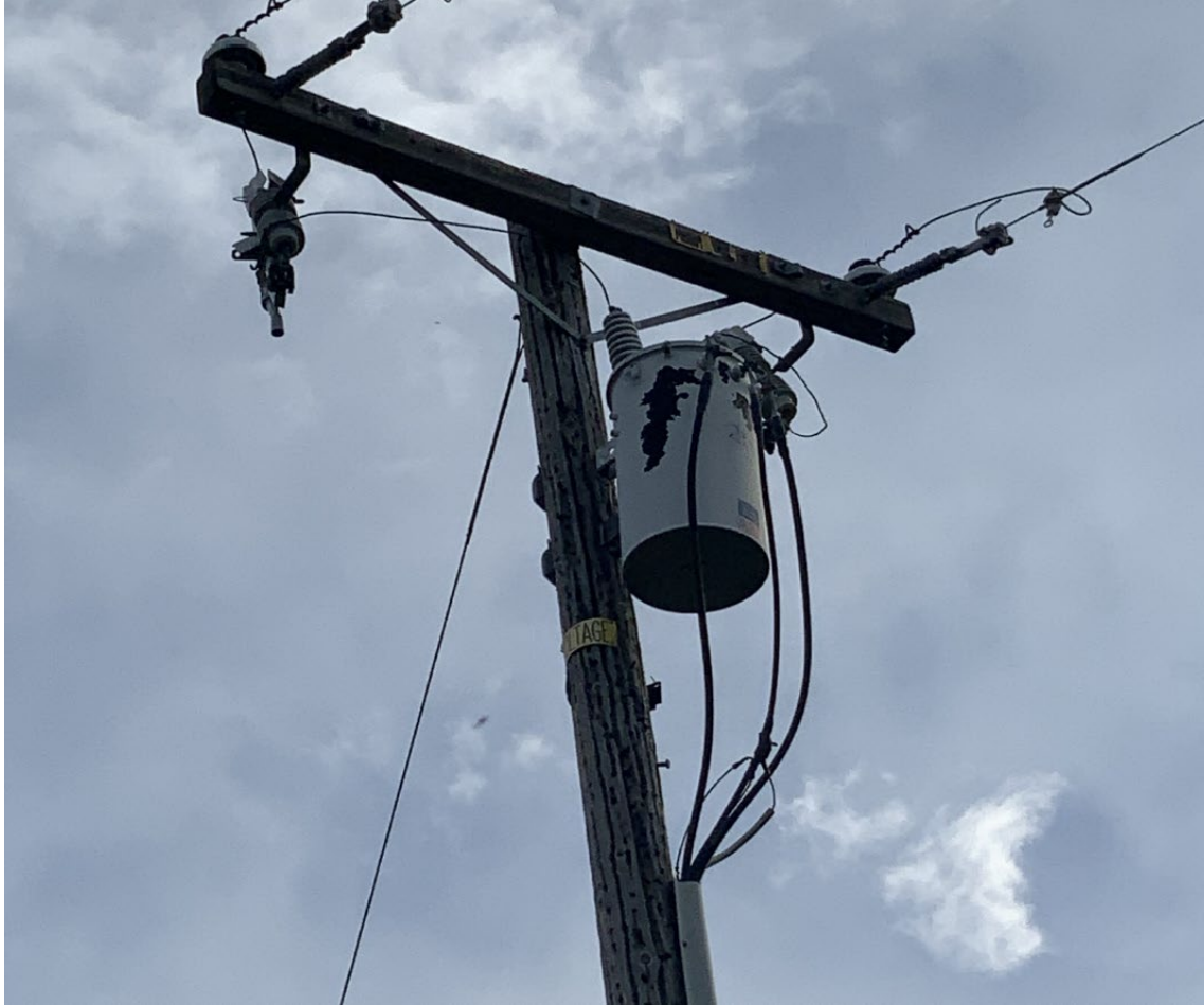
Figure 16: Pole 102285804 with signs of woodpecker damage. Photo taken by PG&E during 2021 FSR. 76
