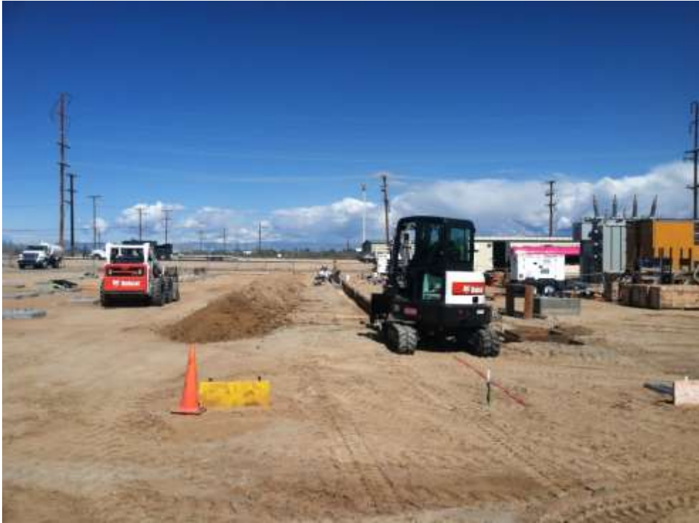
Figure 1 – Installation of the substation pad continued during the subject period. View north, 03/03/15.
