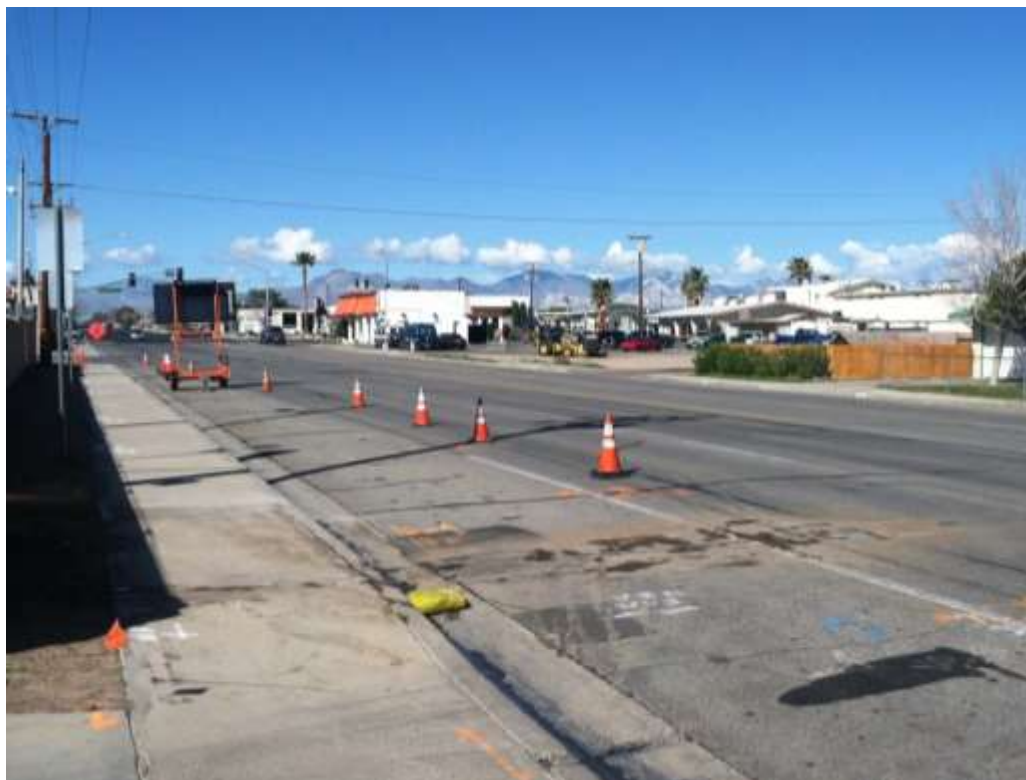
Figure 4 – Work areas were prepared for boring work, adjacent to the SCE Ridgecrest Service Center. View northwest, 03/03/15.
