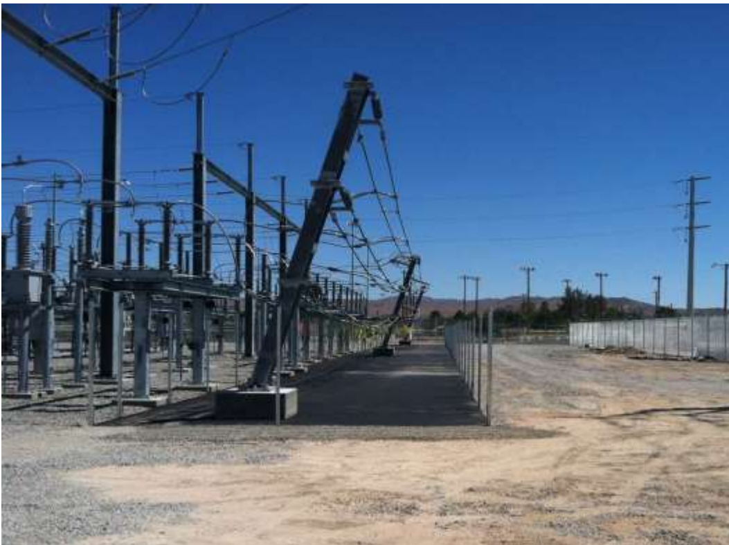
Figure 1 – Installation of interior fencing occurred during the subject period. View south, 6/16/15 above, 6/24/15 below.
