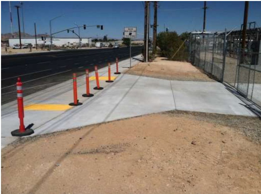
Figure 2 – Installation of a driveway apron was completed during the subject period. View east, 6/11/15 above 6/24/15 below.
