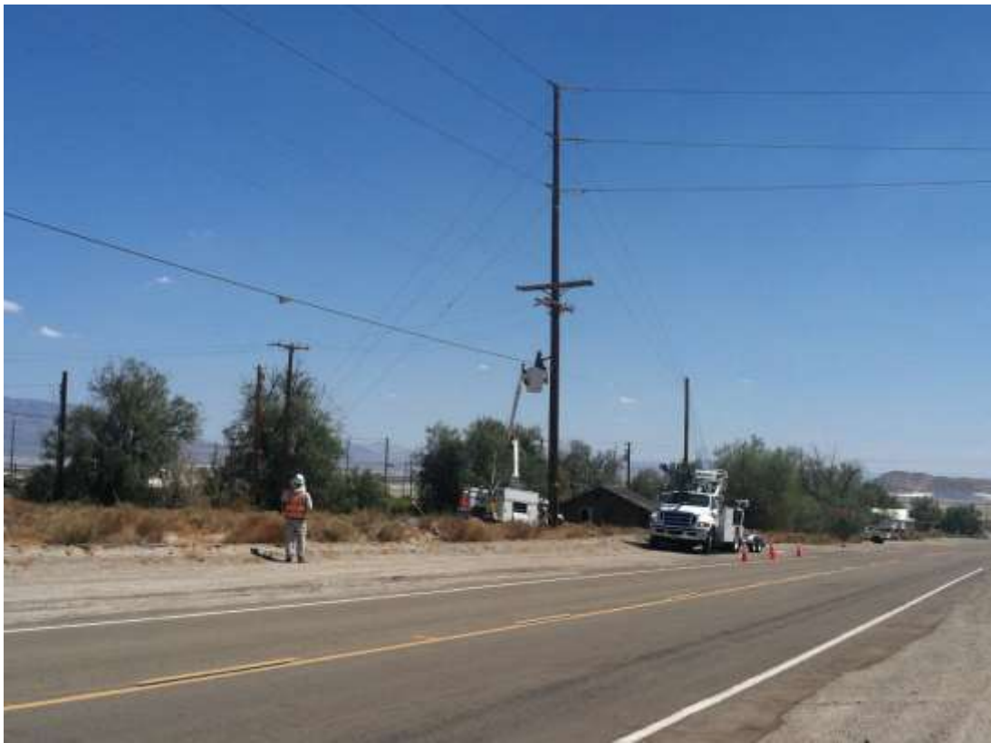
Figure 2 – Line crews installed telecom cables between McGen Substation and Searles Substation during the subject period. View southeast, 7/23/2015.
