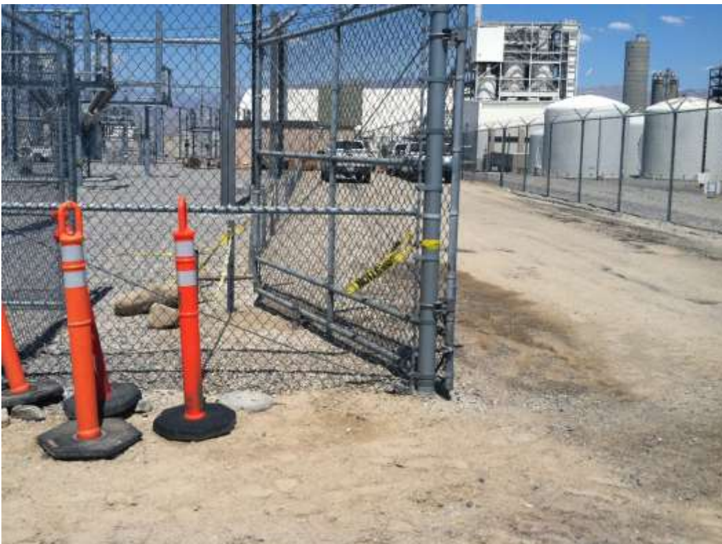
Figure 1 – Trenching and underground work continued at McGen Substation during the subject period. View east, 7/16/2015 above, 7/23/15 below.
