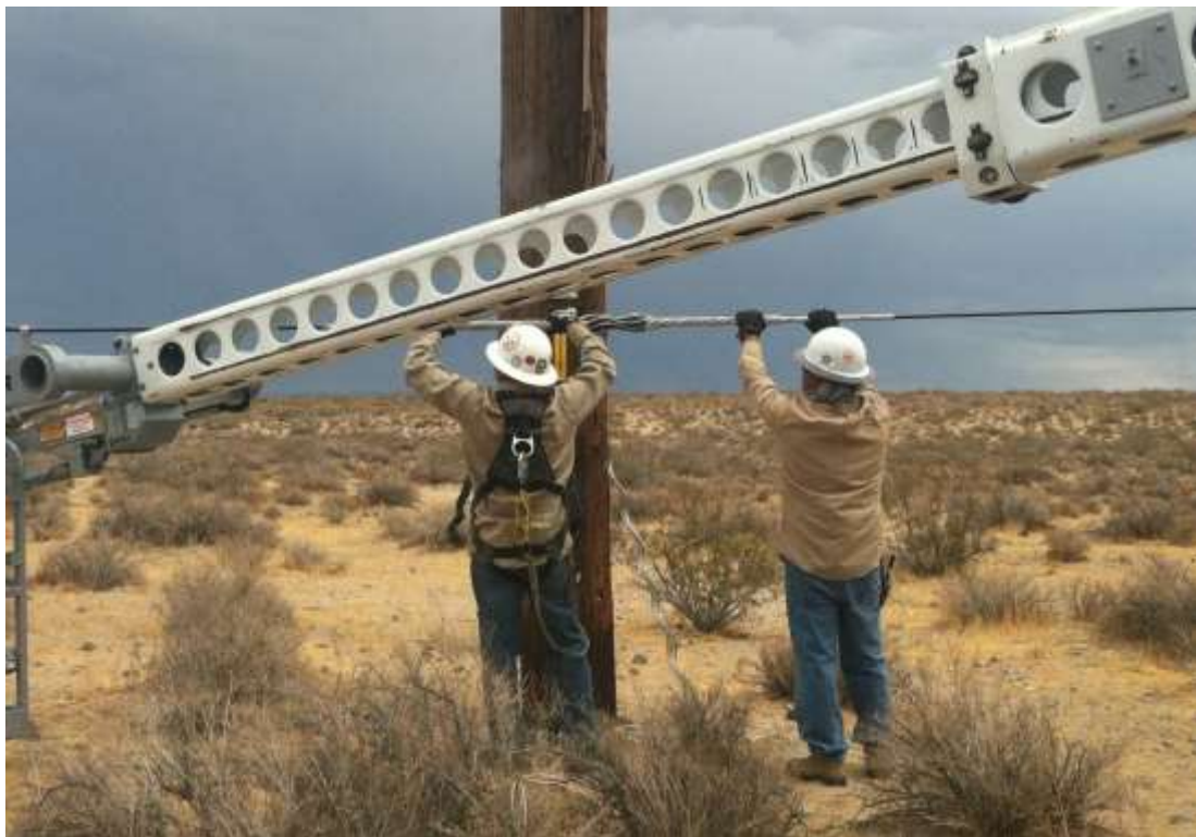
Figure 2 – Crews install fiber optic cables along the alignment, south of Inyokern Substation during the subject period. View east, 8/6/2015.
