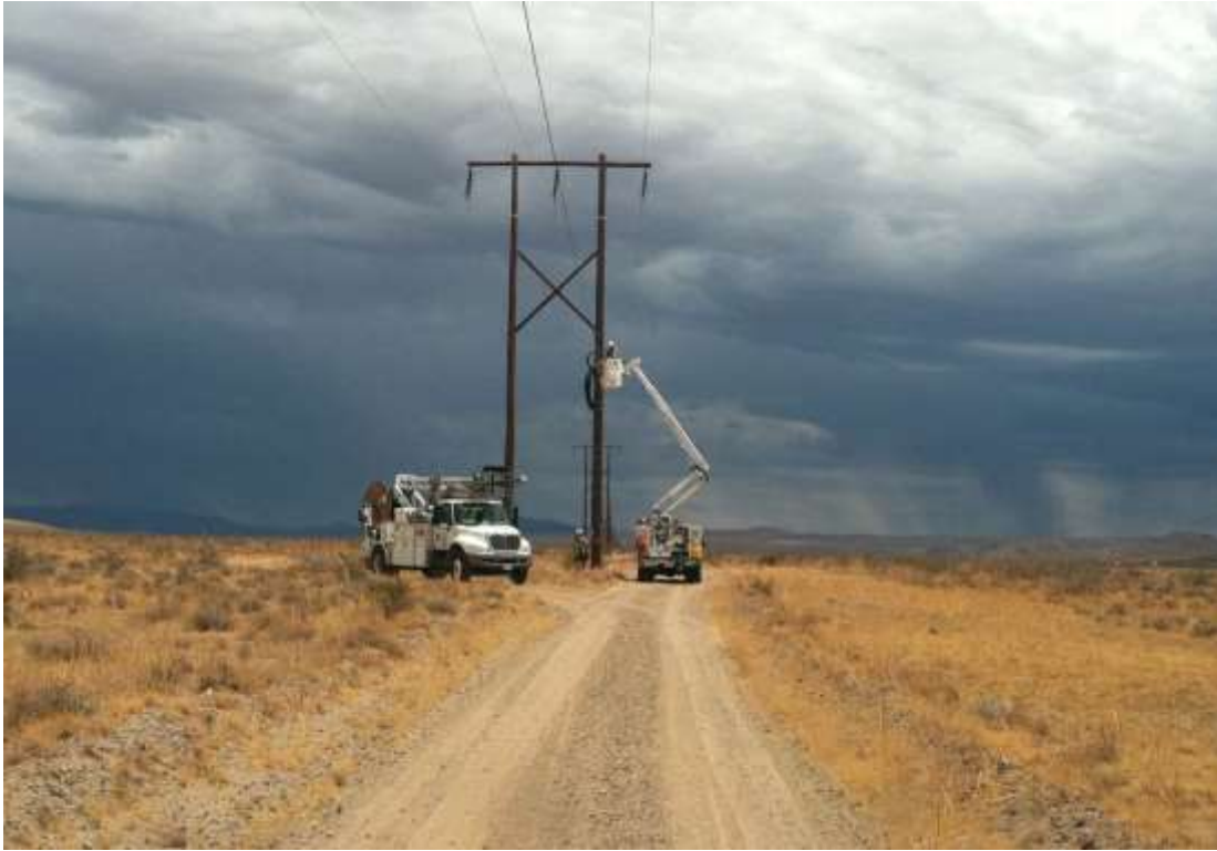
Figure 1 – Line crews installed telecom cables along the alignment south of Inyokern Substation during the subject period. View east, 8/6/2015.
