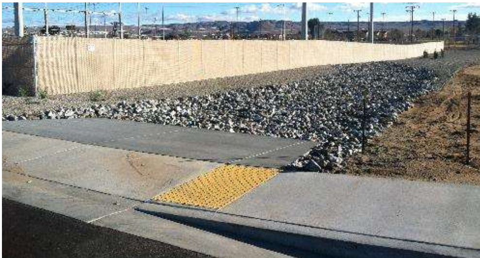
Figure 1 – A storm water channel was complete during the subject period. View southeast, 12/23/15 above, 12/29/15 middle, 01/07/16 below.
