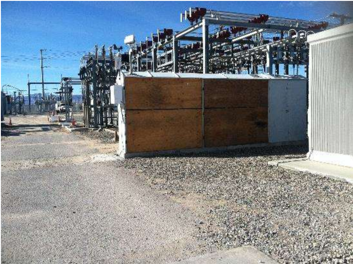
Figure 4 – Removal and modification work began with components of the original Downs Substation. View north 01/15/16.
