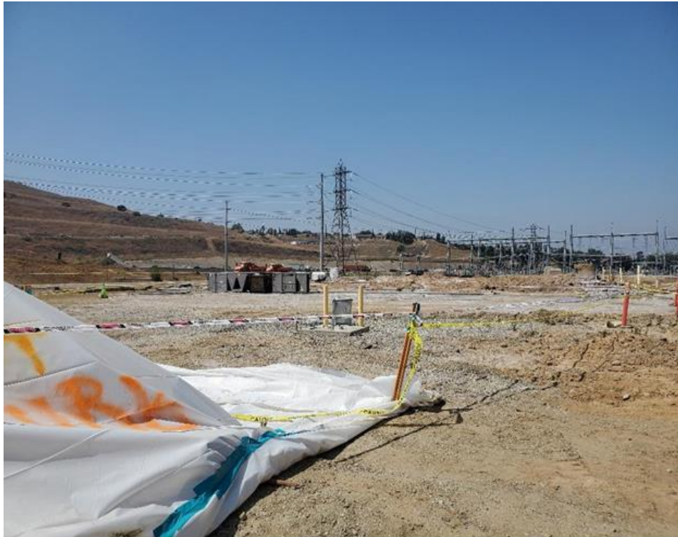
Photo 1: Exclusionary zone -asbestos containing construction material covered and roped off at the old Mesa Substation footprint area, June 12, 2020.
