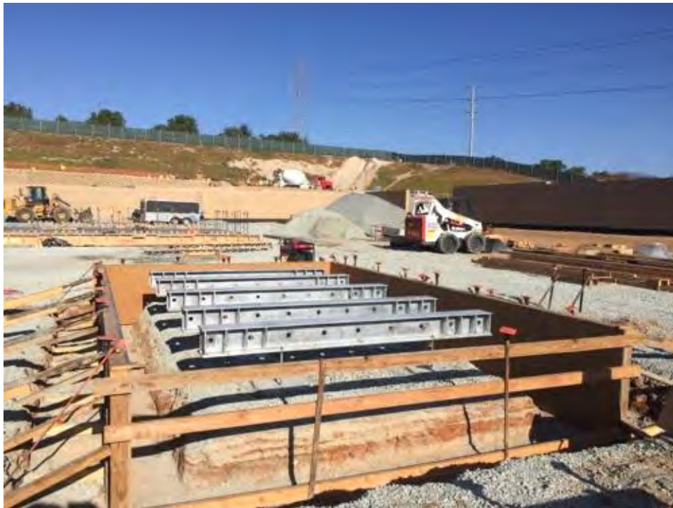
Caption Transformer footings
