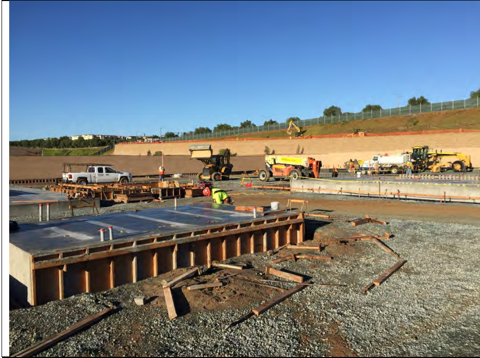
Photograph 3: Suffolk construction crew building electrical pads in the substation area occurred during the week of November 21, 2016.
