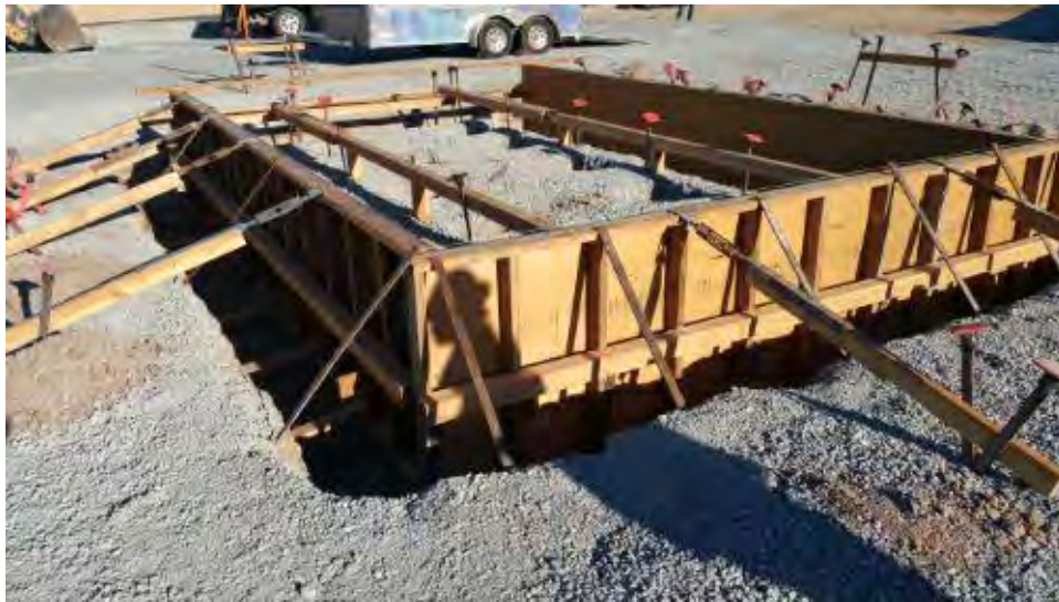
Caption Foundations lacked small mammal/reptile exit ramps.
