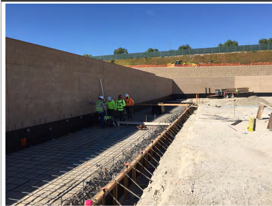
Photograph 2: Concrete formwork for the oil-catch basin occurred during the week of November 7, 2016.
