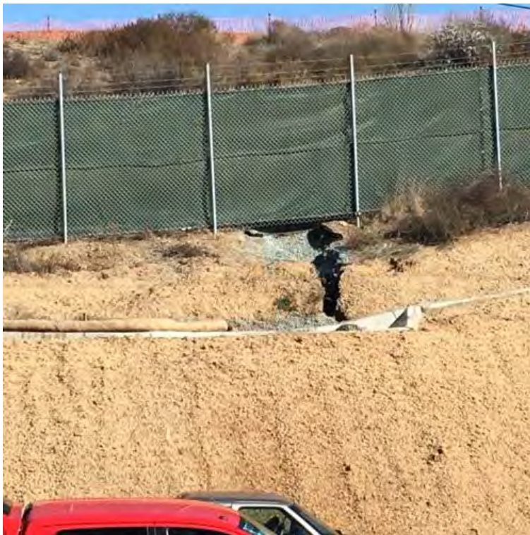
Caption Erosion along eastern fence line
