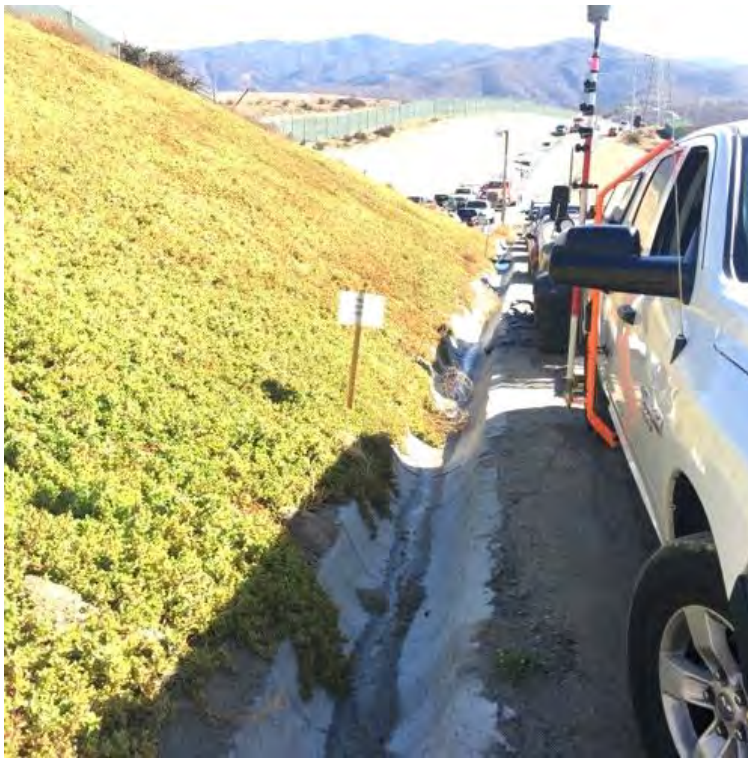
Caption Sediment in culvert
