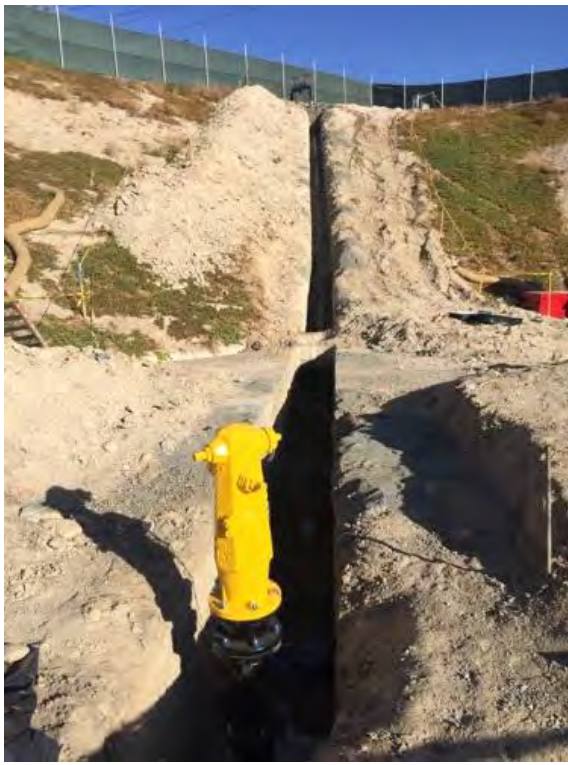
Caption Fire water line and new hydrant
