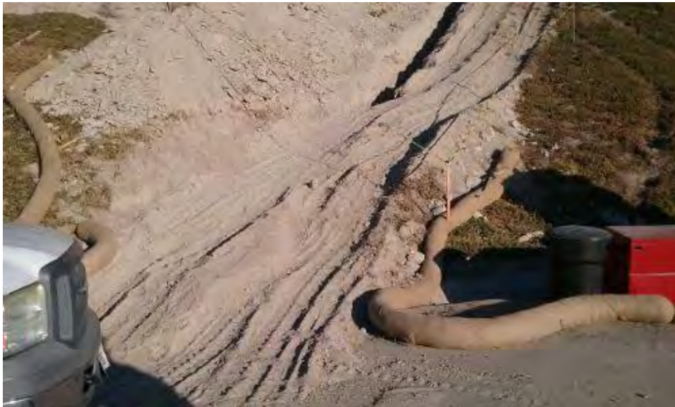
Caption Wattles moved to side ro provide temporary access for water line work.
