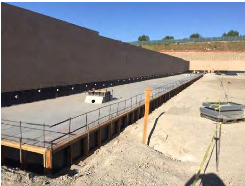
Caption Oil containment basin
