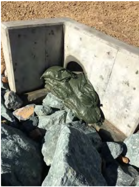
Caption Clean storm drain outlet
