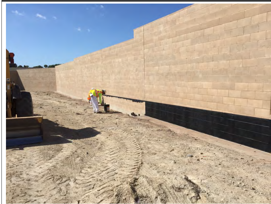
Photograph 2: Application of water proofing on masonry walls occurred during the week of October 31, 2016.
