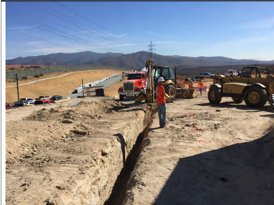
Photograph 1: Excavation of trenches for 12 kV conduit occurred during the week of November 7, 2016.
