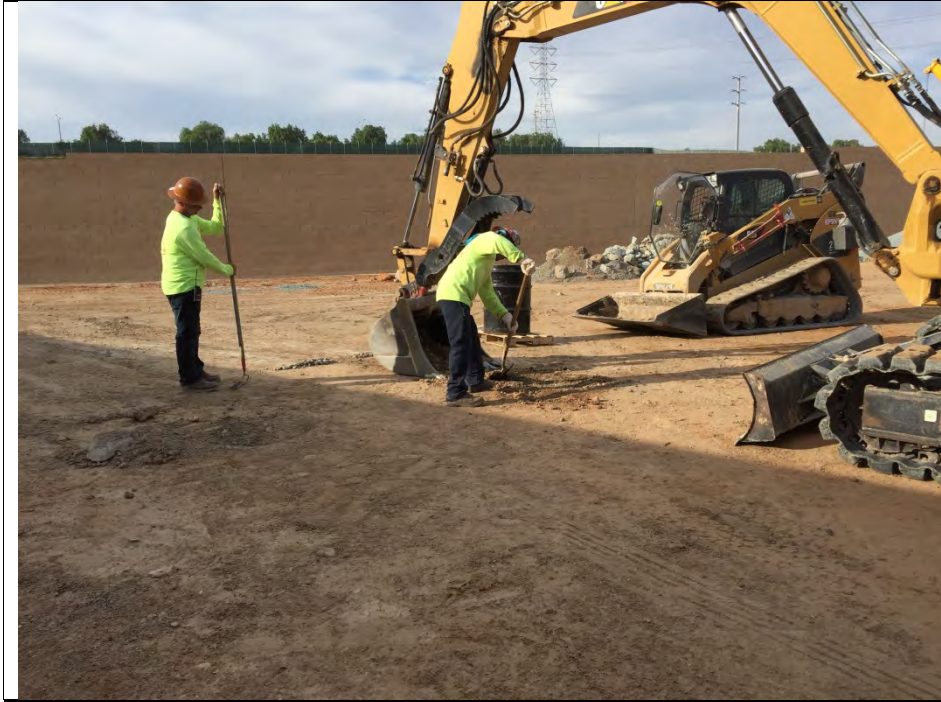
Photograph 3: Geo Pacific construction crew cleaning up hydraulic fluid spill that occurred on November 15, 2016.
