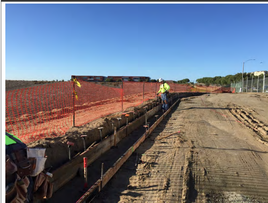
Photograph 2: Construction of the curb and gutter along Road A occurred during the week of November 21, 2016.
