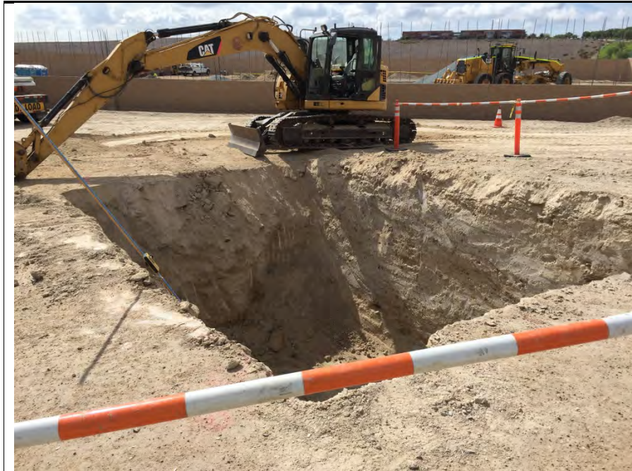
Photograph 1: Excavation of holes for 12 kV vaults occurred during the week of October 31, 2016.
