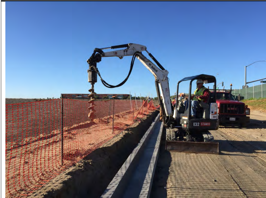
Photograph 1: Installation of fencing along Road A occurred during the week of November 21, 2016.
