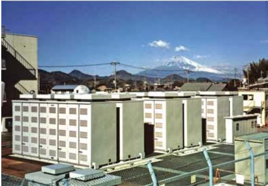
The NAS battery installation at Tokyo Electric Power Co.'s Ohito Substation is rated at 6 MW/48 MWh
