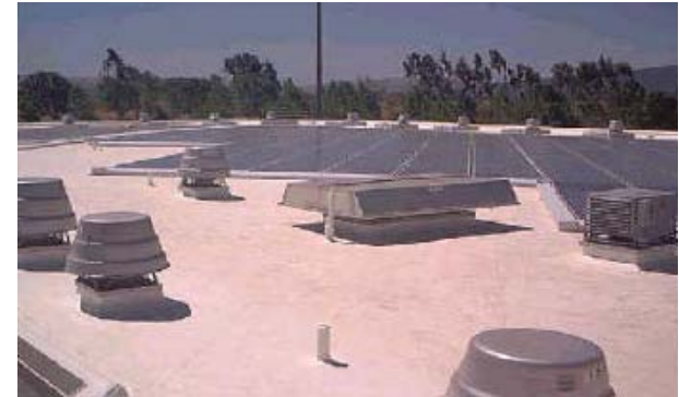
1.5 MW solar installation
