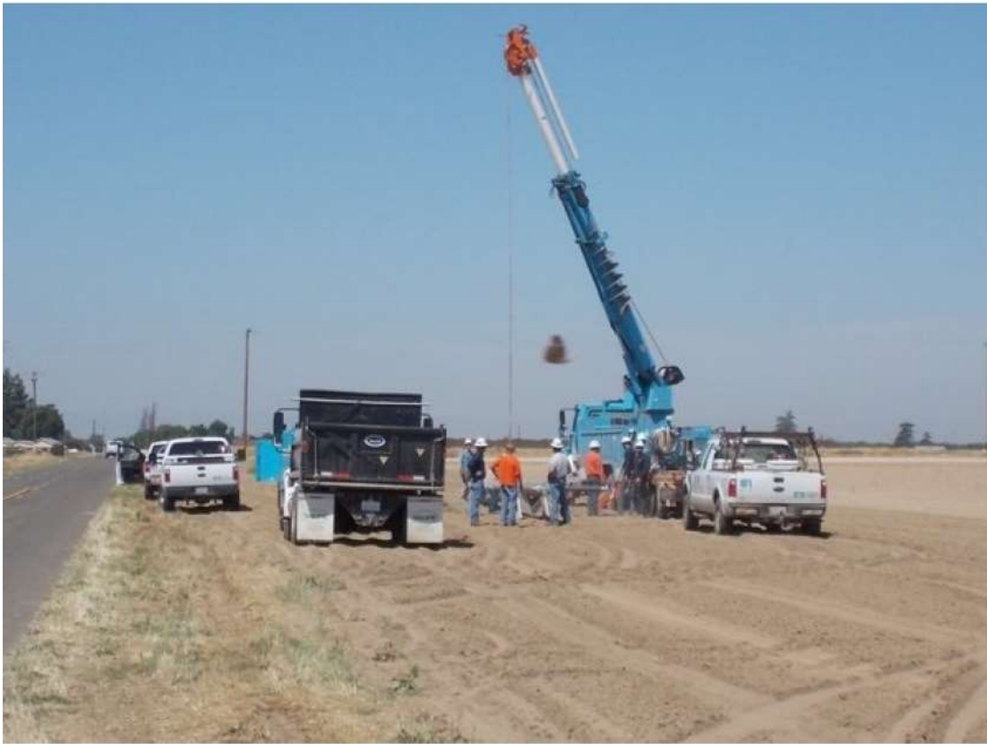
Figure 3 – Crews installed poles along Magnolia Avenue during the subject period. View west (Photograph provided by PG&E).
