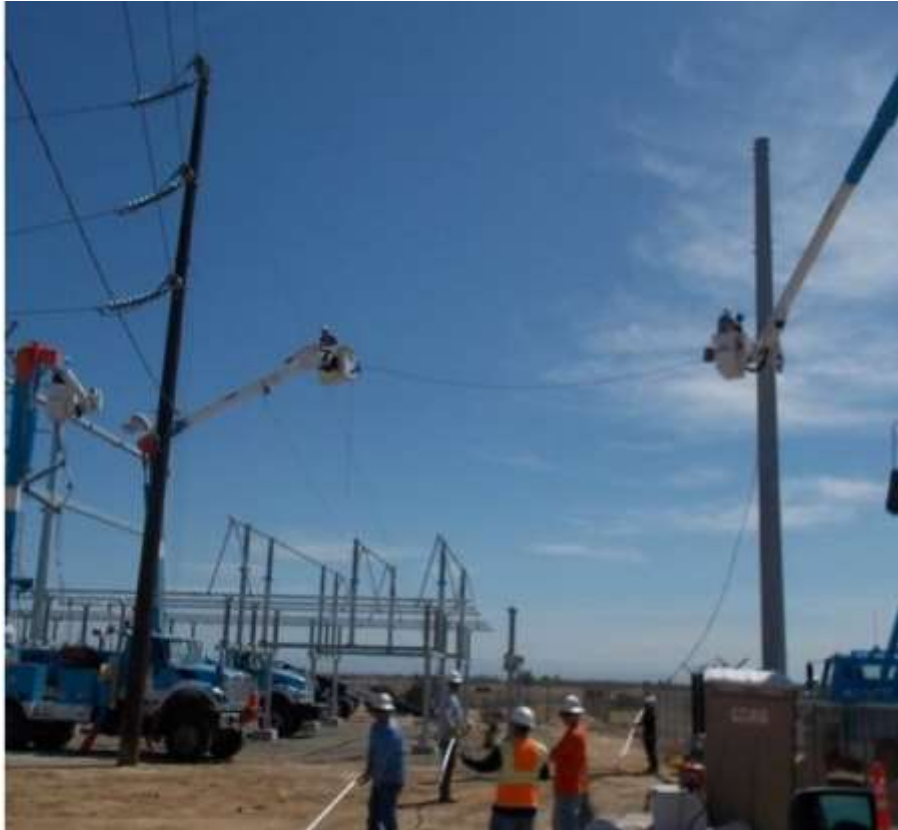
Figure 1 – Structure installation continued at the Cressey Substation during the subject period. View westward (Photograph provided by PG&E).
