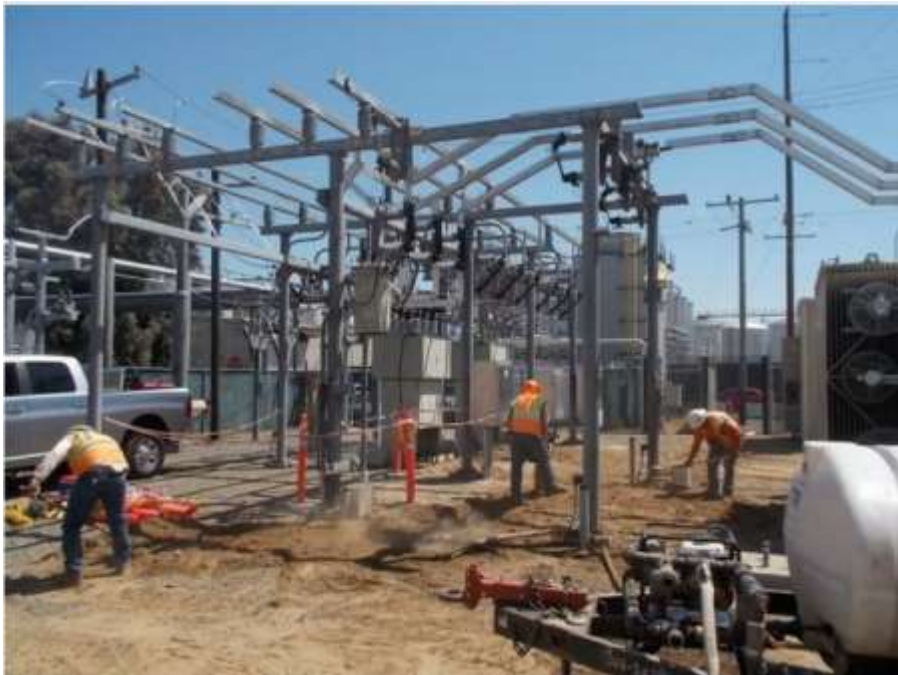
Figure 2 – Conduit installation continued at Gallo Substation during the subject period. View northeast (Photograph provided by PG&E).
