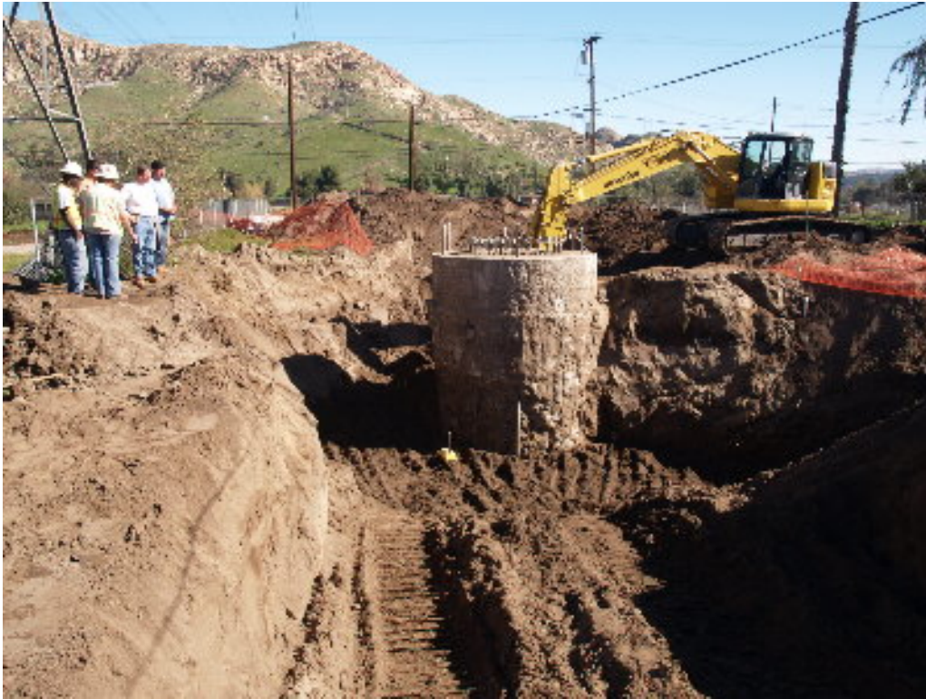
Figure 3 – The contractor worked on compaction at Tower Site 1210 after the foundation was exposed for inspection. The current foundation will be removed below grade and the entire operation repeated.
