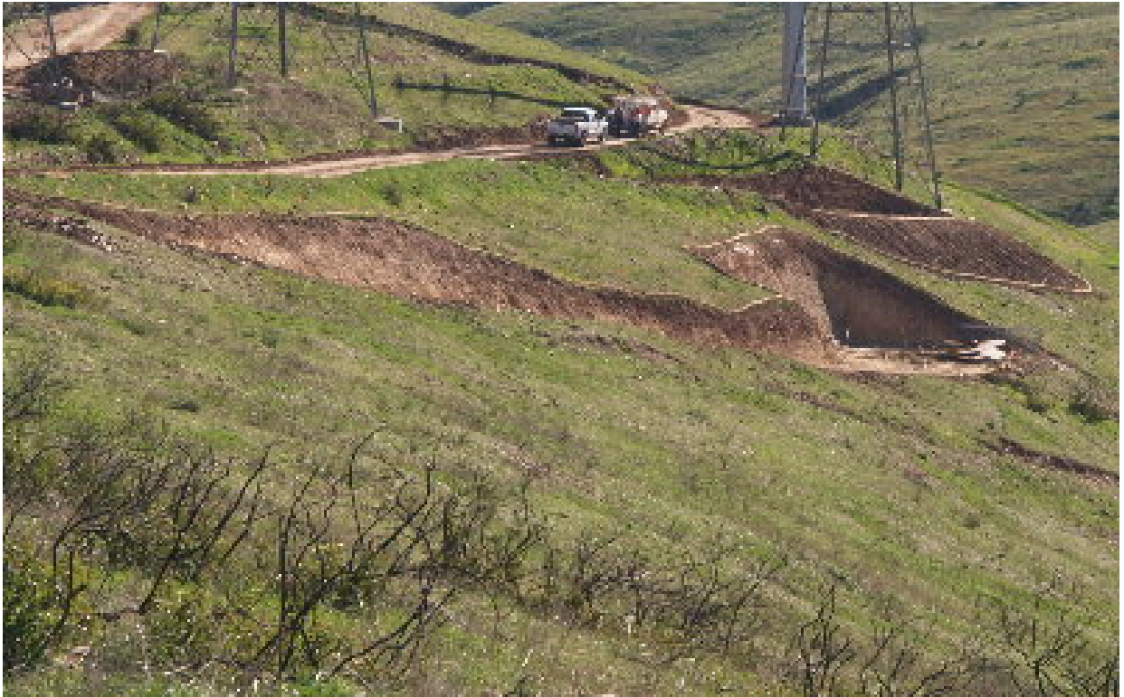
Figure 5 – Several of the straw waddles placed at Tower Site 601 cannot contain the material above or are installed at very steep angles.
