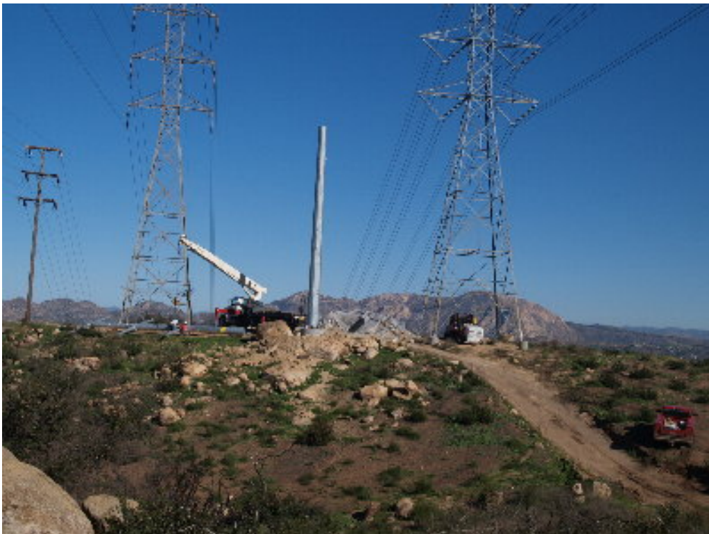
Figure 8 – The PAR crew attached the arms to the upper section of the steel pole. Note the red truck parked off the access road, in the habitat.
