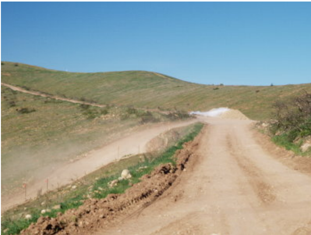
Figure 4 – Fugitive dust was observed leaving the right-of-way at Tower Site 601 during the site visit. The roads and spoil piles had not been watered recently.
