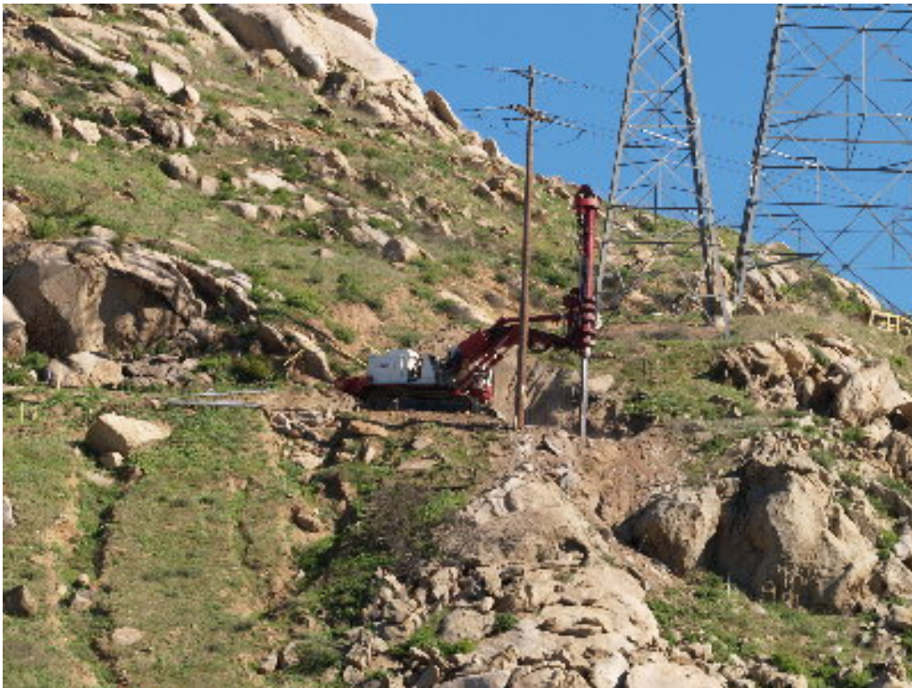
Figure 2 – The Low Drill continued work at Tower Site 1160. Note material moving down hillside under the drill.
