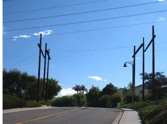
Figure 4-8. Guard structures placed across residential road to prevent pulling rope from sagging onto road, September 26, 2005
