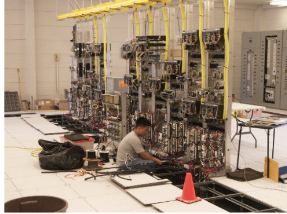
Figure 2-7. Crews worked inside MEER #1 on communication and control systems for the Viejo Substation, March 20, 2005
