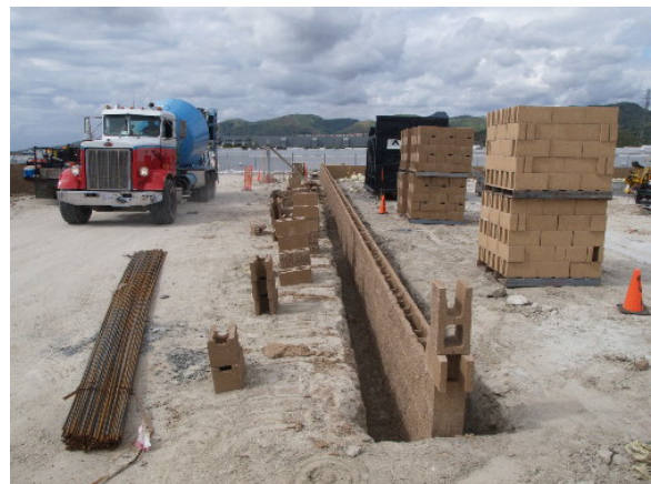
Figure 2-8. Reycon Construction crews built the containment walls and the block wall surrounding the Viejo Substation after the foundations were placed by Union Construction, March 22, 2005
