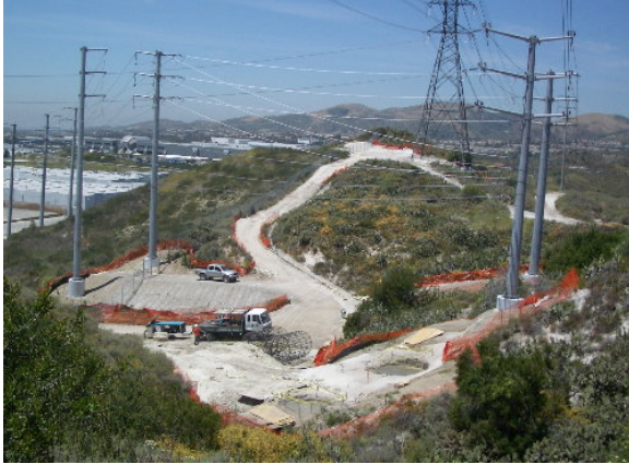
Figure 4-3. The two excavations for H-Frame Structure 13 in the foreground were backfilled with slurry after improper placement, May 20, 2005. Note the contrast compared to Figure 4-1.
