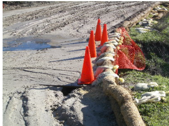
Figure 3-8. Heavy rains and the use of inappropriate erosion prevention and sediment control devices led to sediment transport on the 220 kV transmission line right-of-way, December 30, 2004
