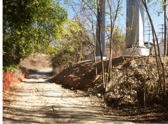
Figure 4-10. No recruitment of native (or ruderal) vegetation has been observed on the disturbed slope below H-Frame Structure 1, October 31, 2005
