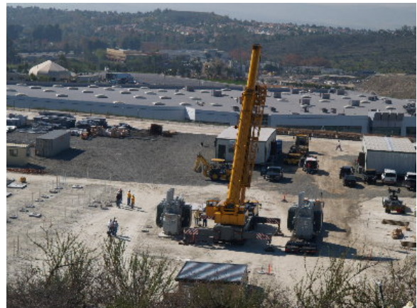
Figure 2-6. Large crane brought to Viejo Substation to set B-bank transformers onto completed concrete pads, November 18, 2004
