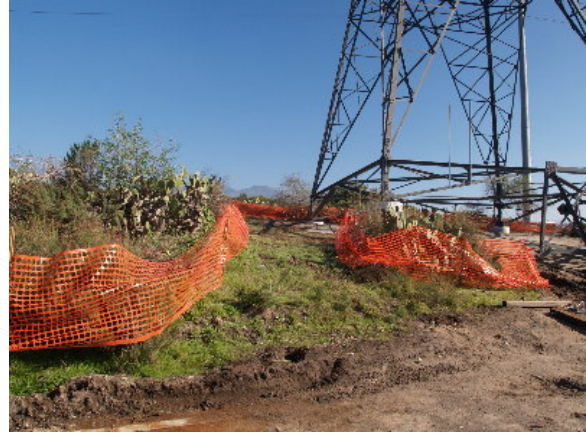
Figure 3-2. Higher value native habitat was marked off to allow the crane and man-lifts to set up on the southern 220 kV tower, December 9, 2004
