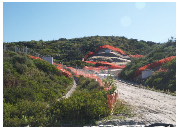
Figure 4-2. New access roads and pads were required for the steel poles connecting the 66 kV right-of-way and the Viejo Substation, April 1, 2005
