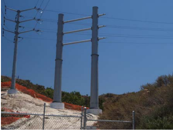
Figure 4-7. H-Frame Structure 13 completed with cross members and west set of arms, June 22, 2005
