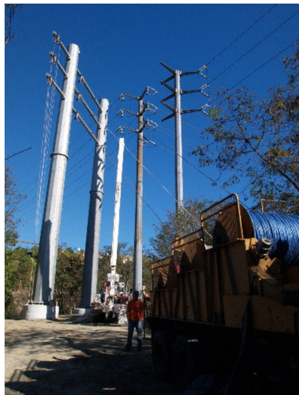
Figure 4-9. The pulling crew set up adjacent to the Chiquita Substation to pull the center circuit of the 66 kV transmission line, April 1, 2005
