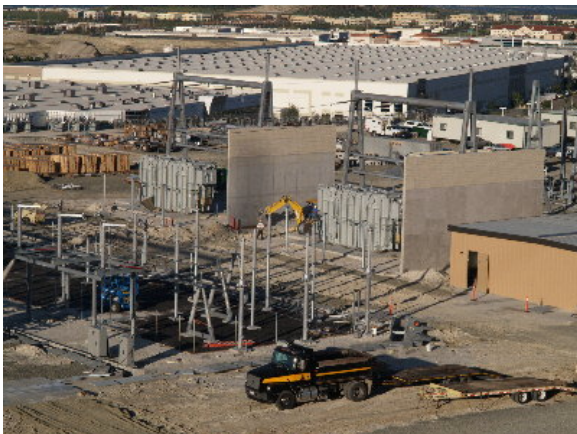
Figure 2-5. Firewalls constructed between the two A-bank transformers and between the transformers and MEER #1, January 11, 2005
