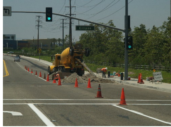
Figure 2-10. Arizona Pipeline installed the 12 kV distribution system and the fiber optic communication lines between the Viejo Substation and the local system, May 24, 2005
