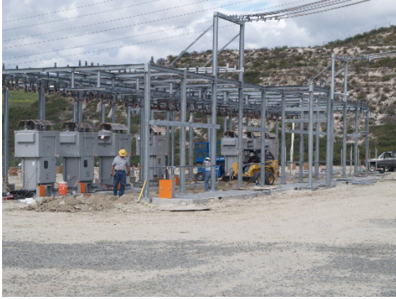
Figure 2-9. The substation electrical contractor, NRG, worked on the 12 kV switching system, March 22, 2005
