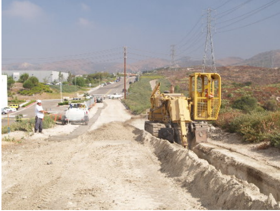
Figure 2-3. Three Kings Construction excavates trench along main access road for fiber optic and 12 kV distribution lines, August 4, 2004
