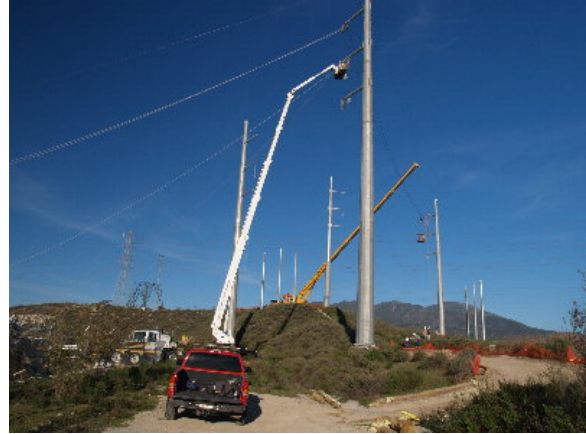
Figure 3-5. Crews used man-lifts and crane-supported baskets during stringing activities on the 220 kV section, December 17, 2004
