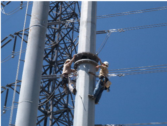
Figure 4-5. A crew scaled H-Frame Structure 12 to guide the upper section into place and bolt it to the lower section, June 7, 2005
