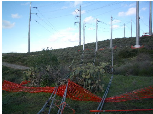
Figure 3-6. Conductor dropped during the stringing of the 220 kV transmission line. SCE worked with the project biologist to remove the conductor with minimal environmental impact, December 30, 2004
