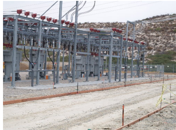
Figure 2-11. The 12 kV underground distribution conductor was connected to the switching system at the Viejo Substation, July 20, 2005
