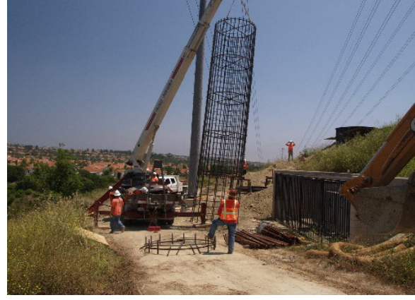
Figure 4-4. Crews prepared to lower the rebar re-enforcing cage and anchor bolts into the foundation for H-Frame Structure 9 prior to concrete placement, June 14, 2005
