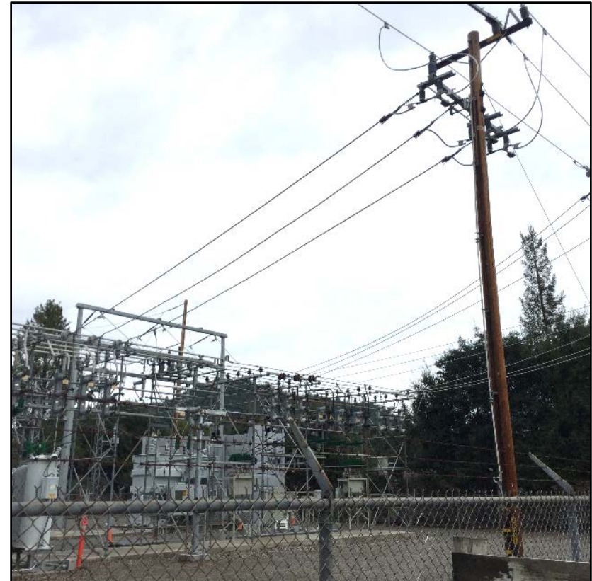
Fitch Mountain Substation
