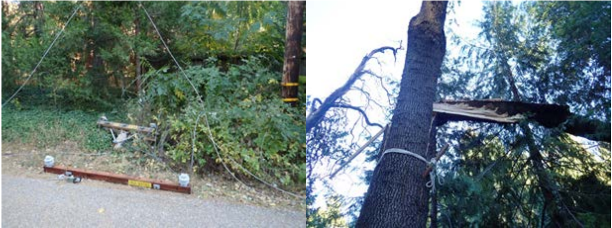
Figure 1. Foresthill, Placer County. Pole, cross-arm and conductor damaged by split tree.
