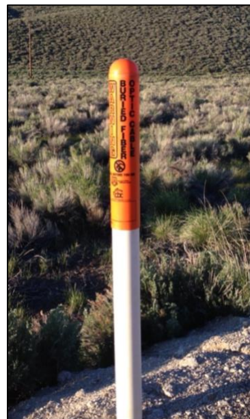
Figure 2 — A marker for a CPUC-funded fiber line in Mono County.
