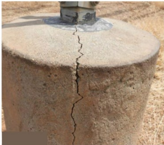
>1/16" crack reaching stub
