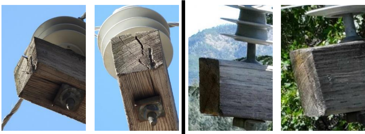
Figure 16: This condition was not identified by PG&E aerial inspections. Left: Photos taken during ground inspections show damage to the crossarm. Right: The crossarm damage is difficult to see from aerial photographs.
