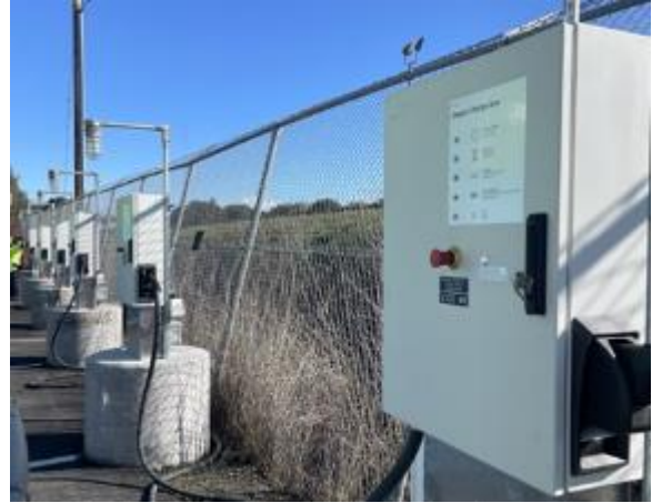
Figure 83. PG&E EV Fleet Program Sequential DCFC Dispensers
