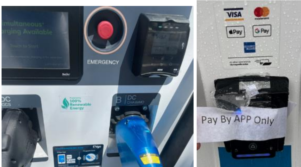
Figure 118. PG&E EV Fast Charge Program Examples of Newly Required Credit Card Readers for EY2022
