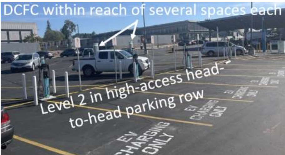
Figure 177. SDG&E Schools and Parks Pilots Community College L2 and DCFC Installation with High Access
