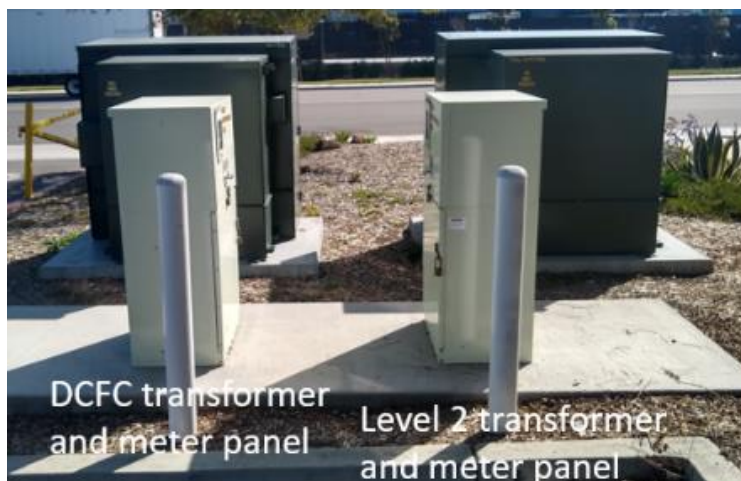
Figure 181. SDG&E Schools and Parks Pilots Site with Separate Meter Cabinets for Different Voltages for DCFC and L2 Chargers
