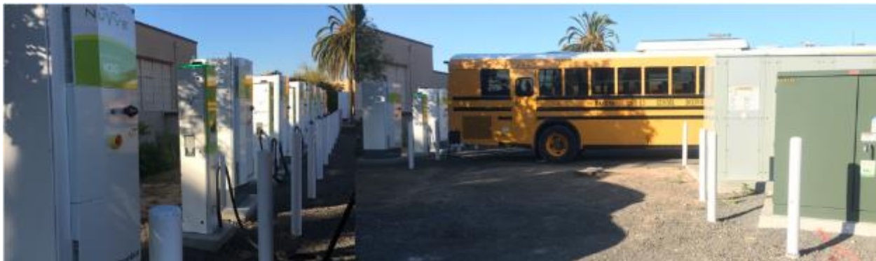
Figure 149. Example of Charging Infrastructure Installed Exclusively in Softscape
