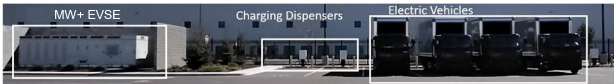
Figure 75. PG&E EV Fleet Program Layout of the First Site with Megawatt EVSE
