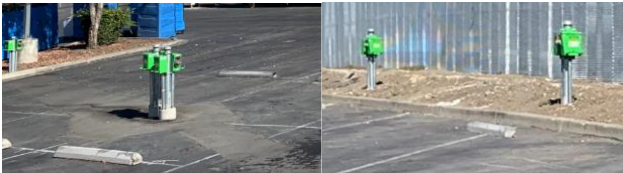
Figure 79. PG&E EV Fleet Program Example eTRU Ports
