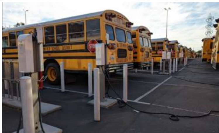
Figure 142. Centrally Placed EV Chargers that Maximize
