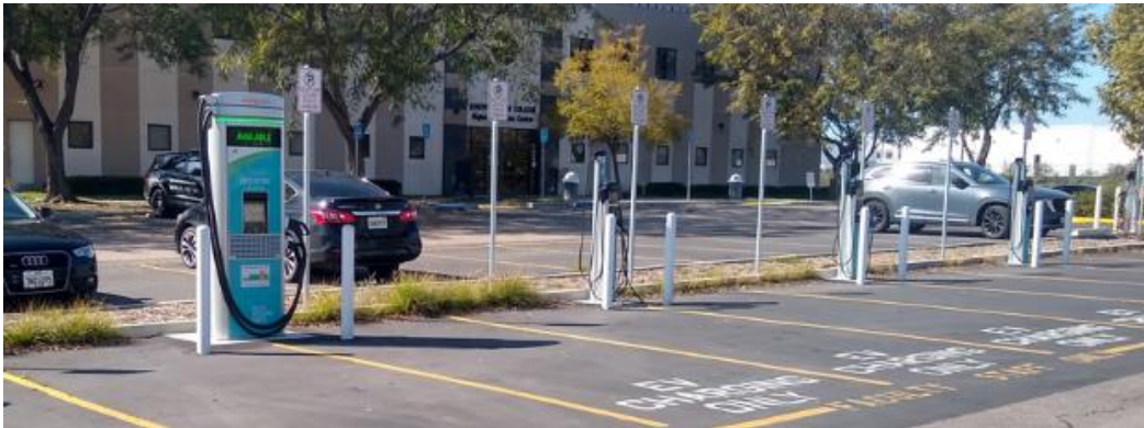
Figure 179. SDG&E Schools and Parks Pilots Examples of DCFC and L2 EVSE with Very High Access to Parking Spaces
