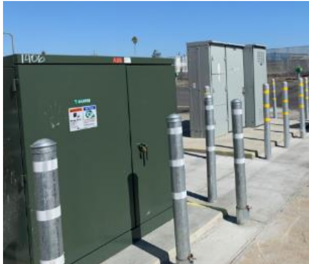
Figure 84. PG&E EV Fleet Program Electrical Equipment Can Take Up Valuable Real Estate
