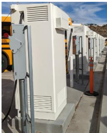
Figure 150. Mid-Parking Lot Installation of Dual Port DCFC Requiring Cement Work and Repair
