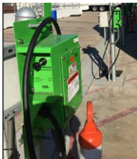
Figure 19. Electric Truck Refrigeration Unit Connector
