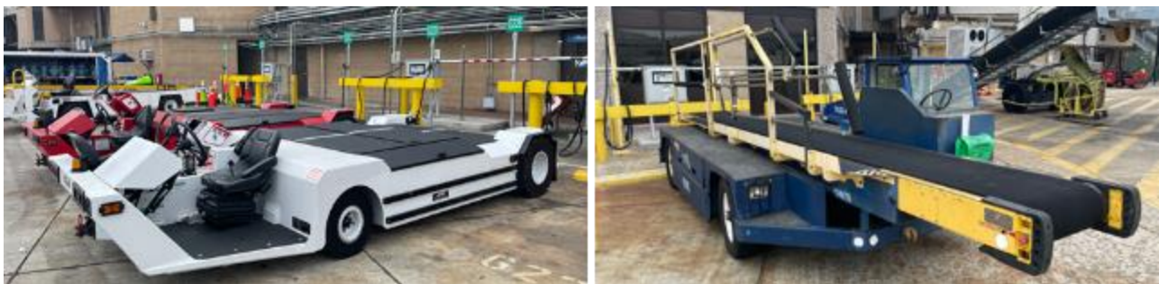
Figure 147. Conduit Runs to Electrical Rooms and GSE Charging (push back tractor and belt loader)
