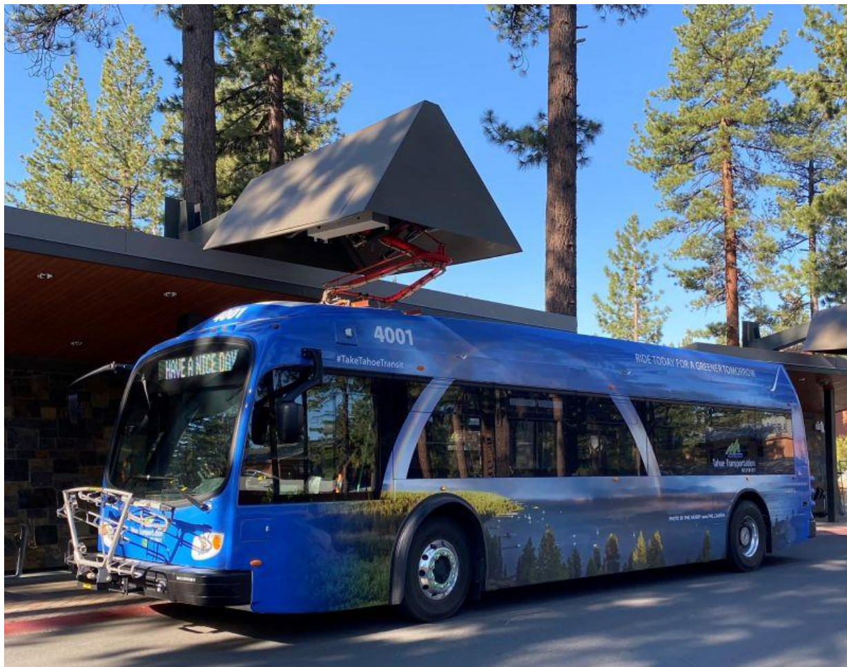
Figure 199. TTD’s Proterra Electric Bus Charging on the 450 kW ABB Pantograph at LTCC
