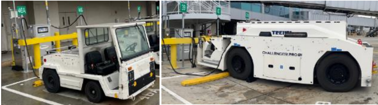
Figure 148. Complex Airport GSE Charging Installation (baggage tractor and push back tractor)
