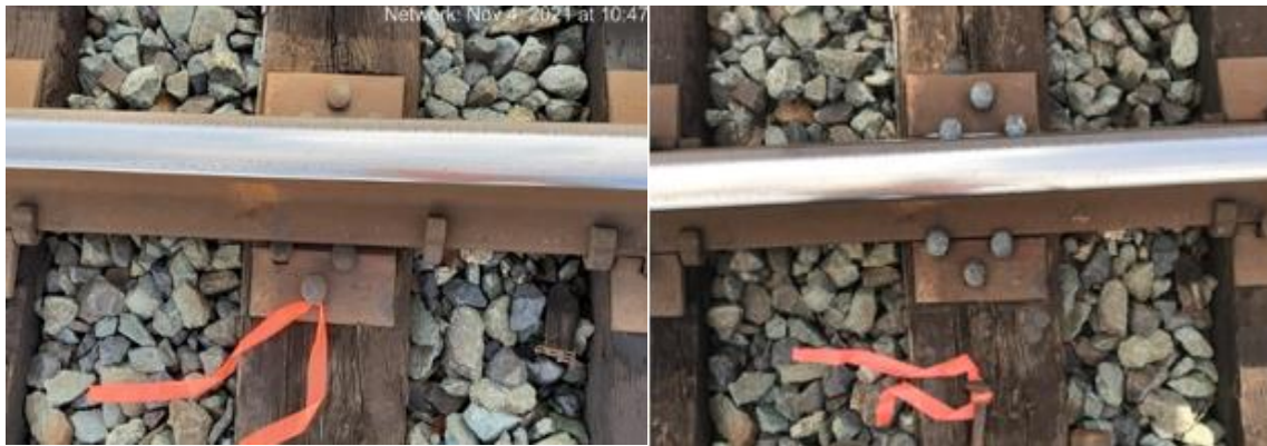
Before: Spikes under the rail causing a load-bearing defect After: Defect corrected. Spikes properly placed
