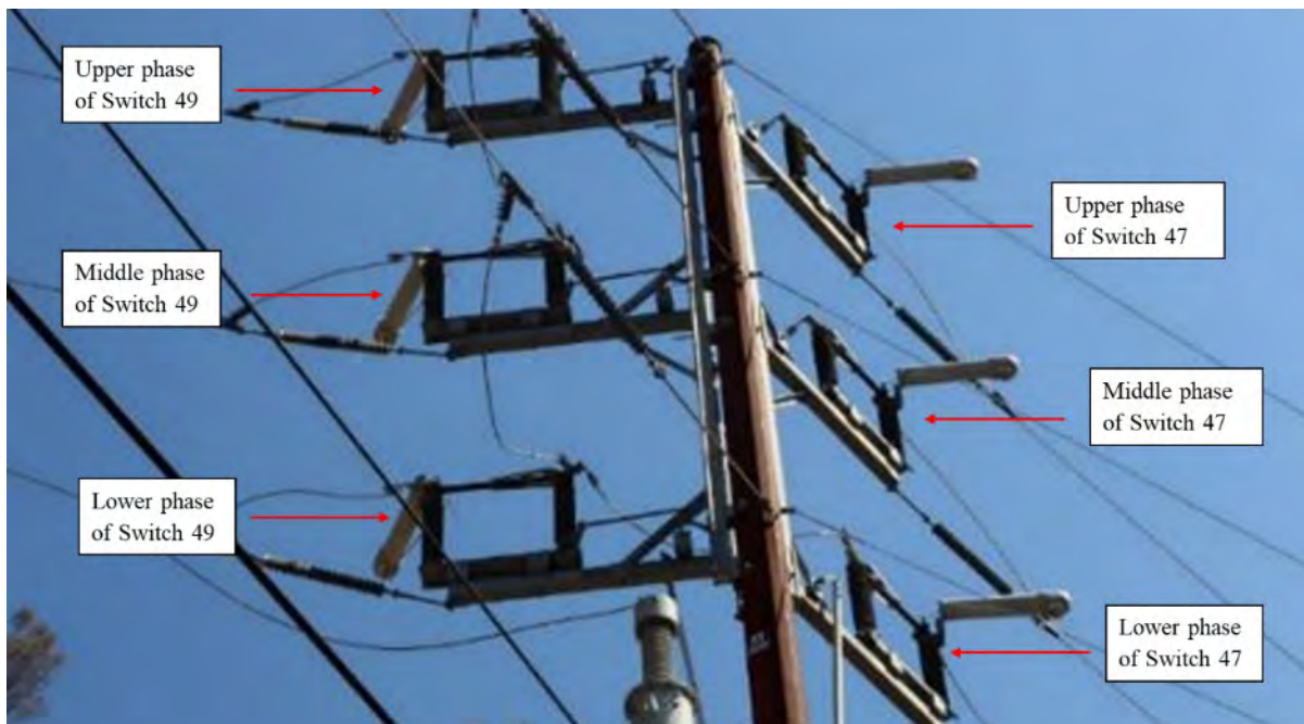
Figure 4: Switches 47 and 49 on Oxbow Junction Pole 33
