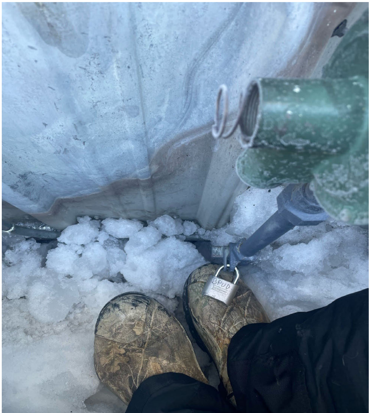
Photograph 2: Locked service valve and damaged regulator on Bridgeport NAPA Auto Parts Store gas riser (photo provided by the Bridgeport fire department)
