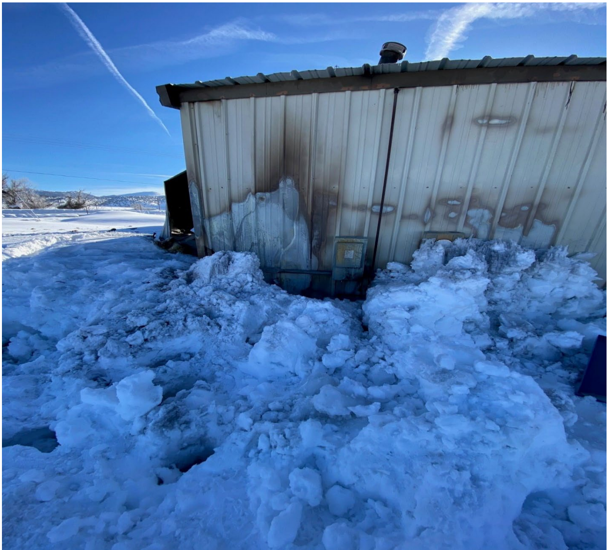
Photograph 1: Fire damage to Bridgeport NAPA Auto Parts Store (photo provided by Bridgeport Fire Department)
