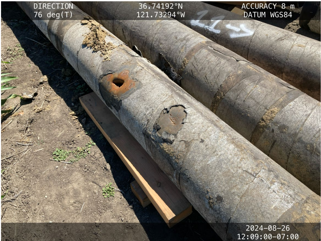
Figure 4. Photo of the impact site after the pipe was removed
