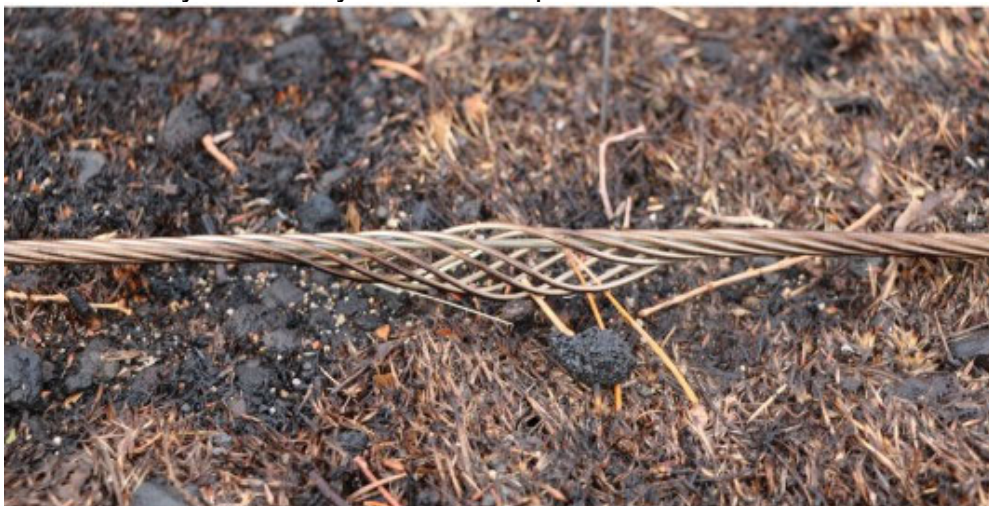
Figure 6: Conductor burned and visible bird-caging. 38
