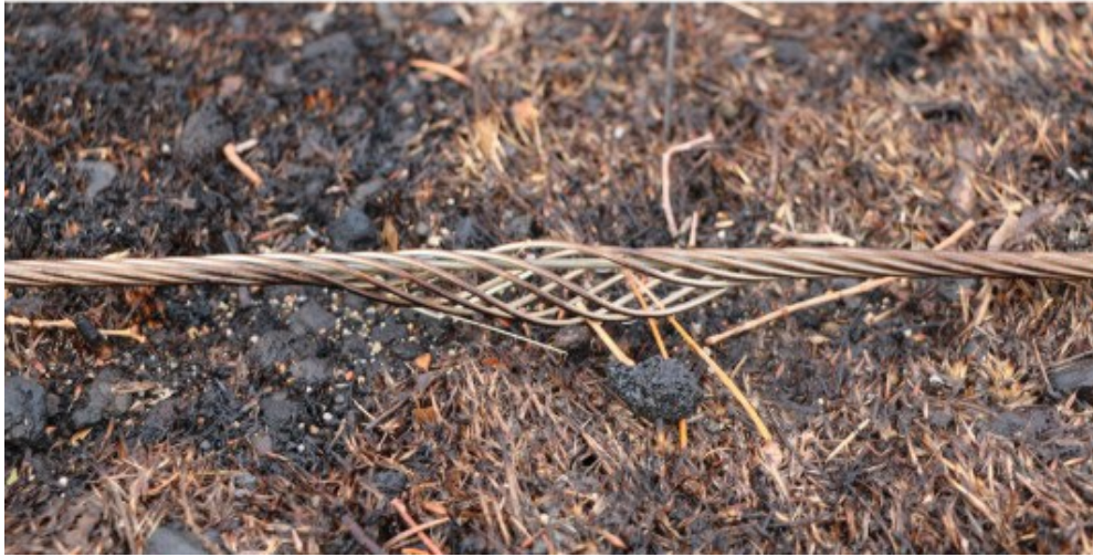
Figure 6: Conductor burned and visible bird-caging. 11
