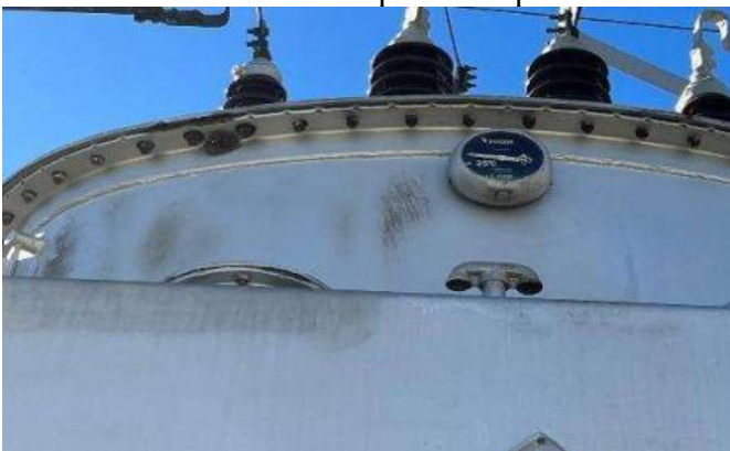
2.5 Transformer Bank 1C Wasp Nest Top Front – Fixed in Field
