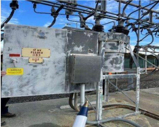
9.16 Under Ground Equipment Box Cover Near CB 1104/2 Was Loose and Not Secured - Leveled and Secured In Field
