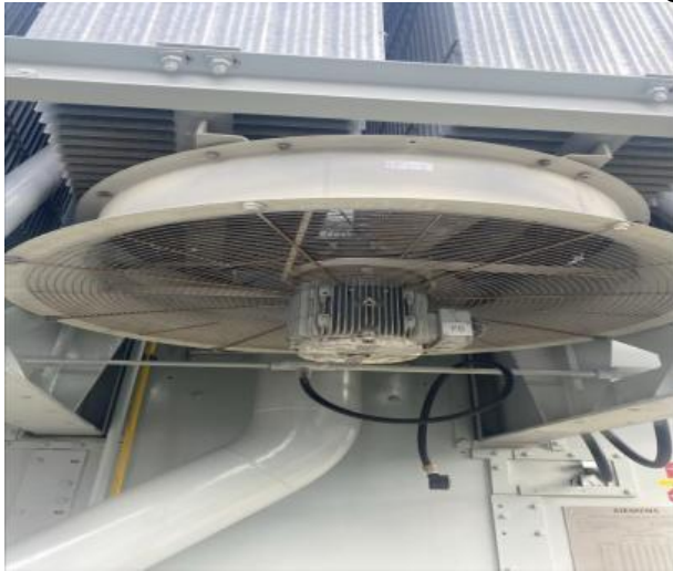
13.5 Transformer Bank 1 One Fan Not Working Existing LC Tag#131702282
