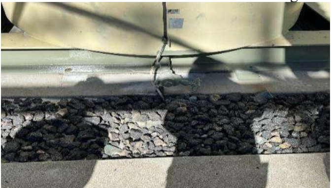
1.6 Circuit Breaker 400 B Phase Oil Leak Existing LC Tag#131966608
