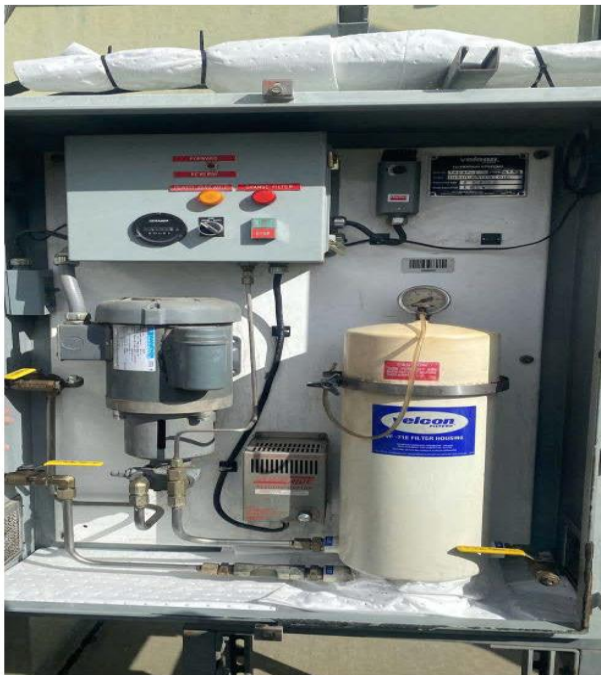
9.11 Transformer Bank 5 Oil Leak Mitigation Existing LC Tag#131966349
