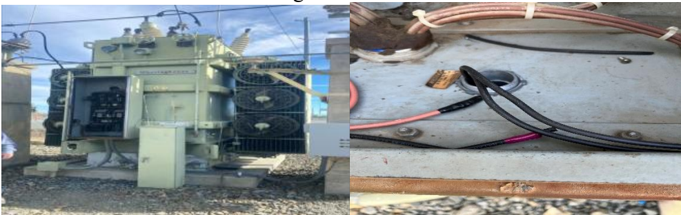
5.8 Transformer Bank 1C Missing Sealant For Conduit In Main Cabinet – Fixed In Field
