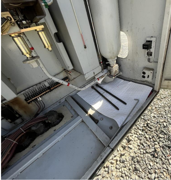
1.3 Circuit Breaker 500 B Sample Valve Oil Leak Existing LC Tag#131965860
