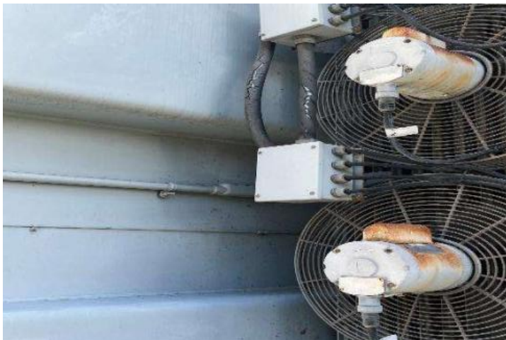
12.1 Transformer Bank 1 Fan Conduit Faded and Cracked Existing LC Tag#131966631
