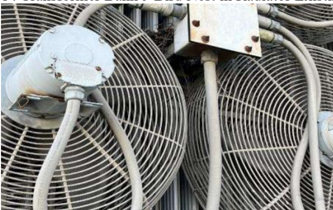
5.15 Transformer Bank 10 Bird Nest in Radiator Existing LC Tag#130927116
