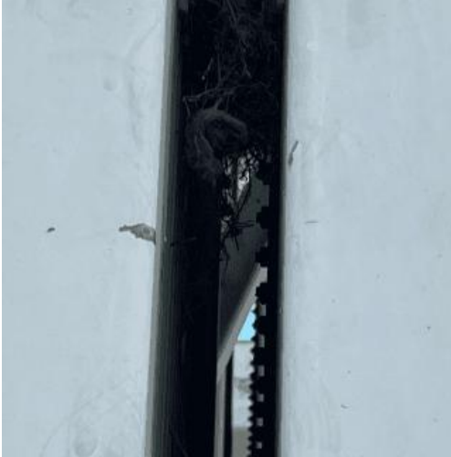
14.8 Transformer Bank 2 Bird Droppings Existing LC Tag#131966309
