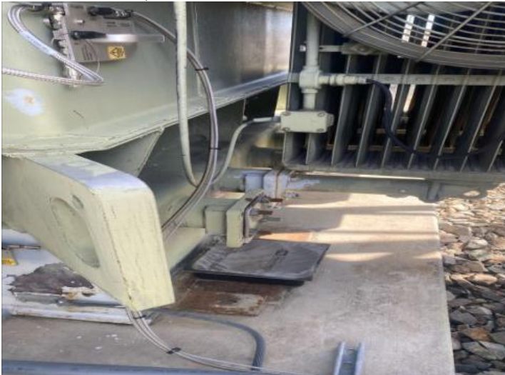
5.5 Transformer Banks 1A, 1B & 1C Oil Leak Mitigation Existing Tags LC#131966024, LC#131966026, & LC#131966029. Photo Below is Bank 1C
