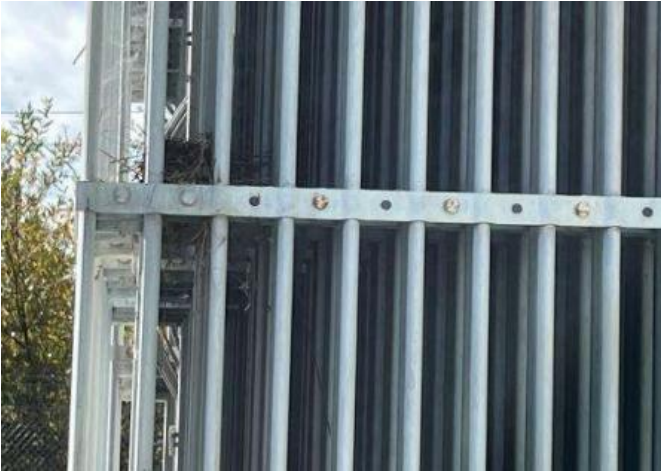
9.5 Transformer Bank 3 Birds Nest In Radiator Existing LC Tag#131966340
