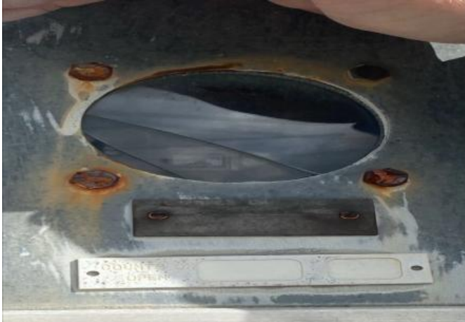
9.15 Circuit Breaker 1103/2- Oil Mitigation and Cleanup Existing LC Tag#131966446
