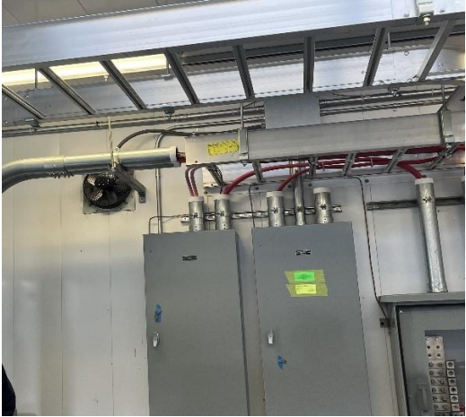
15.2 Circuit Breaker 1232 Birds Nest Existing LC Tag#131961605 and Station Birds Nest Existing LC Tag#131990024
