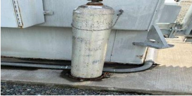
9.4 Transformer Bank 2 Loose Strap for Nitrogen Bottle Add to Existing LC Tag#131966289 on Nitrogen System
