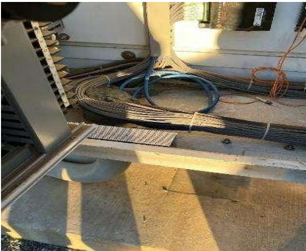
4.5 Transformer Bank 2 Two Conduits in Cabinet Missing Sealant Around Cables – Fixed In Field
