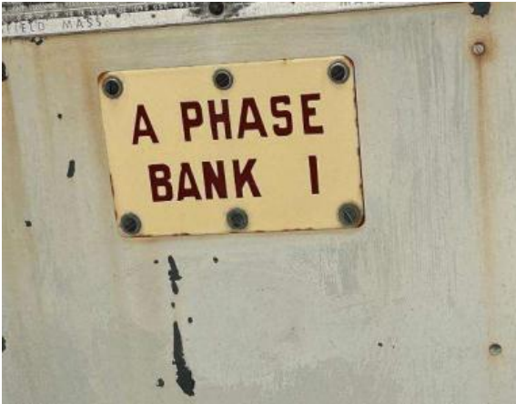
14.5 Transformer Bank 1 B Phase Birds Nest Existing LC Tag#131966301
