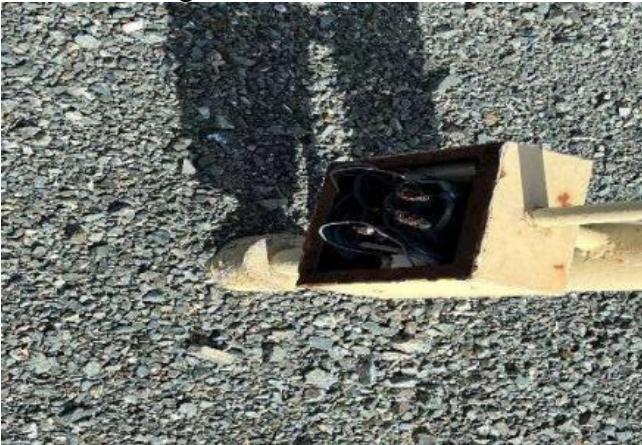
5.17 Substation Yard Light has Exposed Electrical Junction Box Between Transformer Banks 2 and 3 LC Tag#131966285
