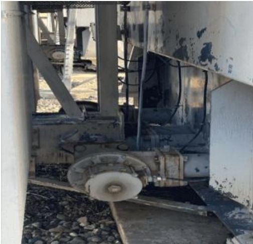
14.7 Transformer Bank 1 Spare Birds Nest in Radiator Existing LC Tag#131984277, Oil Mitigation LC 131966305, Fans Not Working LC 131987155
