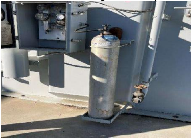
5.14 Transformer Bank 9 Bird Nest in Radiator Existing LC Tag#130927057
