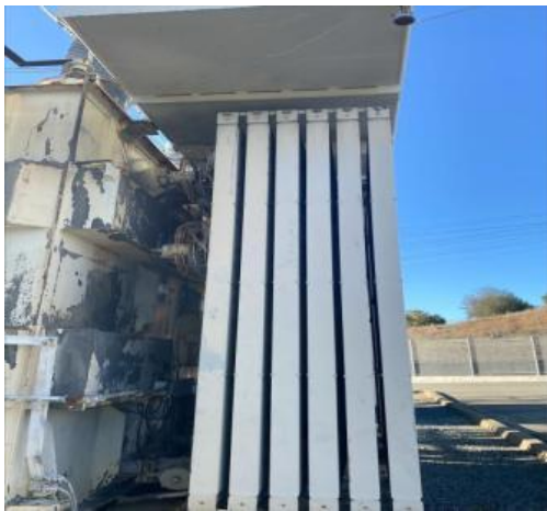
14.6 Transformer Bank 1 C Phase Fans and Oil Pump Not Working Existing LC Tag#13187150
