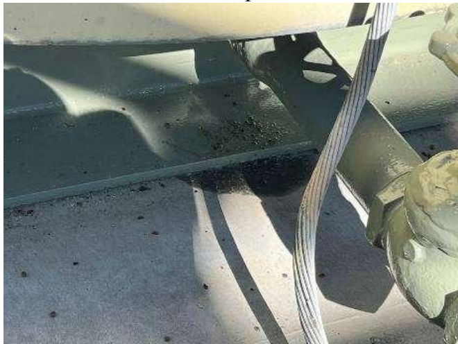
1.4 Bird Nest Near Circuit Breaker 500 Bus Work, Existing Station Bird's Nest LC Tag#131966674
