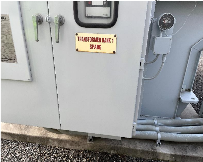
15.7 Transformer Bank 1 Spare Oil Mitigation Existing LC Tag#131990134
