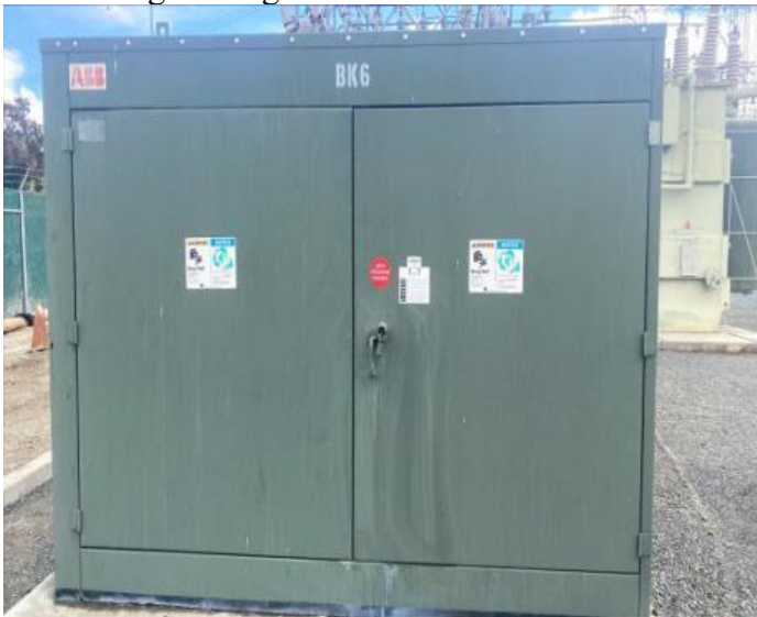
9.13 Transformer Bank 6 Live Front Auto Transformer, Did Not Open, Replace Oil Sample Valve Existing LC Tag#131195947
