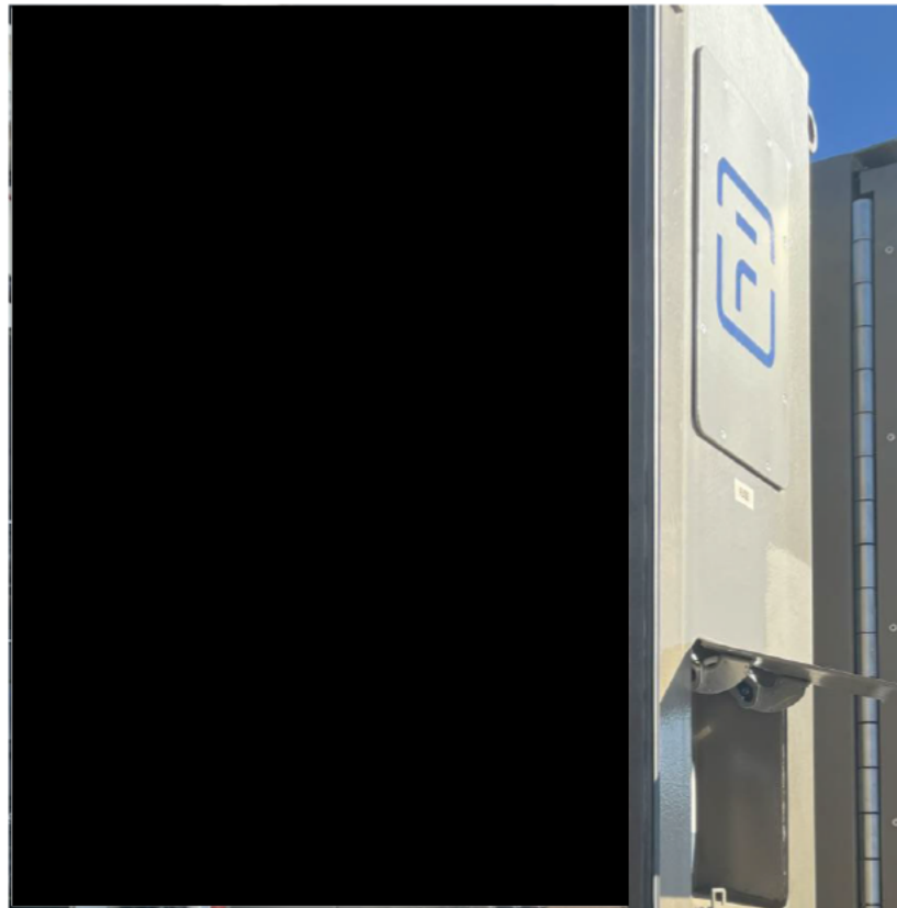
Figure 1: Fire Suppressant properly mounted in BESS cube
