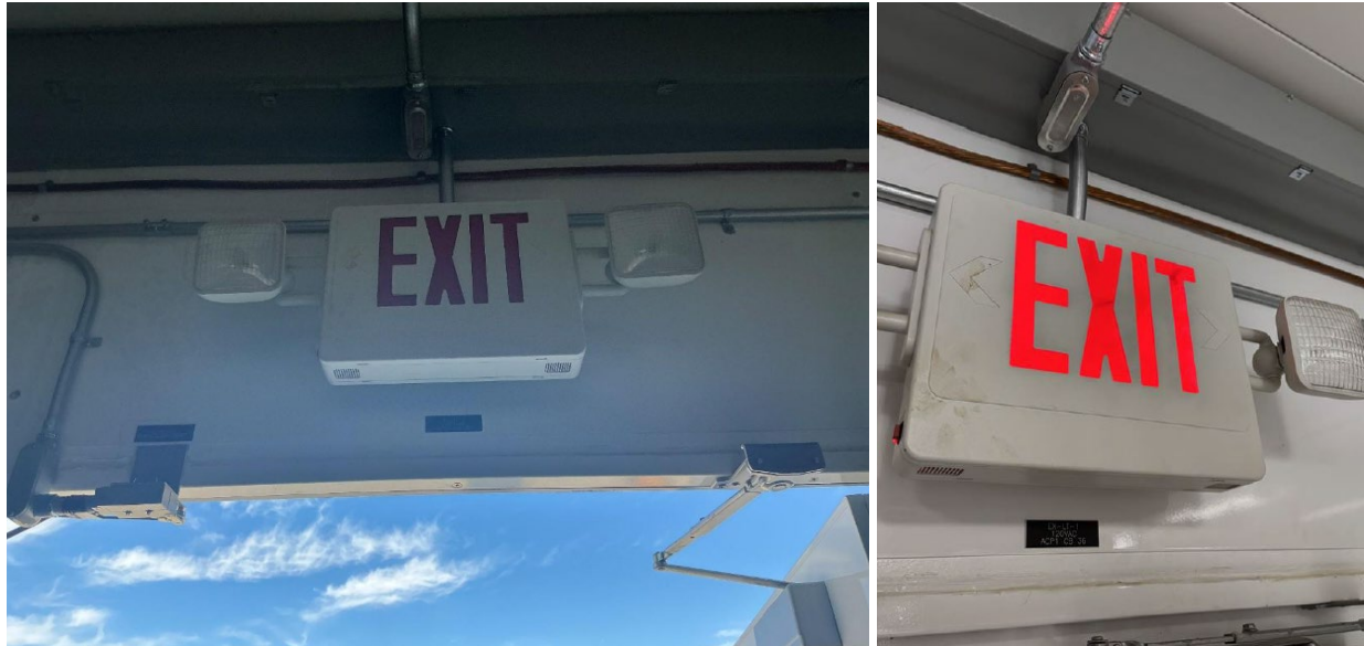
Figure 12: Non-functional exit sign in the substation control house(left). Repaired and functional exit sign (right).
