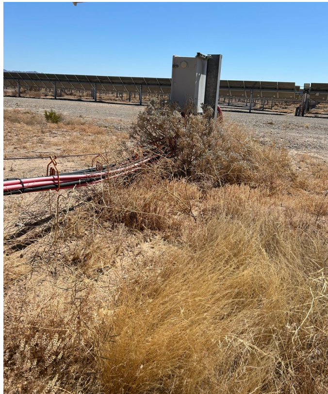
Figure 5: Overgrown vegetation around a combiner box.
