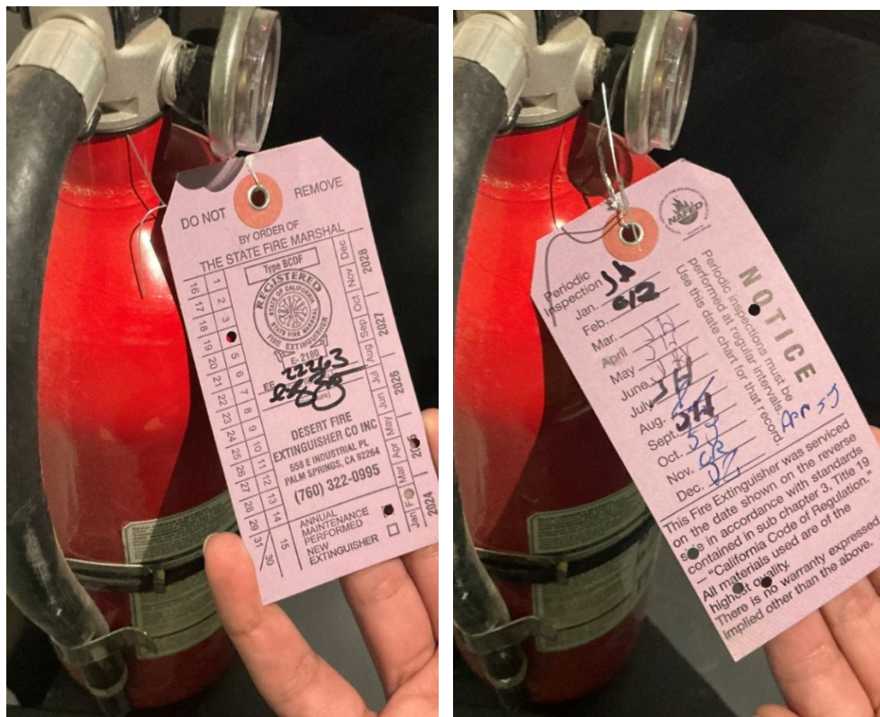
Figure 10: Fire extinguisher tag showing an outdated year, marked for 2025 but not 2026 (left). Reverse side of the tag showing a missed inspection for March 2025 (right).
