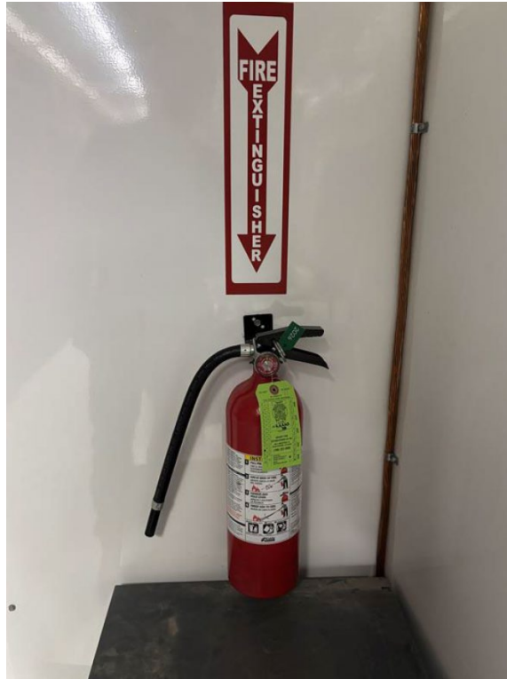
Figure 11: Inspected fire extinguisher in the Dracker Substation control house.
