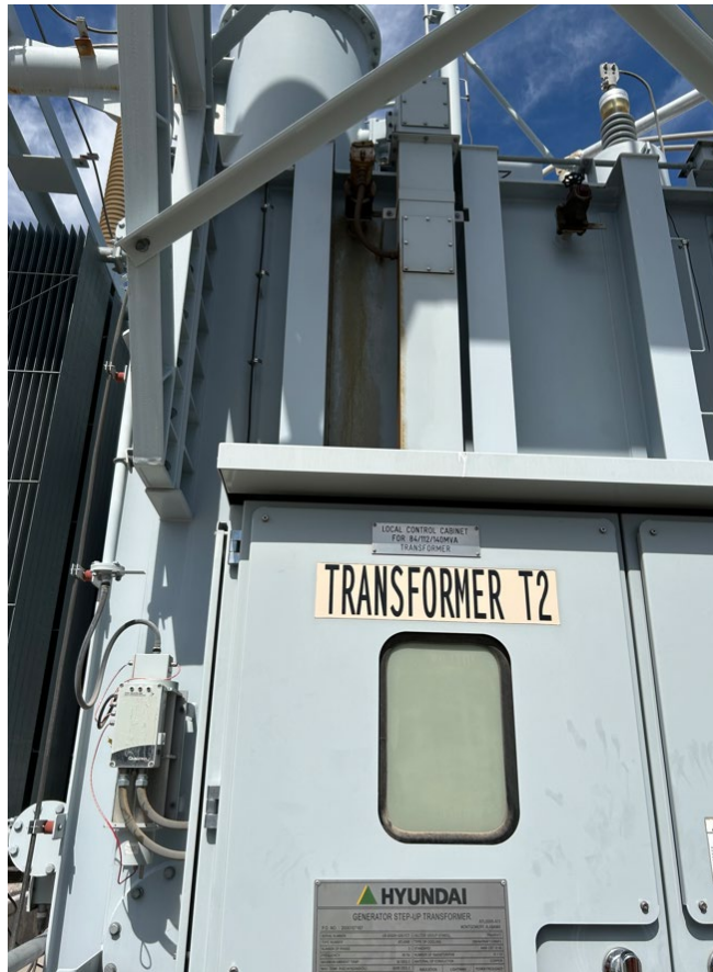
Figure 6: GSU Transformer T2 with evidence of an oil leak.
