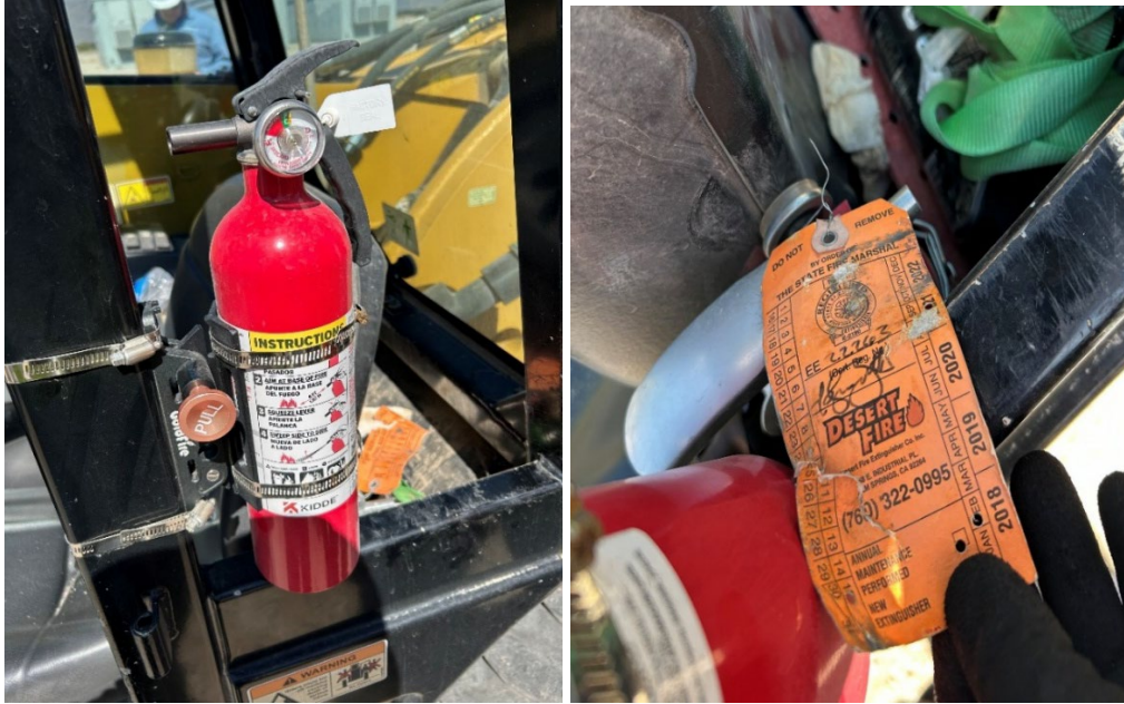
Figure 9: Fire extinguisher on forklift missing inspection tag (Left). Fire extinguisher on forklift with an outdated inspection tag showing last inspection in 2021 (Right).
