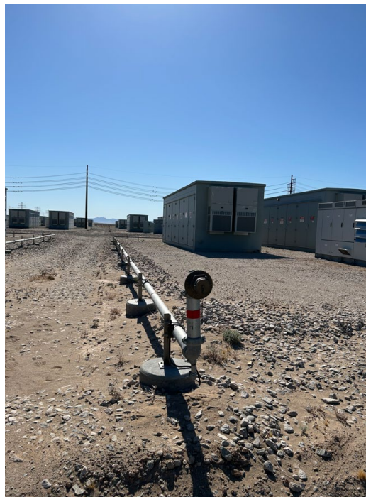
Figure 1: One of the FDCs for the Blythe Energy Storage II manual dry-type fire protection system.
