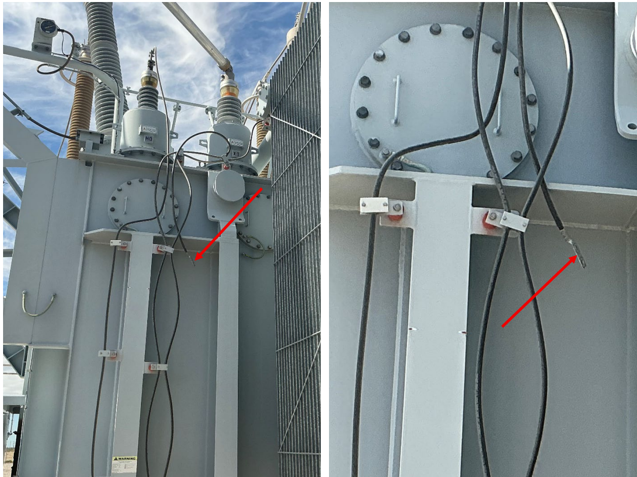
Figure 8: GSU for Blythe 1 with a dangling/disconnected ground wire (left). Close-up view of the dangling/disconnected ground wire (right).
