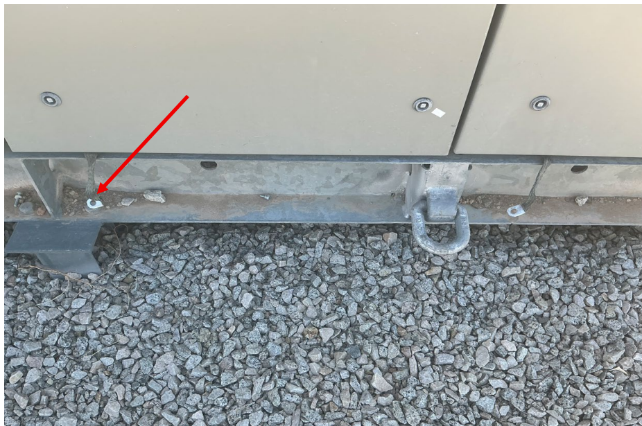
Figure 13: Disconnected grounding straps on the doors of multiple inverters
