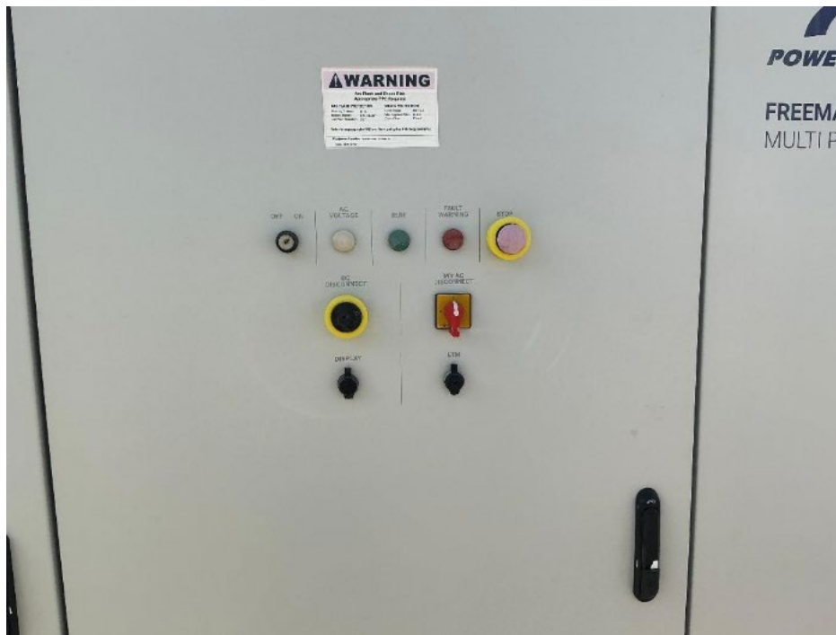
Figure 16: Status lights not operational on working equipment.
