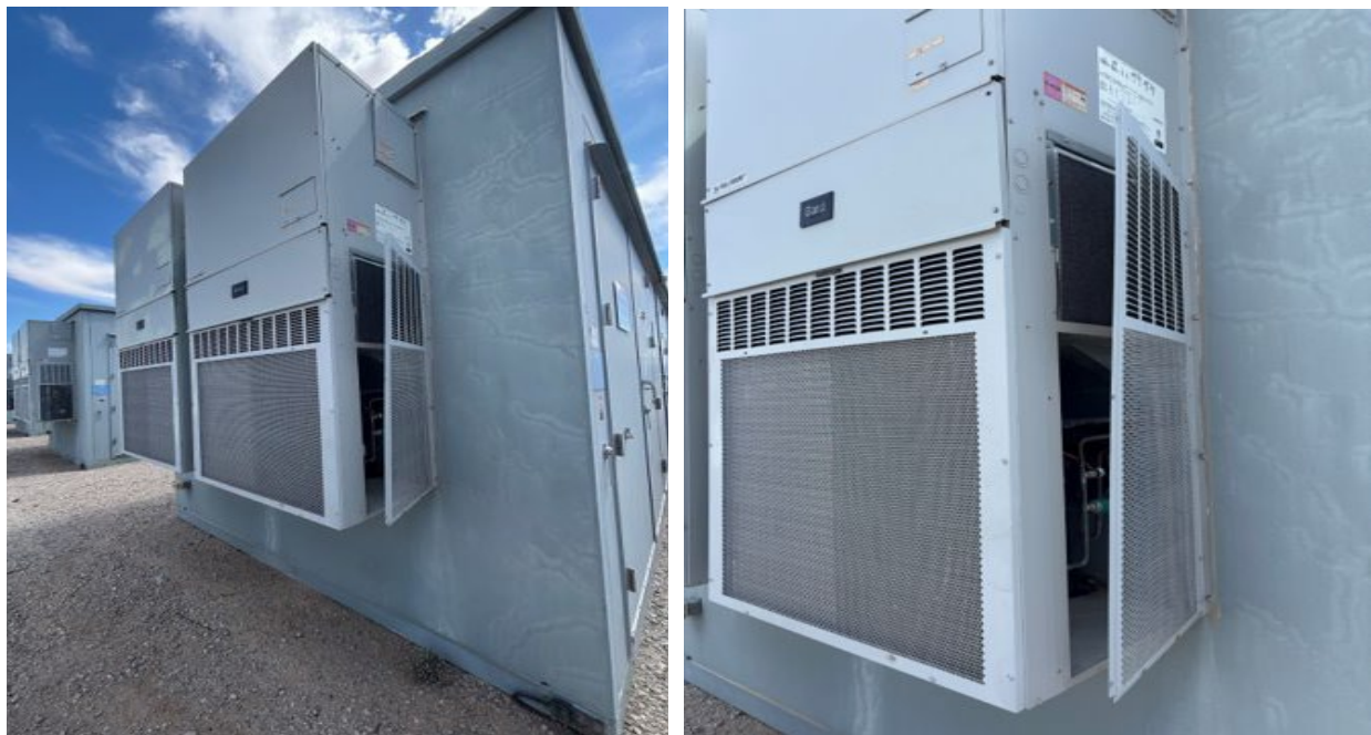
Figure 14: HVAC unit on Battery Unit BATT 18A-9A at Blythe Energy Storage III with unsecured cover panel (left). Close-up view of the unsecured HVAC cover panel (right).
