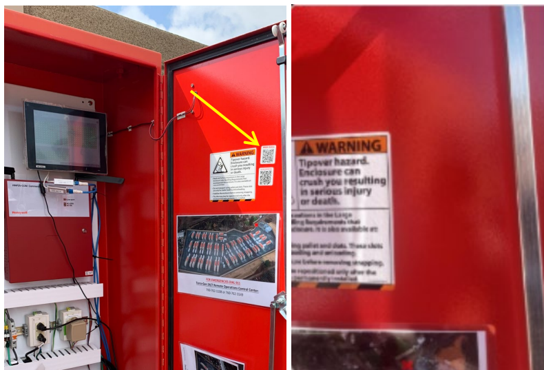
Figure 12: (Left) Pearce QR code posted on the FACP door. (Right) Valley Center removed the QR code from the FACP door during the audit.
