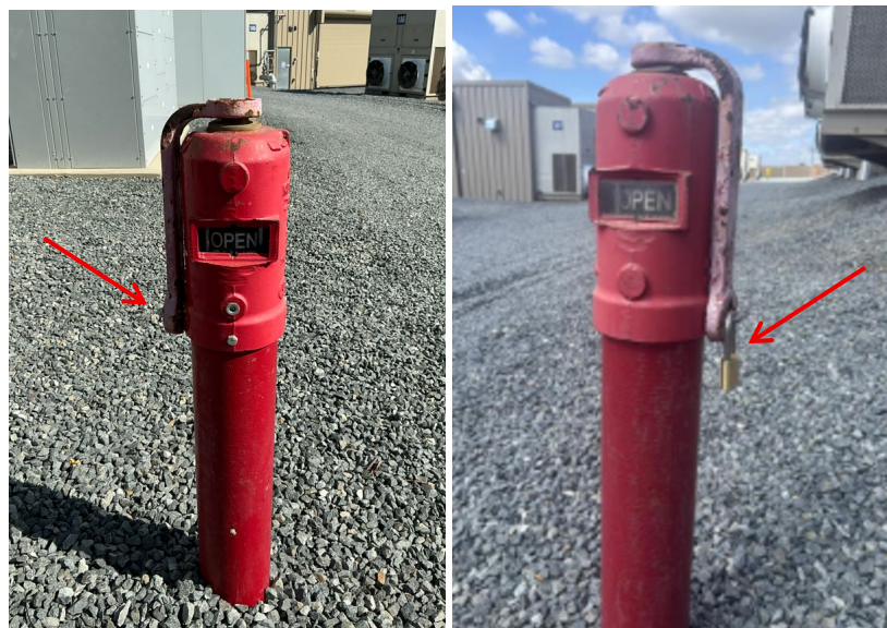
Figure 7: (Left) PIV without a proper locking mechanism. (Right) Valley Center locked the PIV during the audit.
