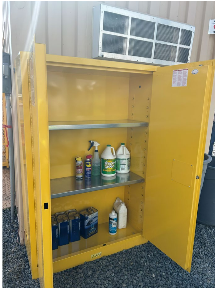
Figure 3: Flammable material storage cabinet without a self-closing mechanism.
