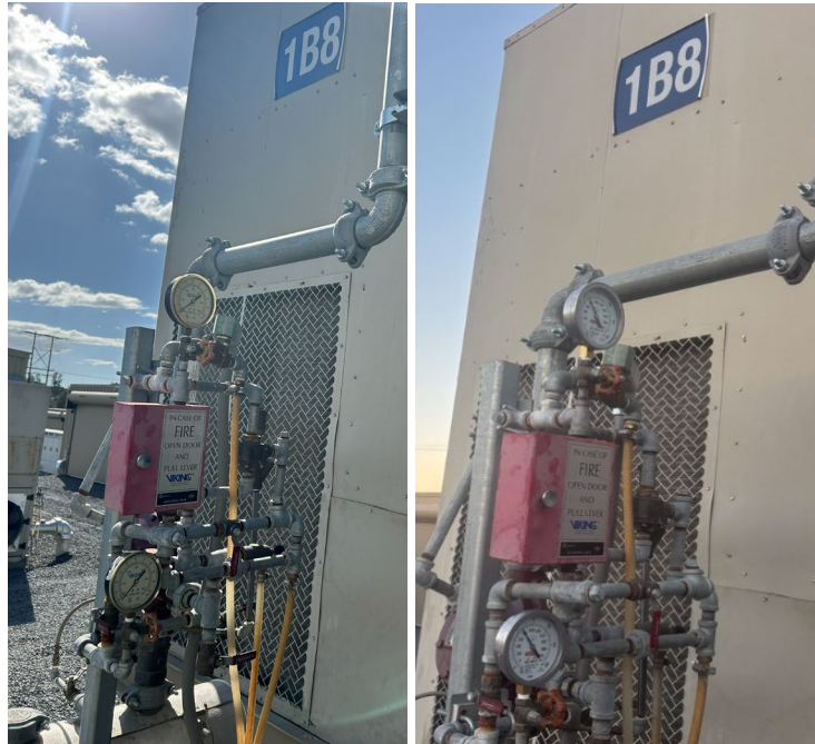
Figure 2: (Left) Both gauges on Unit 1B8 TRM system reading zero. (Right) Valley Center replaced both pressure gauges on Unit 1B8 during the audit.
