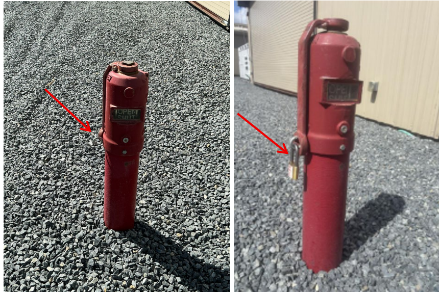
Figure 6: (Left) PIV with no locking mechanism. (Right) Valley Center locked the PIV during the audit.
