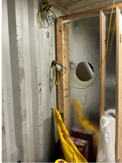
Figure 5: Valley Center removed the hot stick from site before the conclusion of the CPUC audit.
