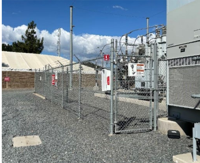
Figure 9: Fire extinguisher located on the substation gate not indicated on site map.
