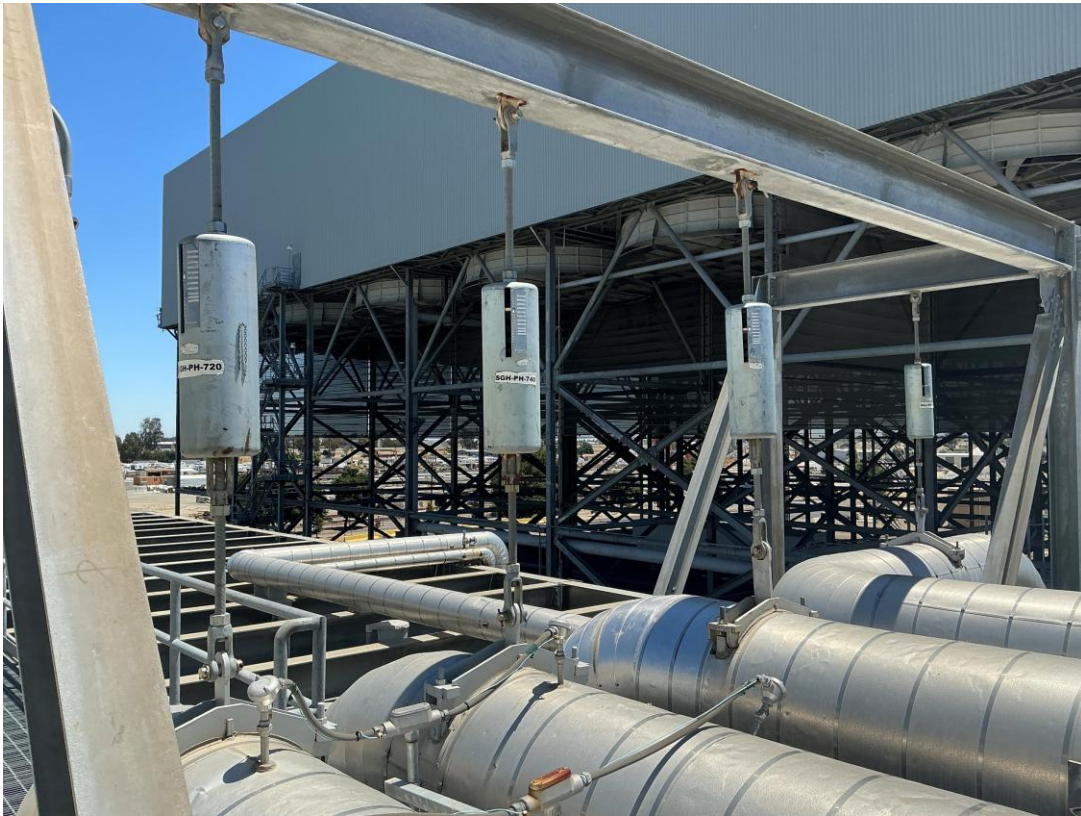
Figure 3: Pipe hanger without hot indications (Steam turbine deck).
