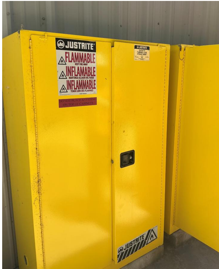
Figure 10: NFPA 704 Placard is not on a flammable storage locker.
