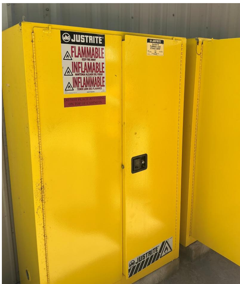
Figure 9: Flammable Storage Locker not latched.
