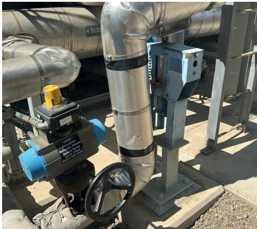
Figure 5: Pipe support exceeding hot condition.
