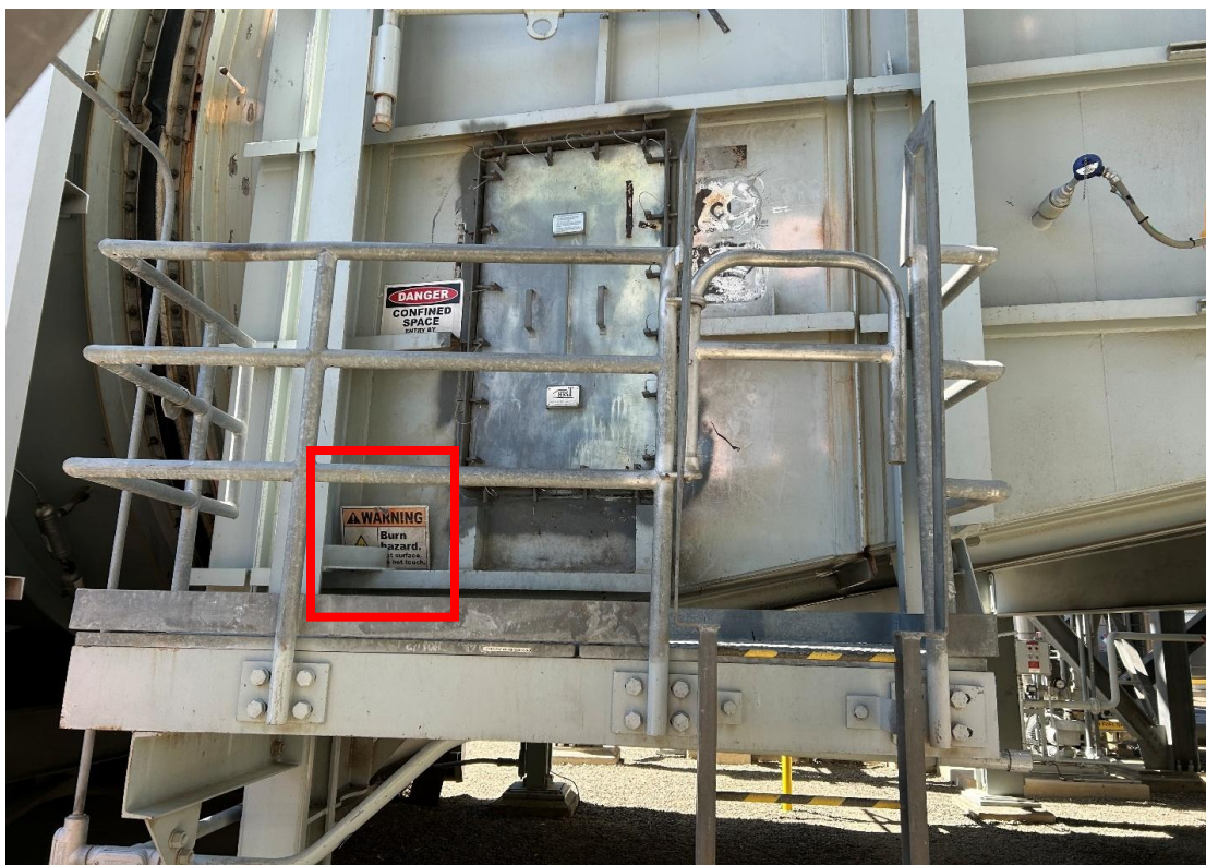
Figure 12: Sign stating “Burn Hazard” is not visible.
