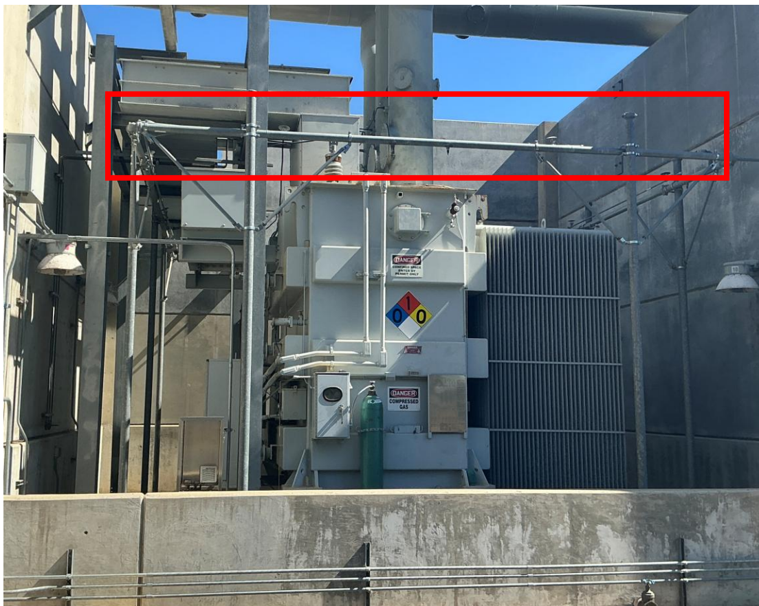
Figure 2: Deluge piping not adequately identified.
