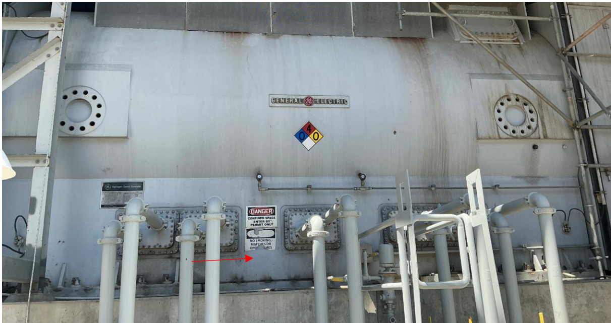
Figure 14: Sign stating “No Smoking Matches or Open Flames” is in poor condition on generator.
