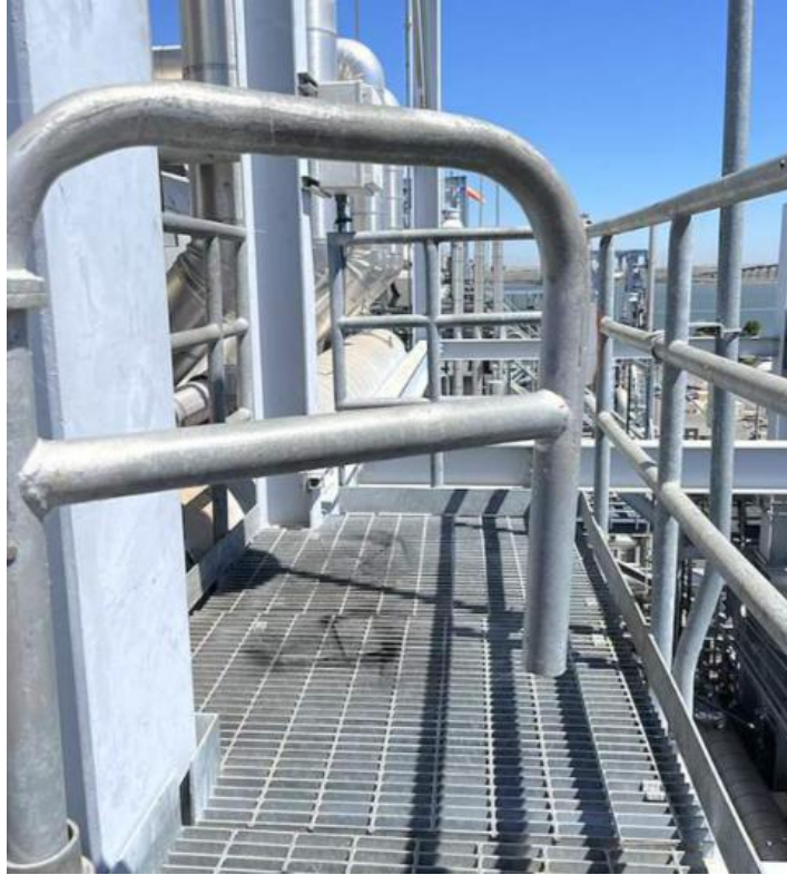
Figure 7: Staged swing-gate open on Heat Recovery Steam Generator (HRS) deck.
