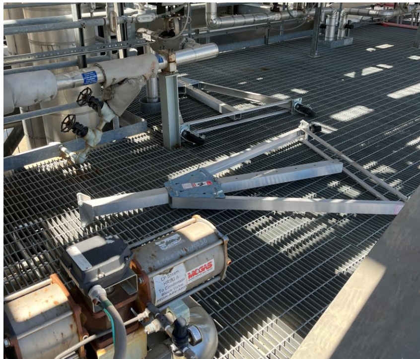
Figure 21: Unsecured equipment on an elevated platform.
