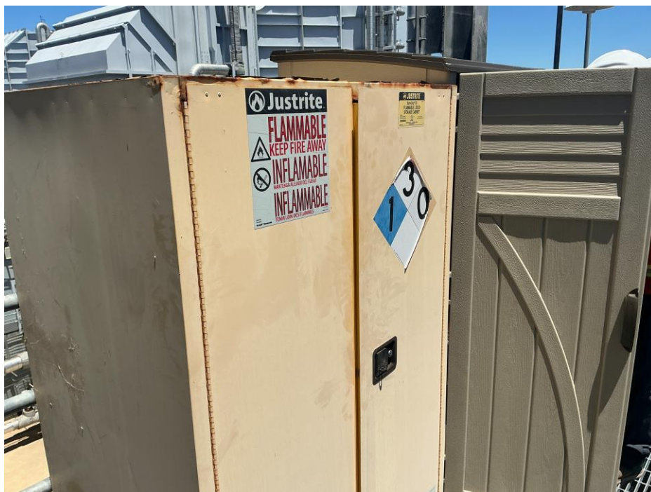
Figure 8: Flammable Storage Locker not latched.
