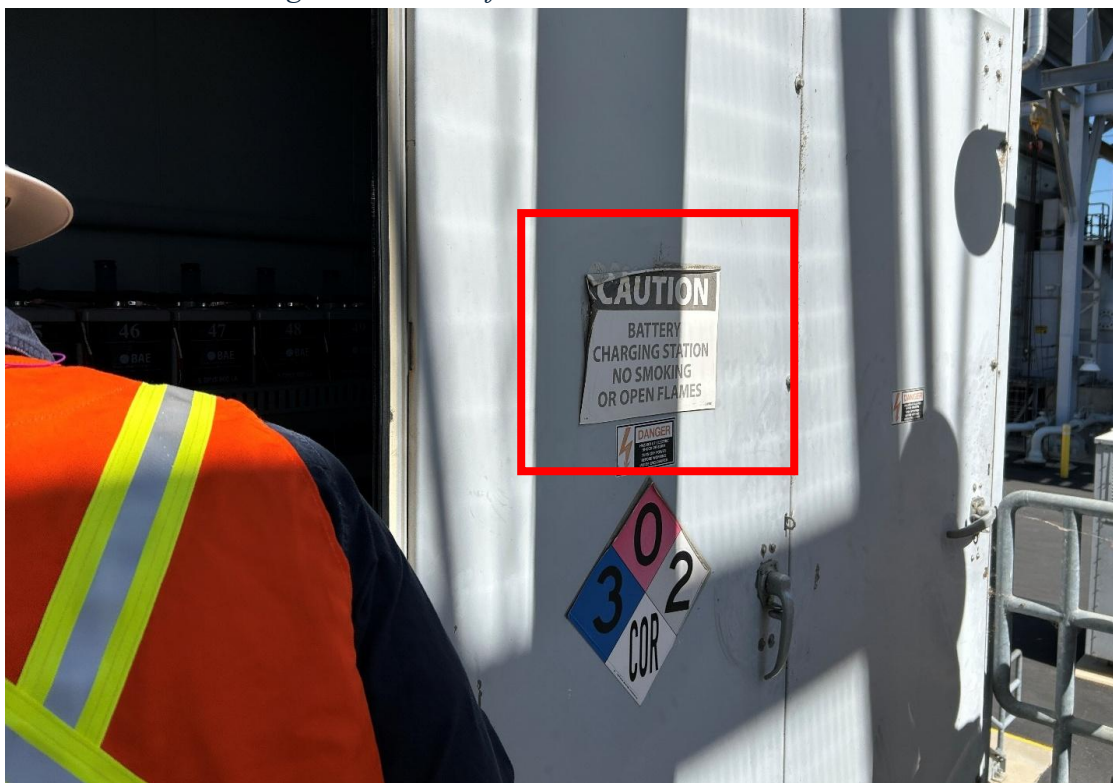
Figure 17: Sign identifying a battery charging station is degrading.
