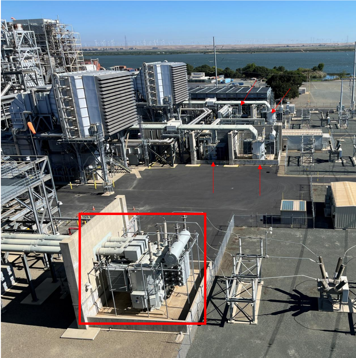
Figure 1: View of transformers with deluge-style fire suppression systems.
