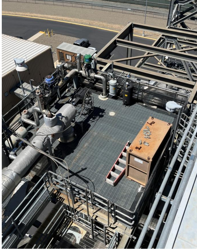
Figure 19: Unsecure ladder and loose parts on an elevated surface.
