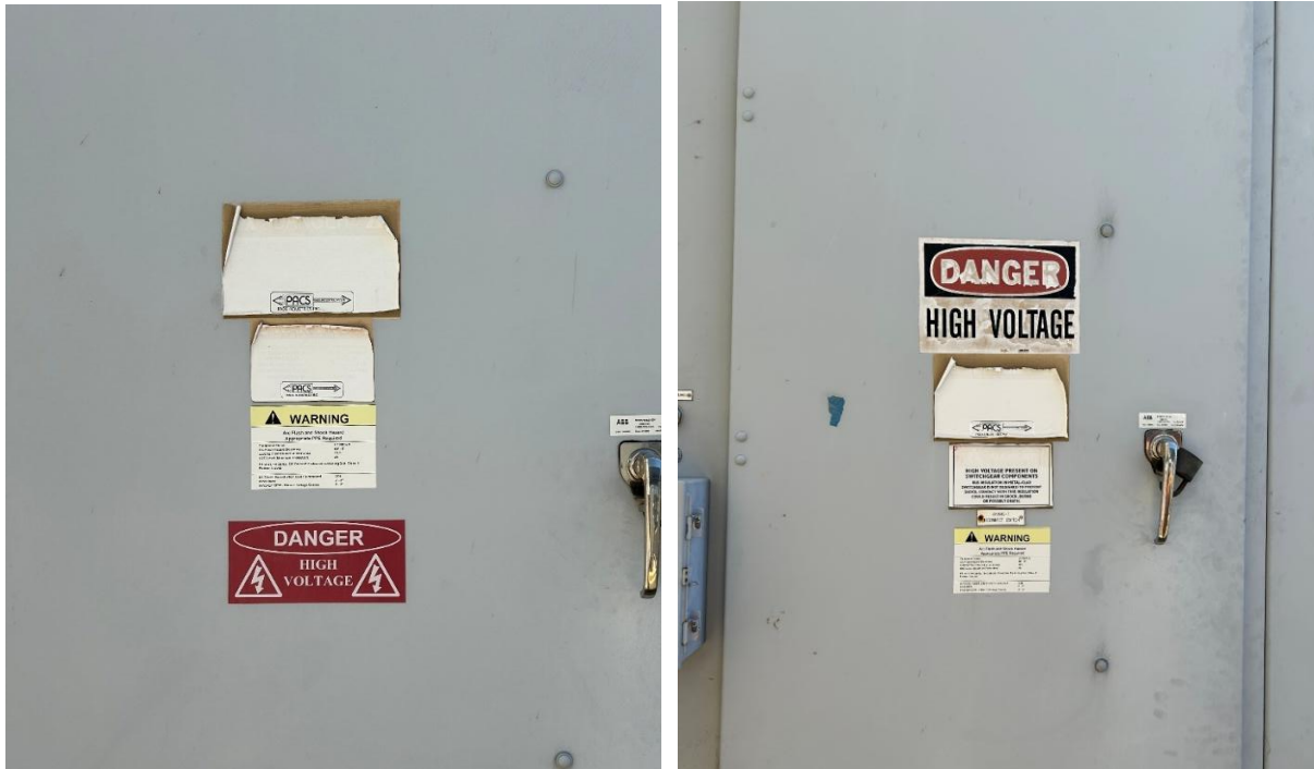
Figure 18: Illegible warning signs.
