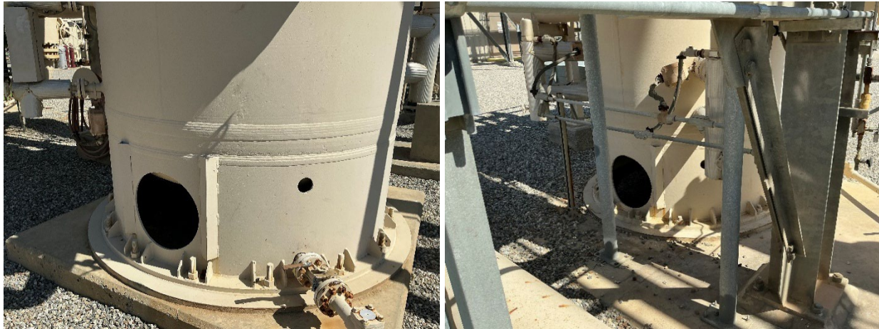
Figure 11: Confined space entry point without signage.
