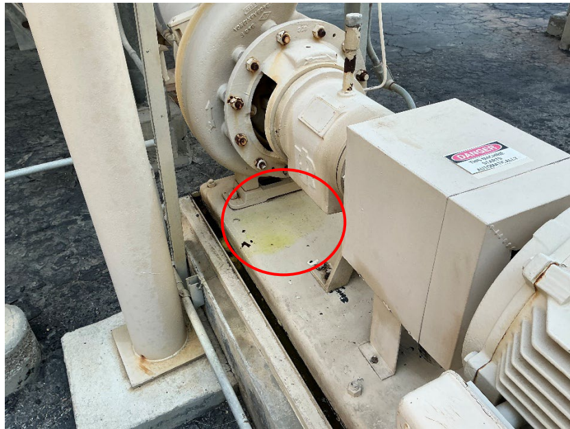
Figure 14: Oil residue on Pump P408-B.
