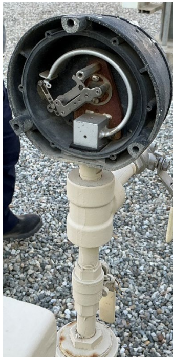
Figure 6: Missing backplate on liquid Gauge.
