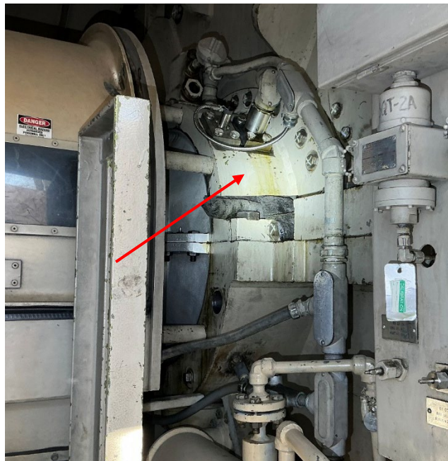
Figure 13: Oil leak on Unit A Generator equipment.
