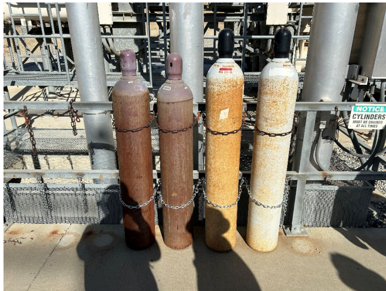
Figure 3: Unmarked SF6 gas cylinder in substation.
