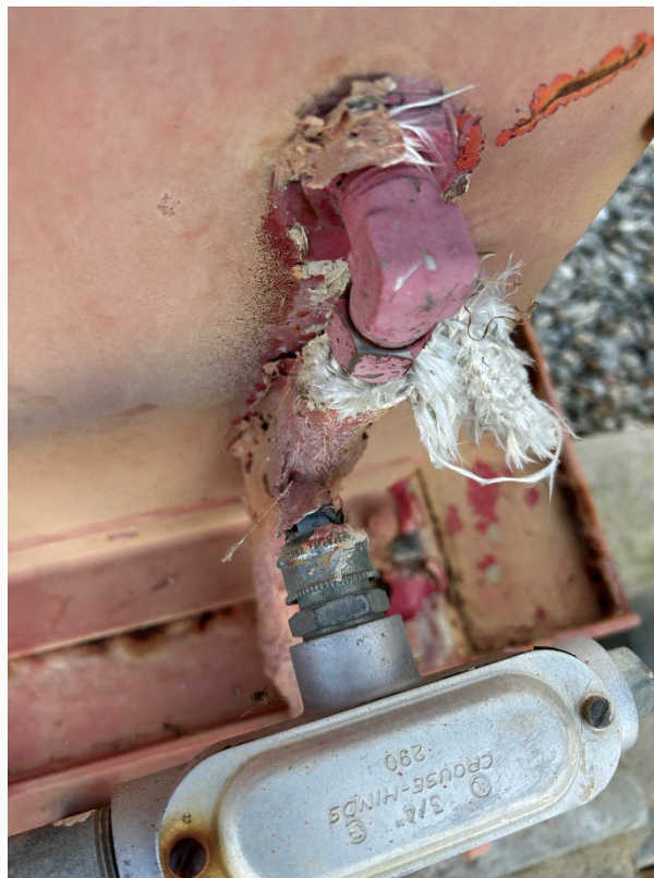
Figure 5: Deteriorated wire shielding on pressure sensor serving the fire pump.
