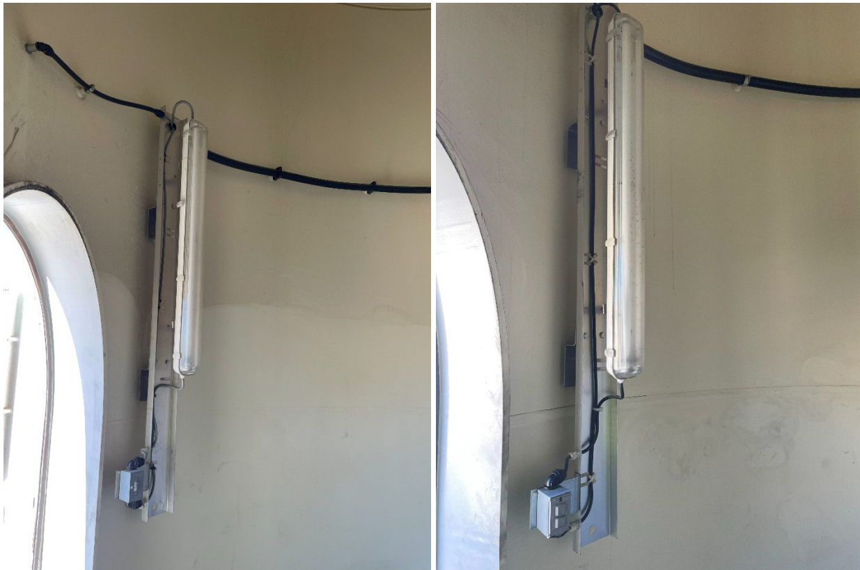
Figure 5: Non-operational lighting on turbines 1-0056 & 1-0064.
