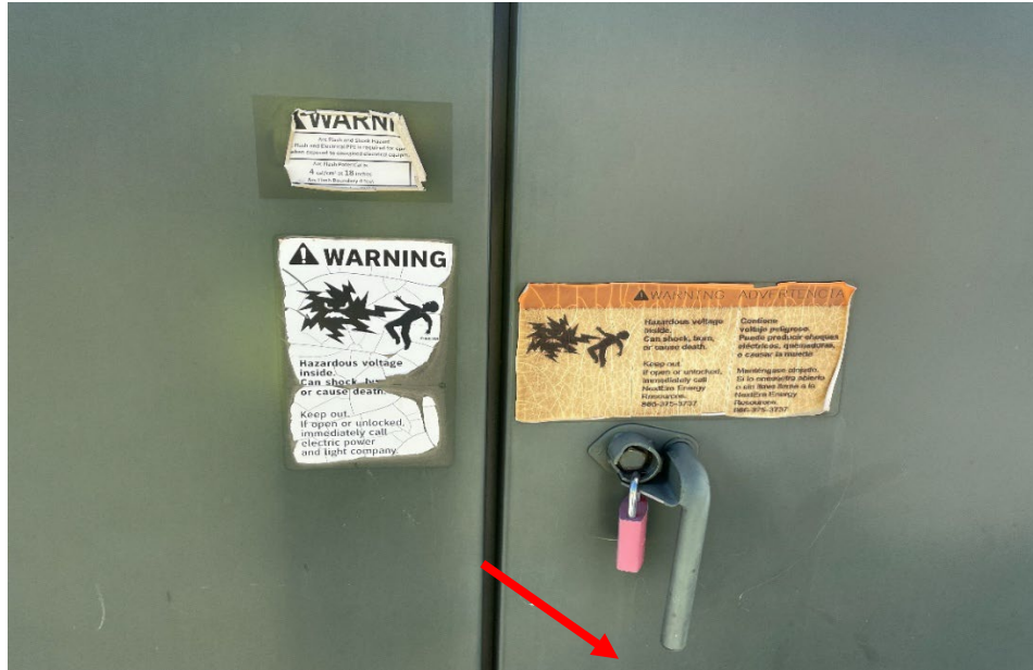
Figure 7: Sun faded and damaged arc flash label on pad mounted transformer 1-0064.
