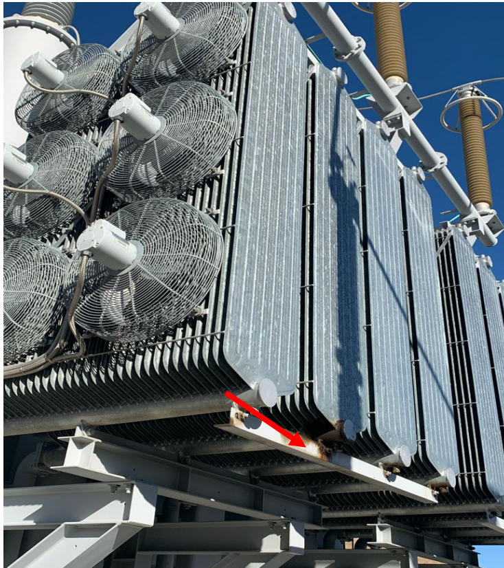
Figure 4: Evidence of oil leak on the substation GSU transformer.
