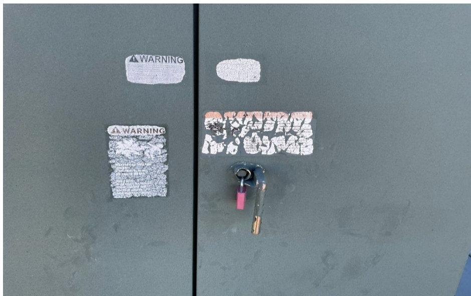
Figure 8: Sun faded and damaged arc flash label on pad mounted transformer 1-0056.
