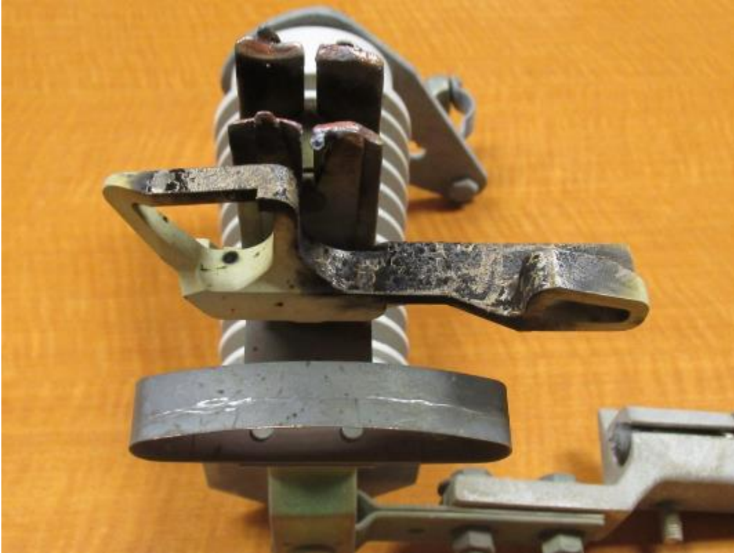
Figure 9: Rotating contact, west end, north conductor of pole switch PS 2191
