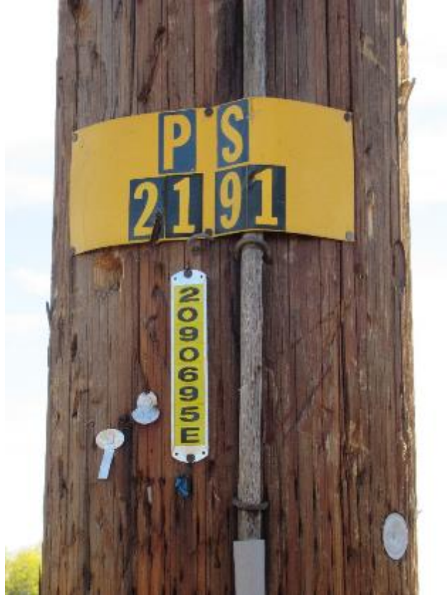
Figure 12: Edison pole number 2090695E and pole switch PS 2191 pole markers
