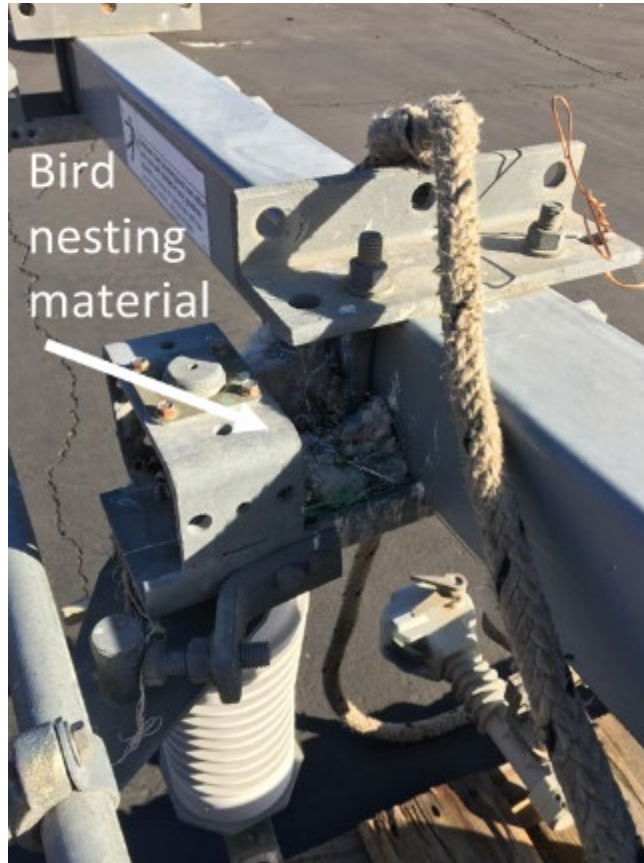
Figure 10: Bird nesting material above the section of the switch that connects the middle conductor phase of pole switch PS 2191. 56
