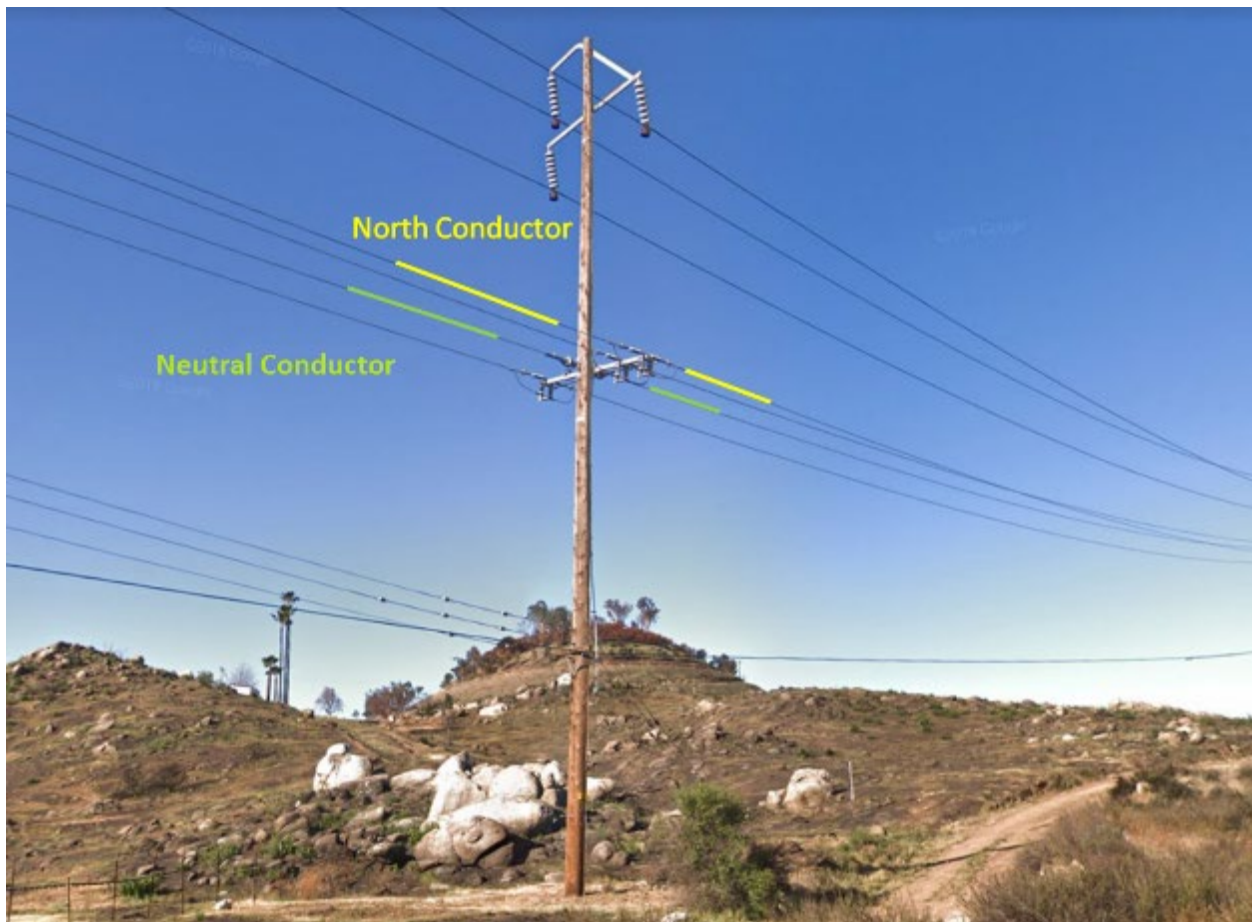
Figure 7: Looking south west at pole 2090695E and PS 2191 (Picture for example purpose only, image date April 2018, newly installed 12ft Omni-rupter pole switch shown)
