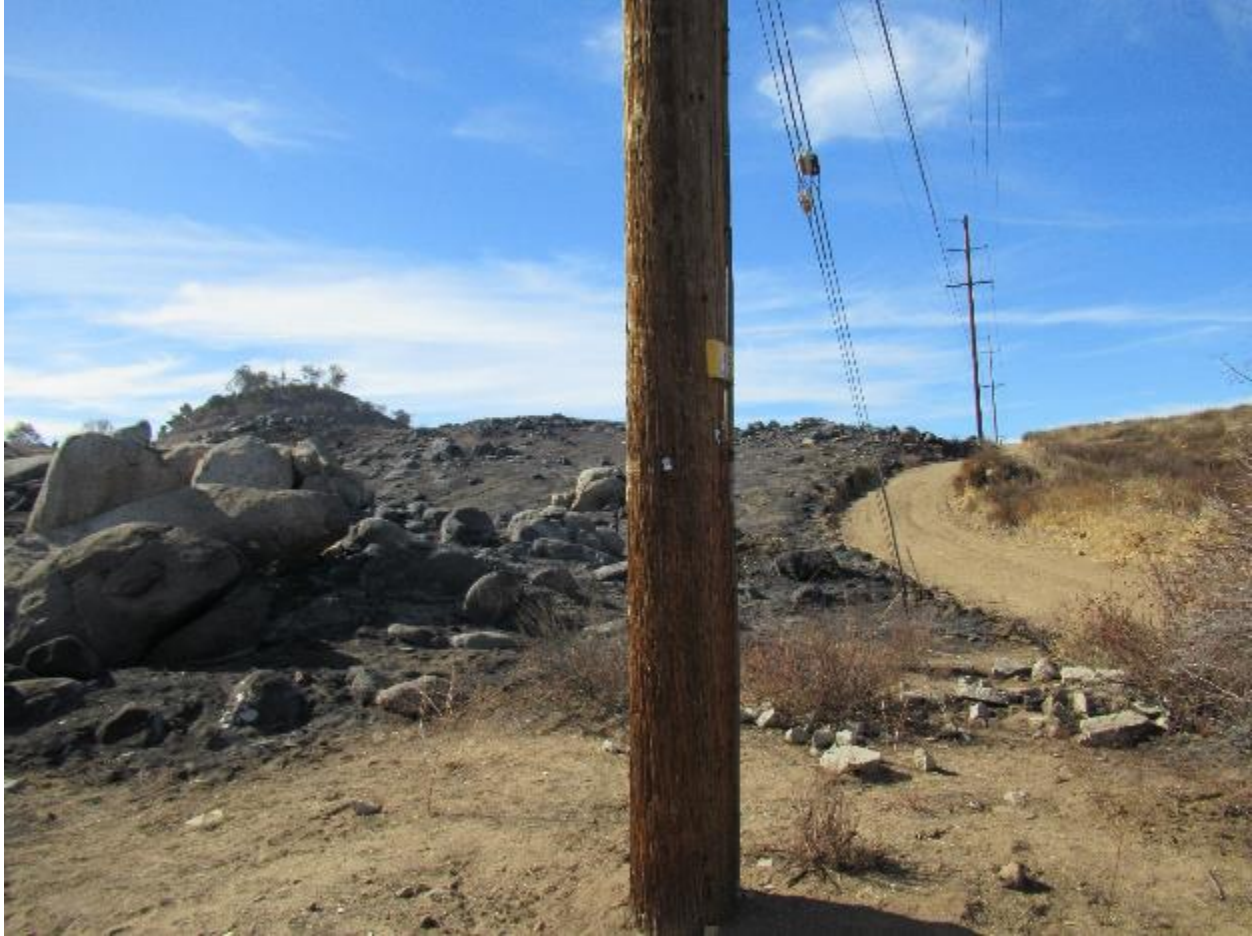
Figure 11: Brush at the base of Edison pole 2090695E
