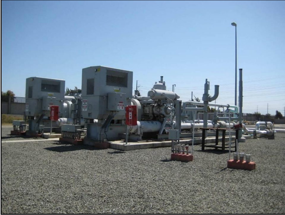
Photo 2: Fuel gas compressors at the gas yard.
