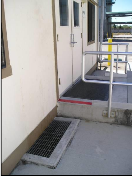
Photo 3: Trip hazard at a building ramp.
