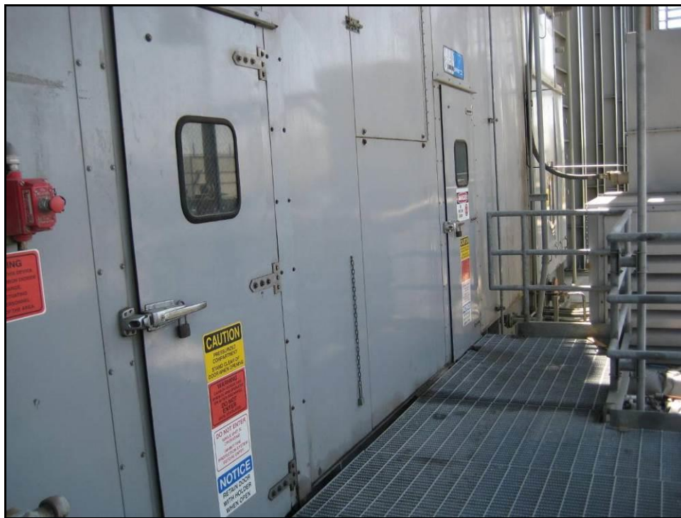
Photo 1: Turbine compartment lacked a warning sign.
