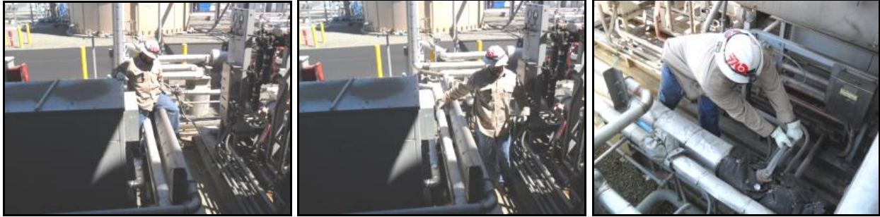
Photo 8: Operator maneuvered pipes and conduits in order to access a shutoff valve.
