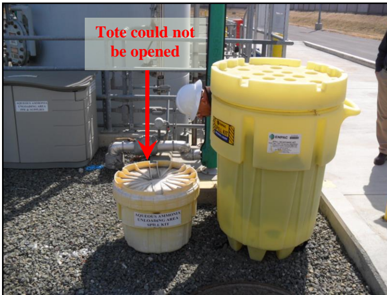
Photo 12: Spill kits at the ammonia storage tank.
