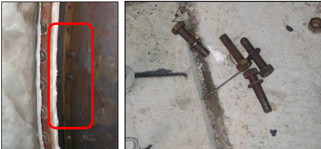
Photo 6: Connector bolts failed at Metcalf's Unit 1. Source: March 22, 2007 File Photo
