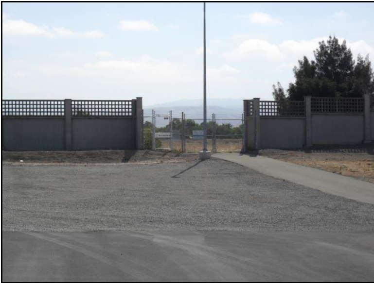
Photo 10: Perimeter walls are not monitored and lack barbed wire to deter intruders.
