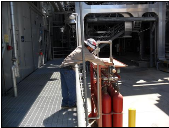
Photo 9: Operator leaned over a guardrail to shutoff a CO 2 valve.
