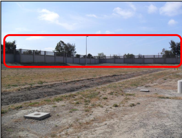
Photo 11: South perimeter wall has excessive vegetation providing an intrusion path.
