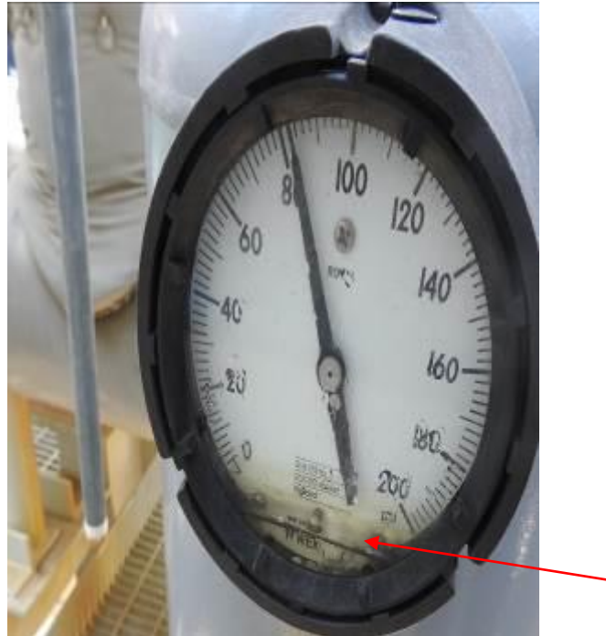
Water deposition inside the Pressure gauge
