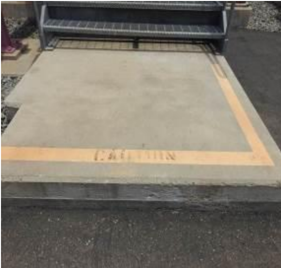
Caution sign for the step are worn out
