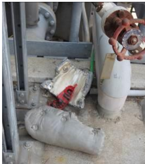
Abandoned insulation cover
