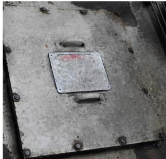
Faded confined space warning sign
