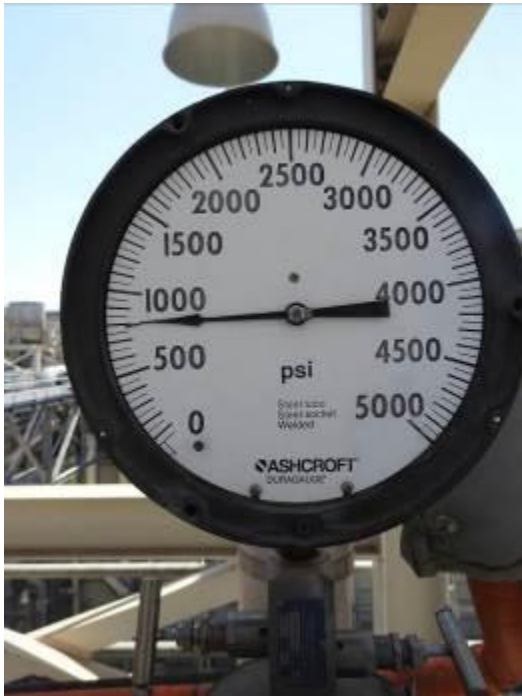
Pressure gauge missing the glass cover
