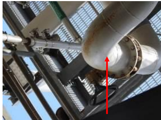
Leaking condenser water-box vent valve
