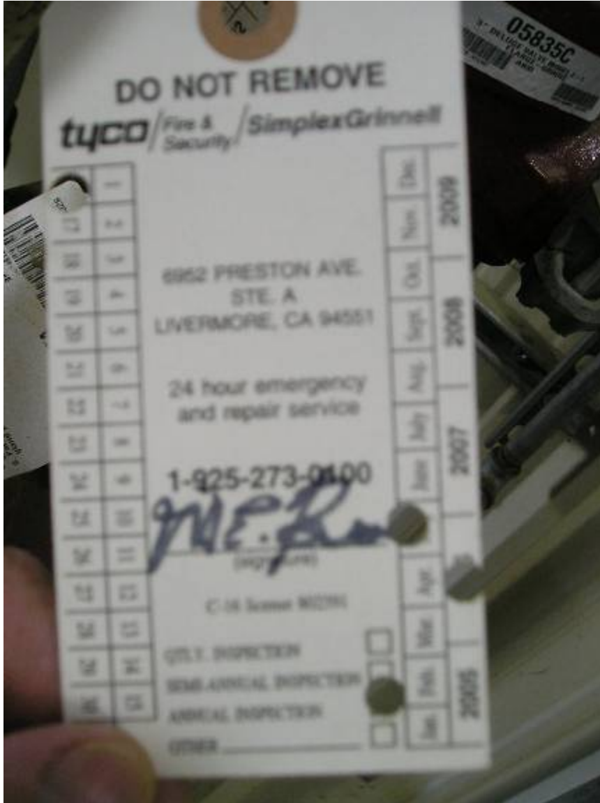
Photo 34: Close-up of the fire suppression system inspection tags show an inspection date of May 2006.
