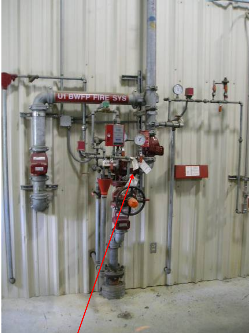
Photo 33: Inspection tags are visible on the boiler feedwater pump fire suppression system.
