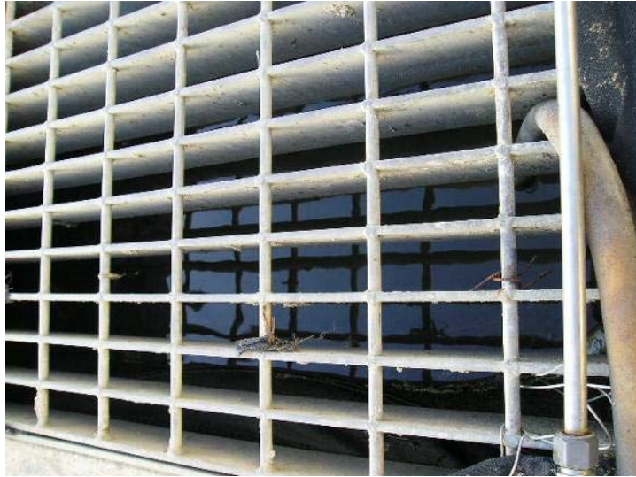
Photo 21: Clogged debris screen in storm drain.
