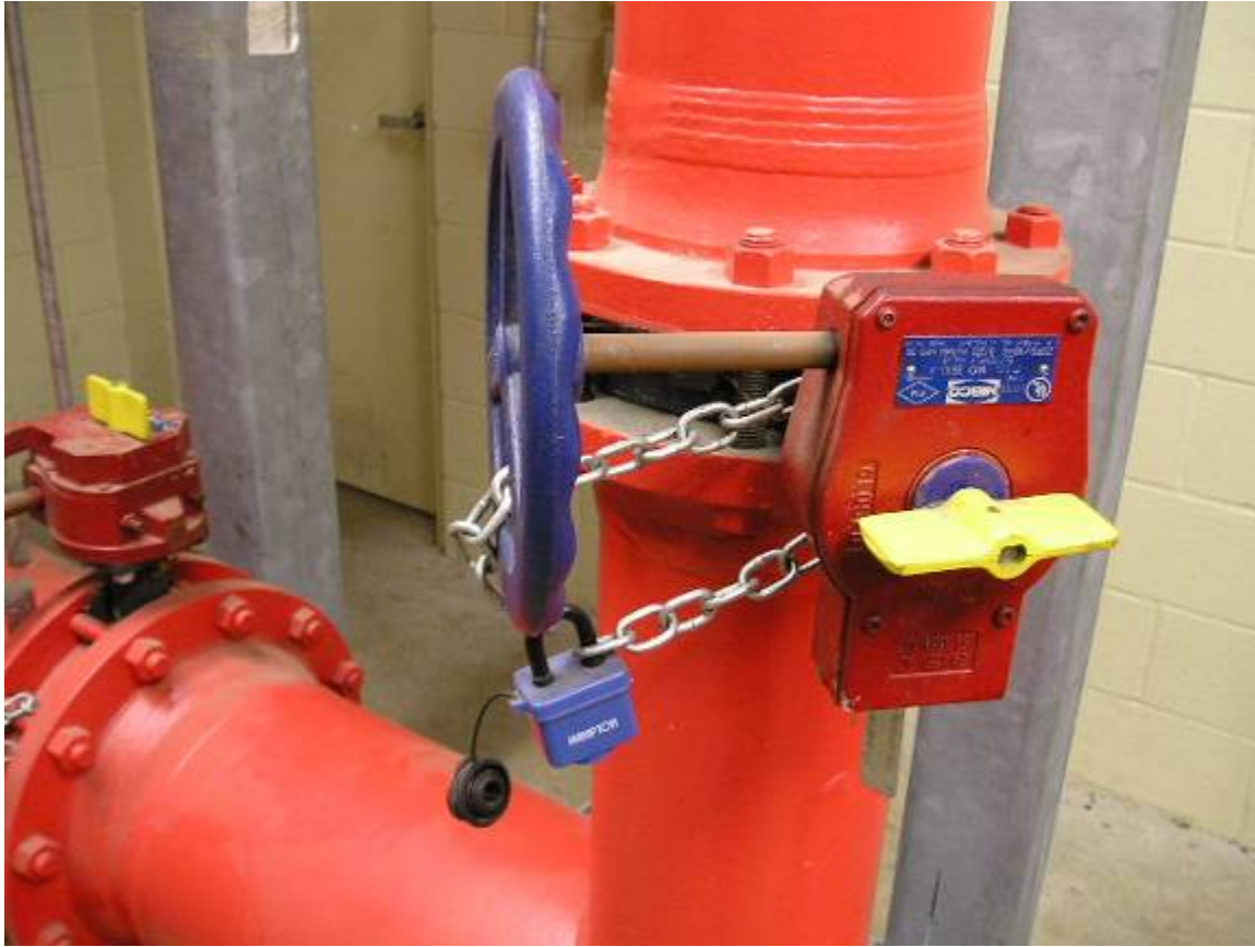
Photo 36: Locks are installed to prevent accidental closure of valves as recommended in the May 2006 inspection.
