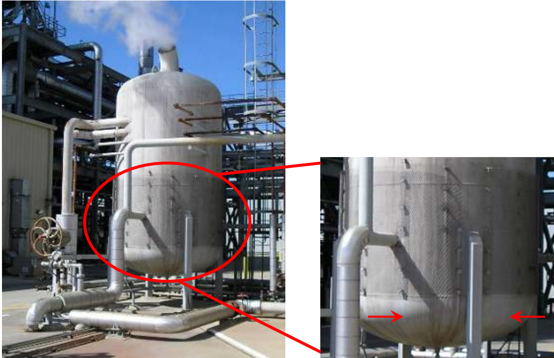
Photo 9: Blowdown tank's lower portion lacks protective barrier.
