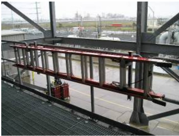
Photo 31: The plant stores ladders on hangers, leaving walkways clear.
