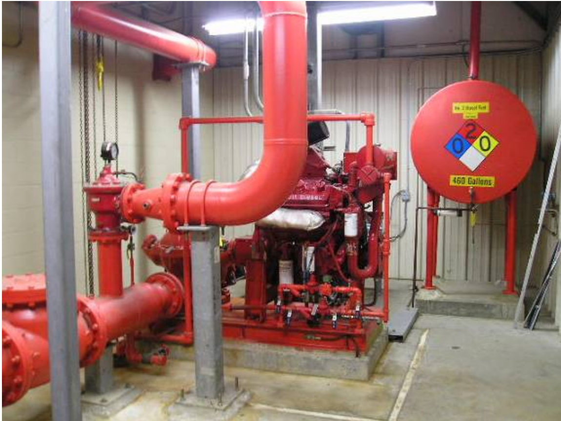
Photo 35: The main diesel powered fire pump
