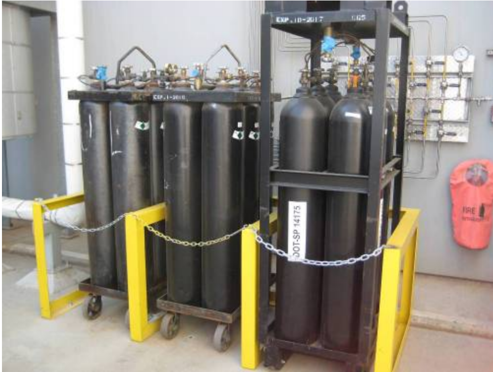
Photo 13: Improved storage of high pressure cylinders.
