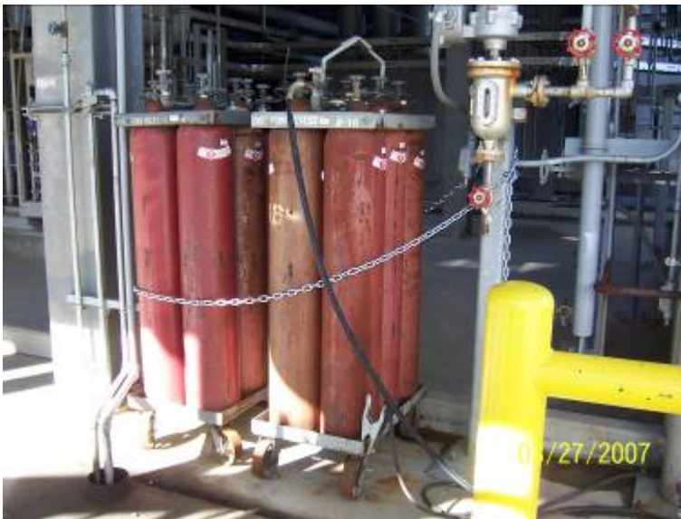
Photo 12: High pressure hydrogen cylinders are not properly secured.
