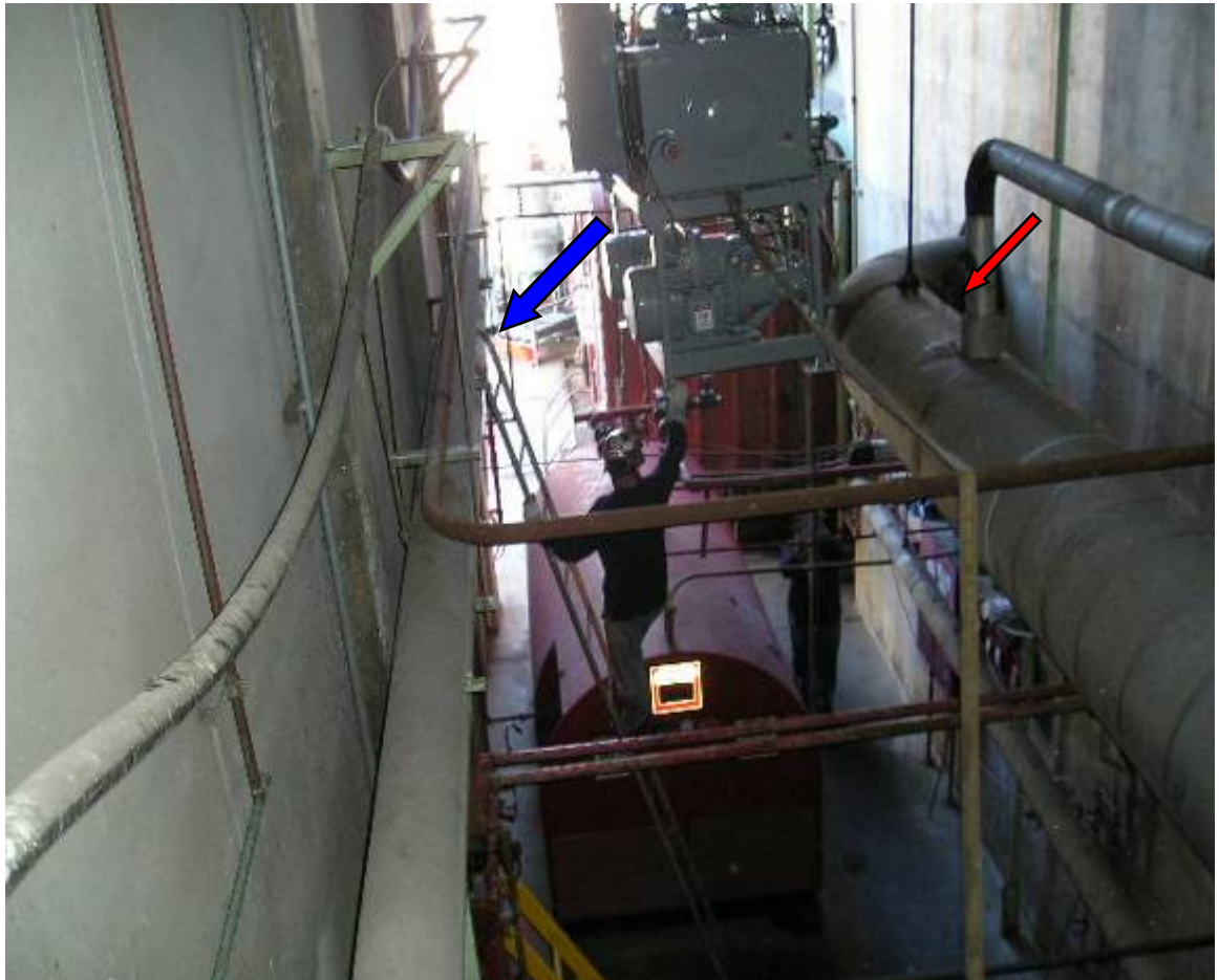
Photo 15 The ladder is not secure. The top right of the ladder (blue arrow) swings back and forth rapidly approximately 6 inches or more from the wall as the worker is attempting to position the hanging structure. Note: The structure on the pulley has moved closer to the camera. It is now close to the steam pipe insulation (red arrow) on the right, forward and above the person standing below.
