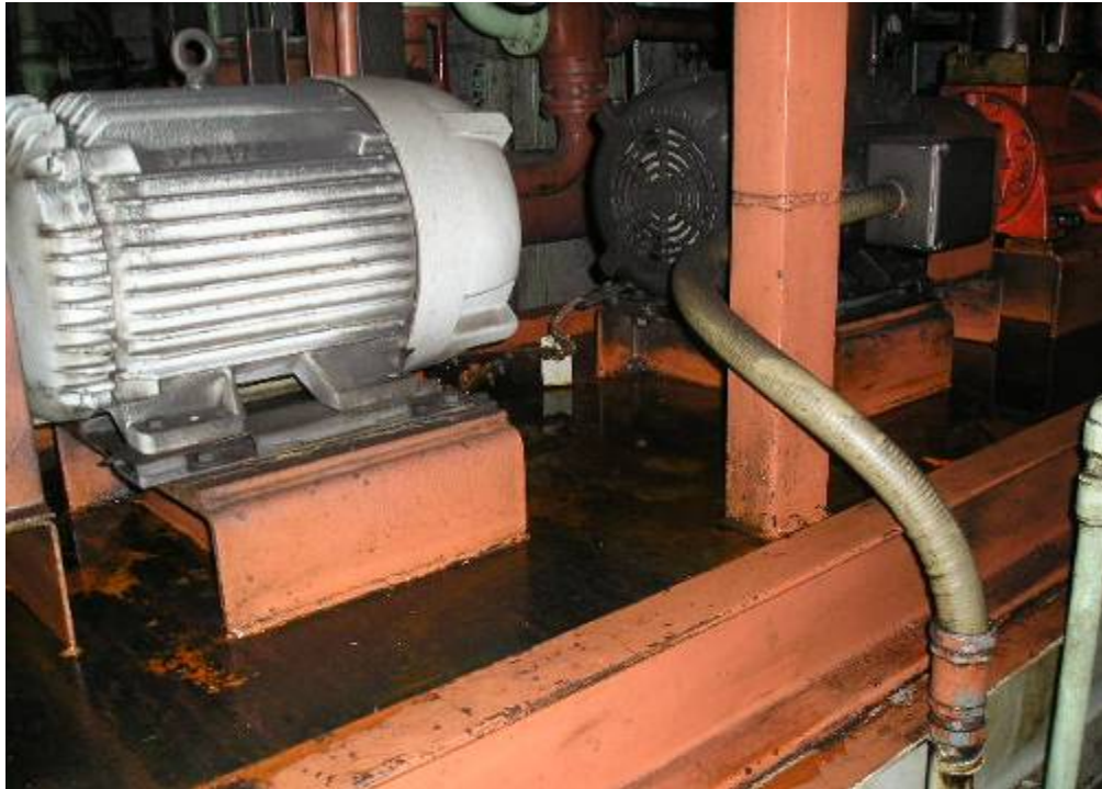
Photo 6 Pooling of oil was observed on the skid of the Lube Oil Supply Pump to the Main Boiler Feed Pump.
