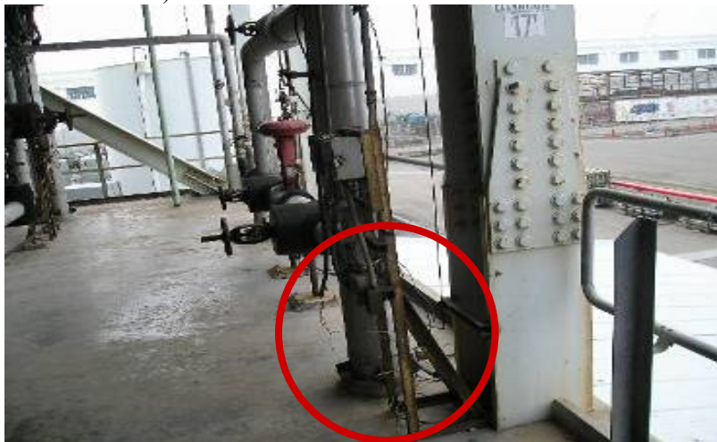
Photo 3 Loose wiring at Elevation 17, Column 11-L – See Photo 4 for close-up view.
