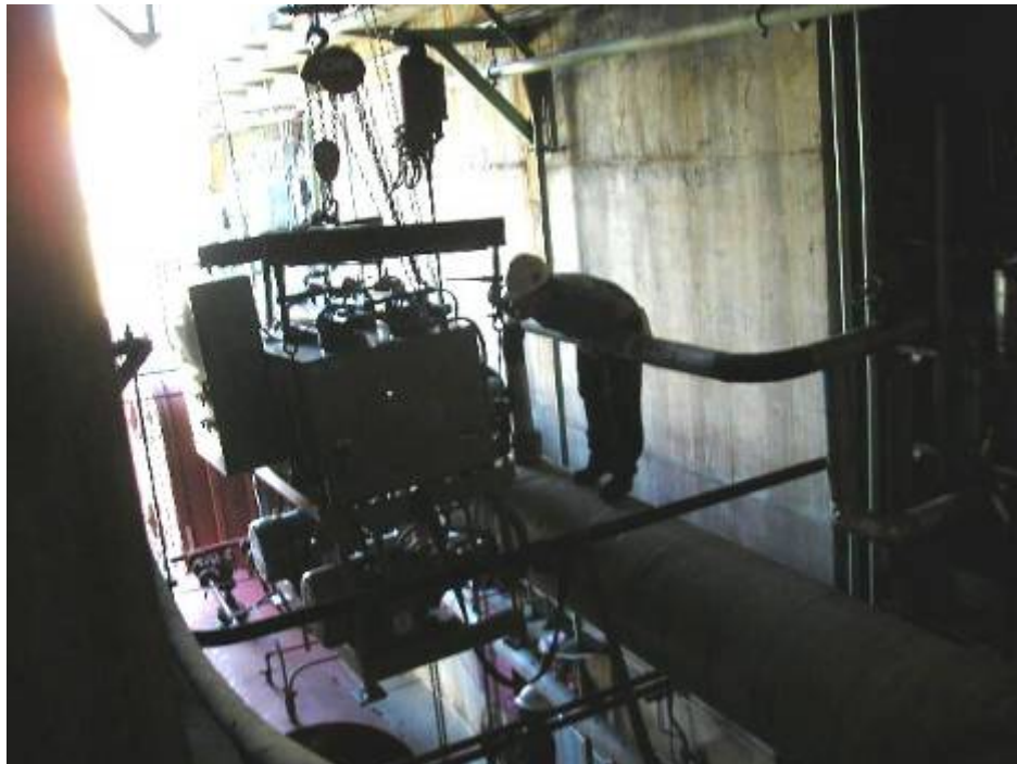
Photo 17 Worker lacks fall protection (Worker on pipe is near red arrow in Photo 15.) When CPSD auditors expressed safety concern, the plant manager responded that a worker on a steam pipe may be a safety concern and went to the lower level to discuss the concerns with the workers involved.
