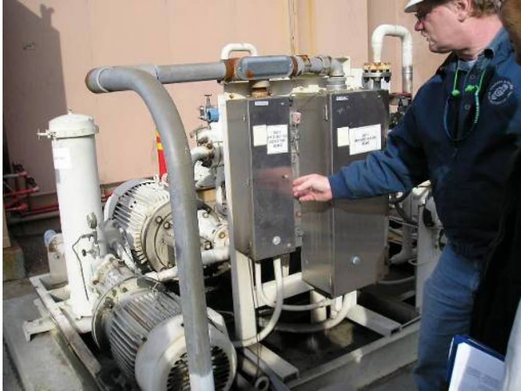
Photo 12 An intruder had tripped this Circuit Breaker (52-33-9B) causing a previous outage
