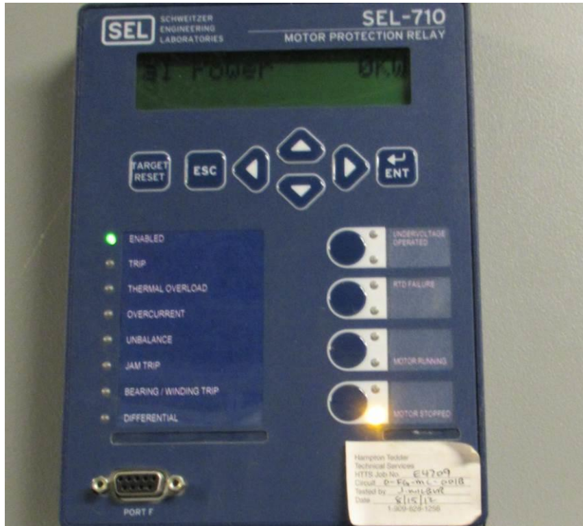
Figure 12: Calibration stickers are not kept up-to-date.
