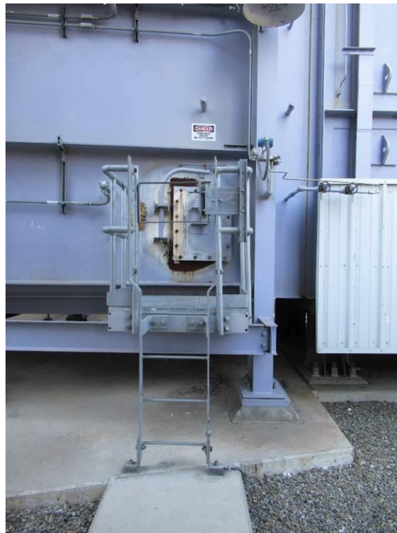
Figure 1: Manway hatch is severely corroded and presents a burn risk for workers.
