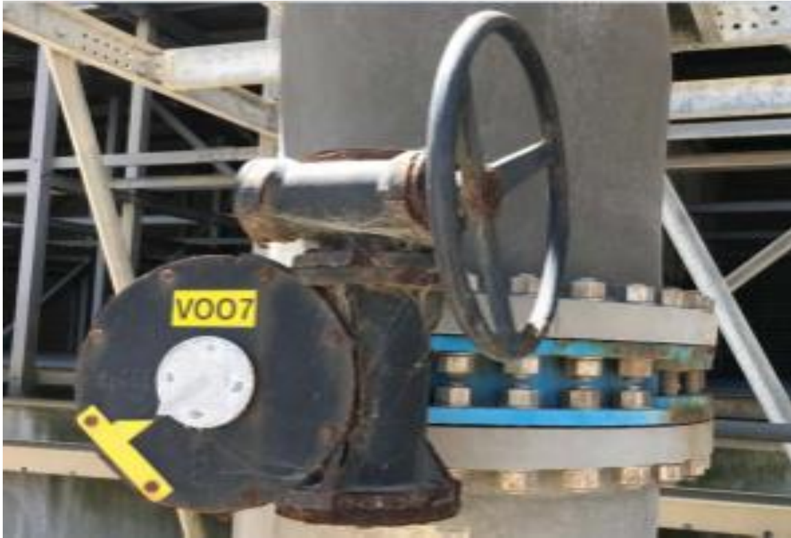
Figure 7. Corroded riser butterfly valve at the cooling tower.
