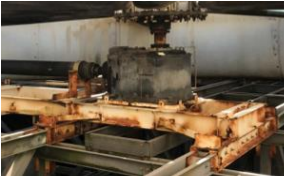
Figure 8. Corroded support braces.
