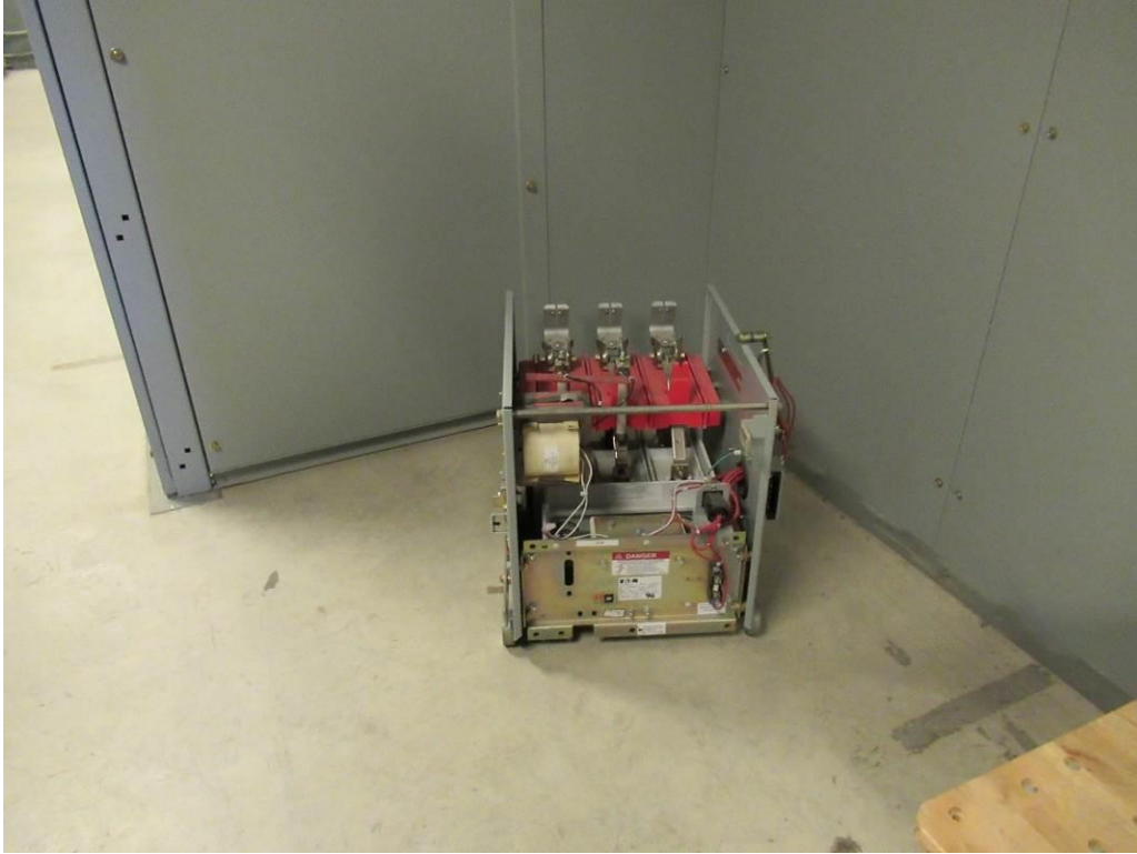
Figure 15: Improper storage of spare component.
