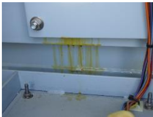
Figure 11 is a photograph of oil that was observed to be leaking at an inverter panel.
