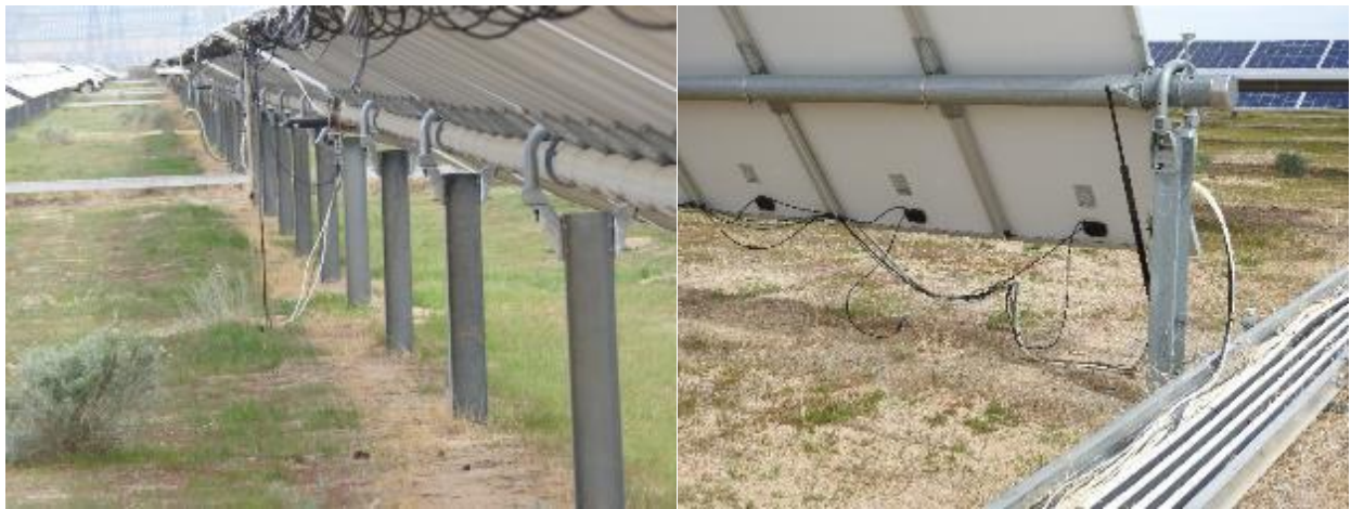
Figures 5 and 6 are displaying cables that have detached from panels and contacting the ground.
