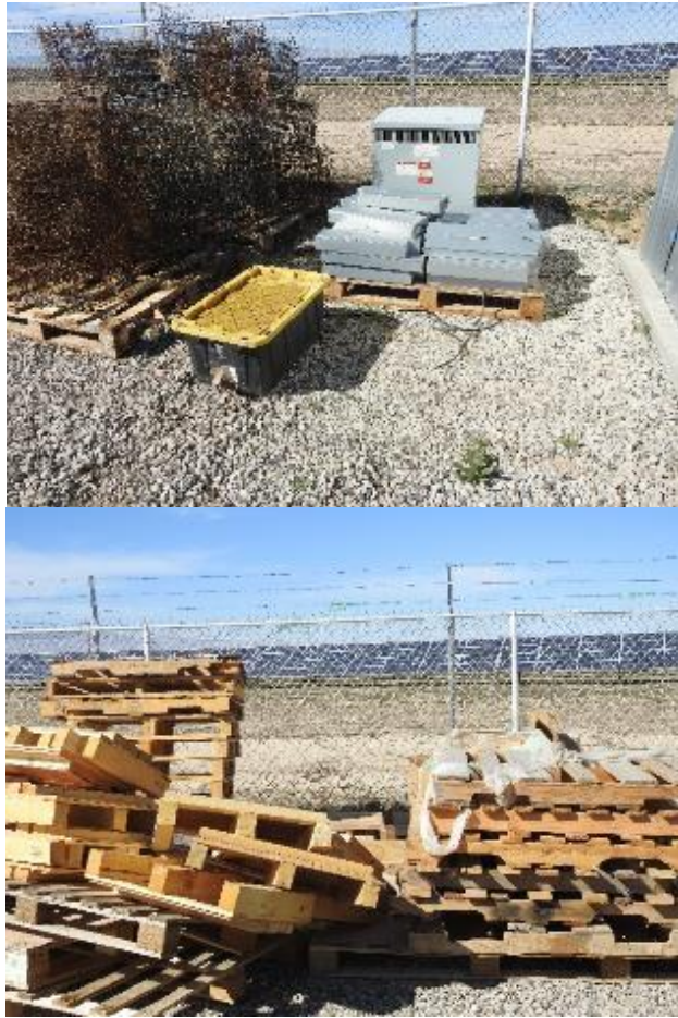
Figure 1 is of a storage container that contained an unidentified fluid and a pallet supporting electrical components left outside unprotected. Figure 2 is of a photograph of a stack of disarray pallets.
