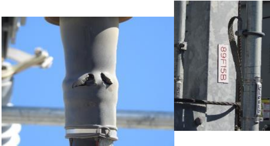
Figure 12 is a photograph of the damaged insulator boot and Figure 13 is the structure ID of the facility.
