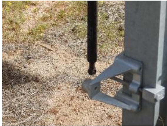
Figure 10 is displaying an observed detached solar array strut.
