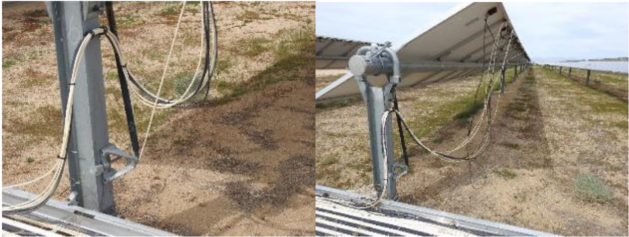
Figures 3 and 4 are photographs of a cable that was caught on the strut of the solar panel structure.
