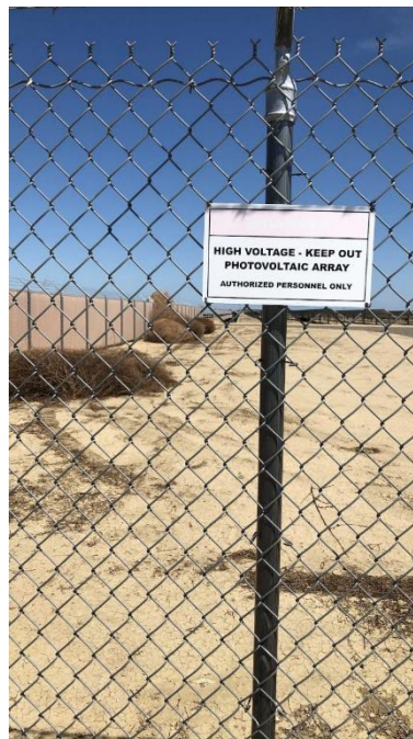
Figure 13. Fading “Danger High Voltage” sign at the B Block, on the south side fence.
