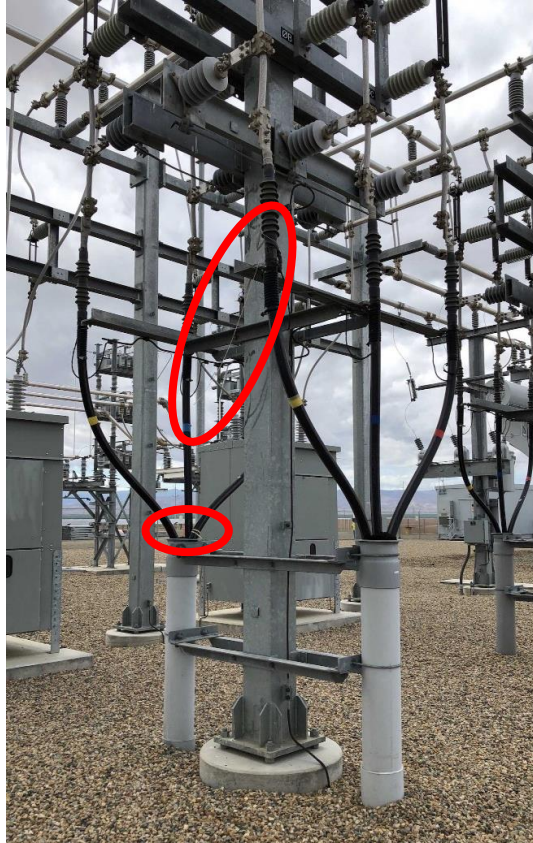
Figure 16. Strings wrapped around feeder conductors on the GSU 1 side.
