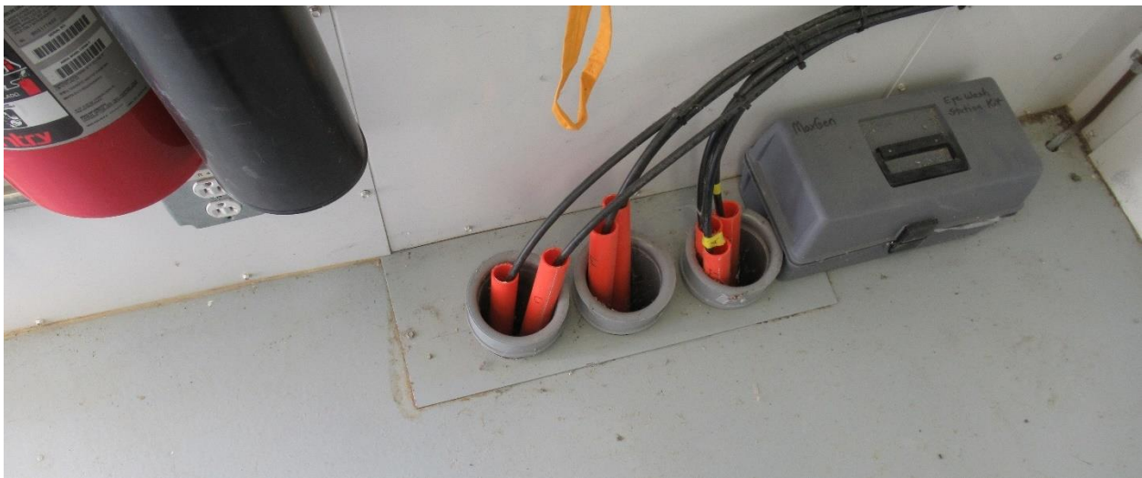
Figure 5. Unsealed cable conduits in the substation control room.
