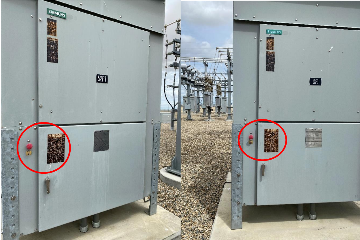
Figure 10. Fading signs on Circuit Breaker 52F1 (left) and 52F3 (right) in the substation.
