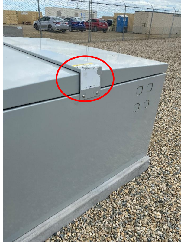
Figure 12. Fading sign on the auxiliary transformer (Aux 52) in the substation.
