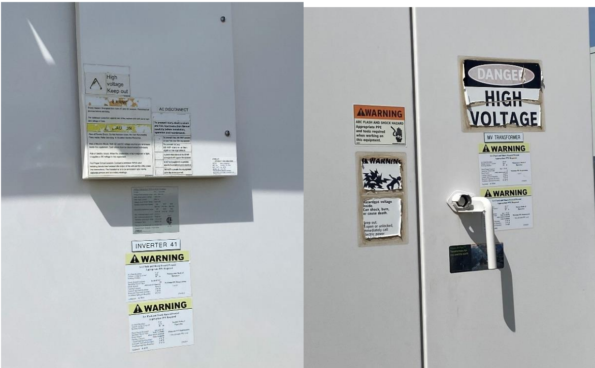
Figure 11. Fading signs on Inverter 41 (left) and fading and peeling signs on the medium voltage transformer (right) for the inverter.
