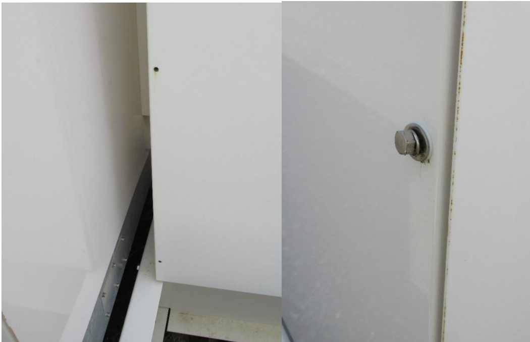
Figure 1. Missing and loose fasteners on Inverter 41 panels.
