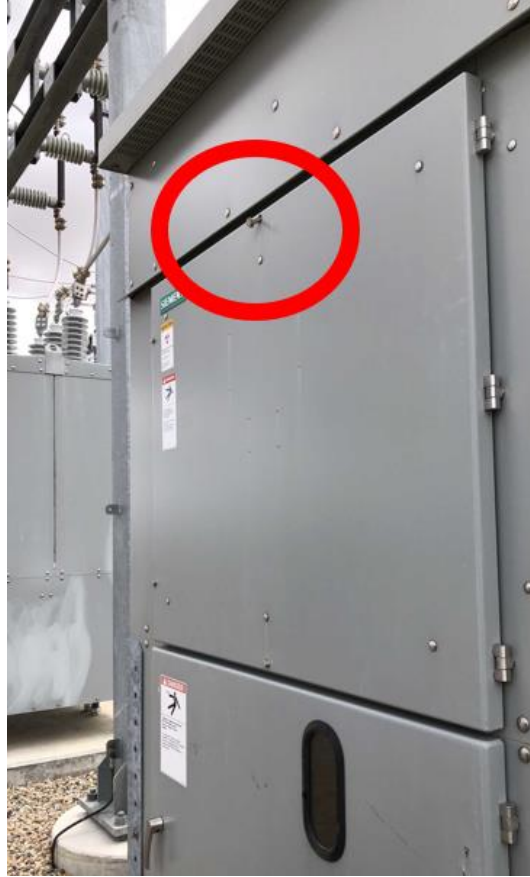
Figure 2. Loose fastener on Feeder Breaker 52F1.
