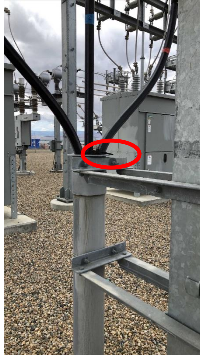
Figure 15. Broken zip tie on a feeder conductor on the GSU 1 side.
