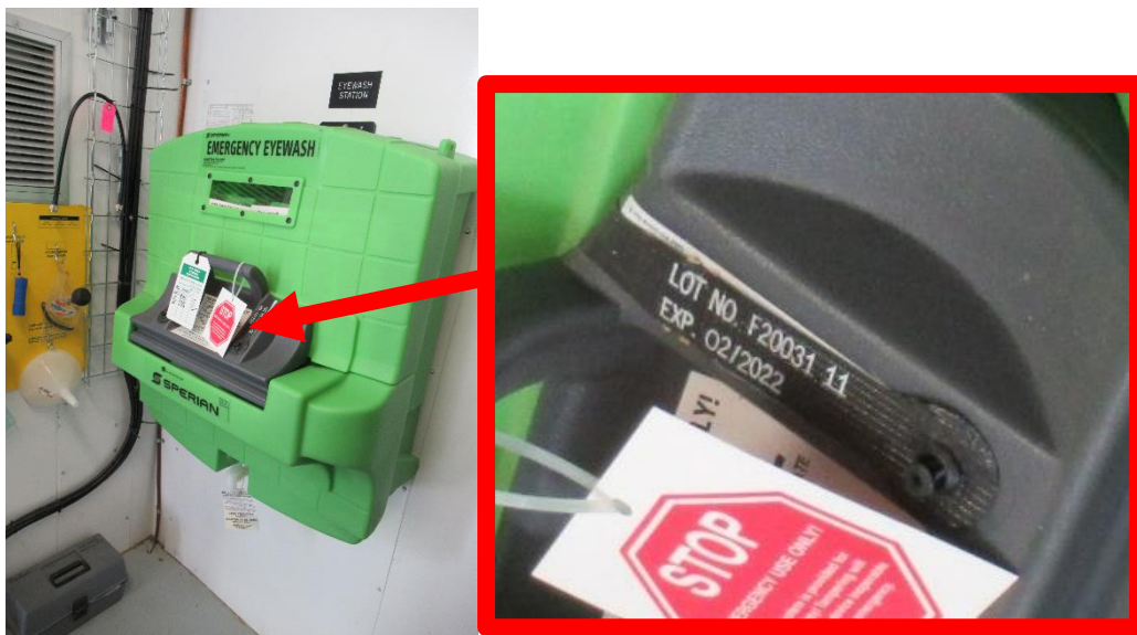
Figure 3. Expired eye wash station in the substation control room.
