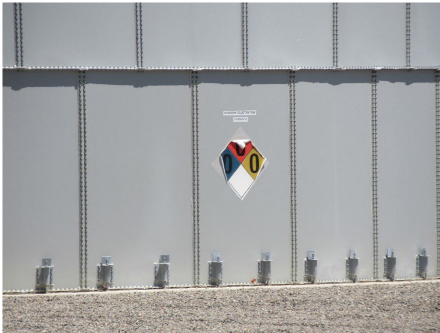
Figure 12 : Damaged NFPA diamond on the blowdown collection tank.
