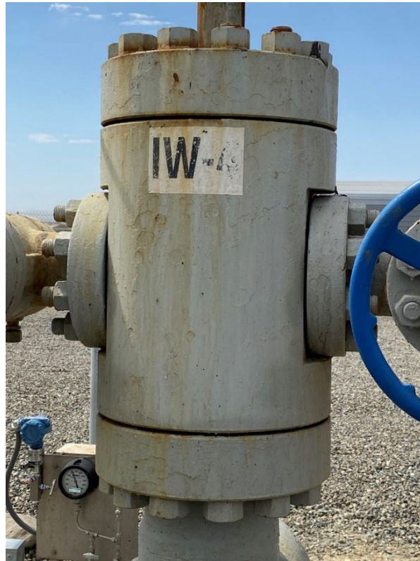
Figure 7 : Injection Well #4 equipment label is faded and illegible.
