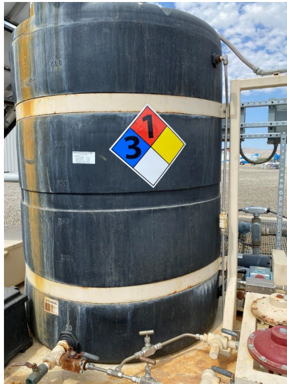
Figure 6: The Annulus fluid NFPA diamond at Injection Well 4 is missing its yellow reactivity number.
