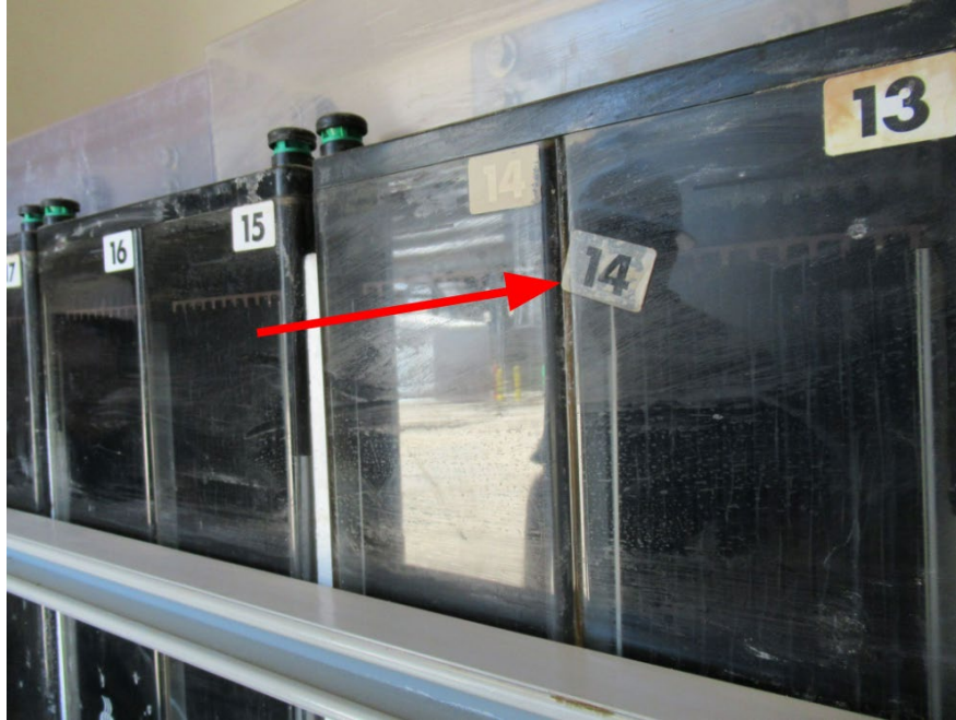
Figure 14 : Battery equipment labels are falling off.
