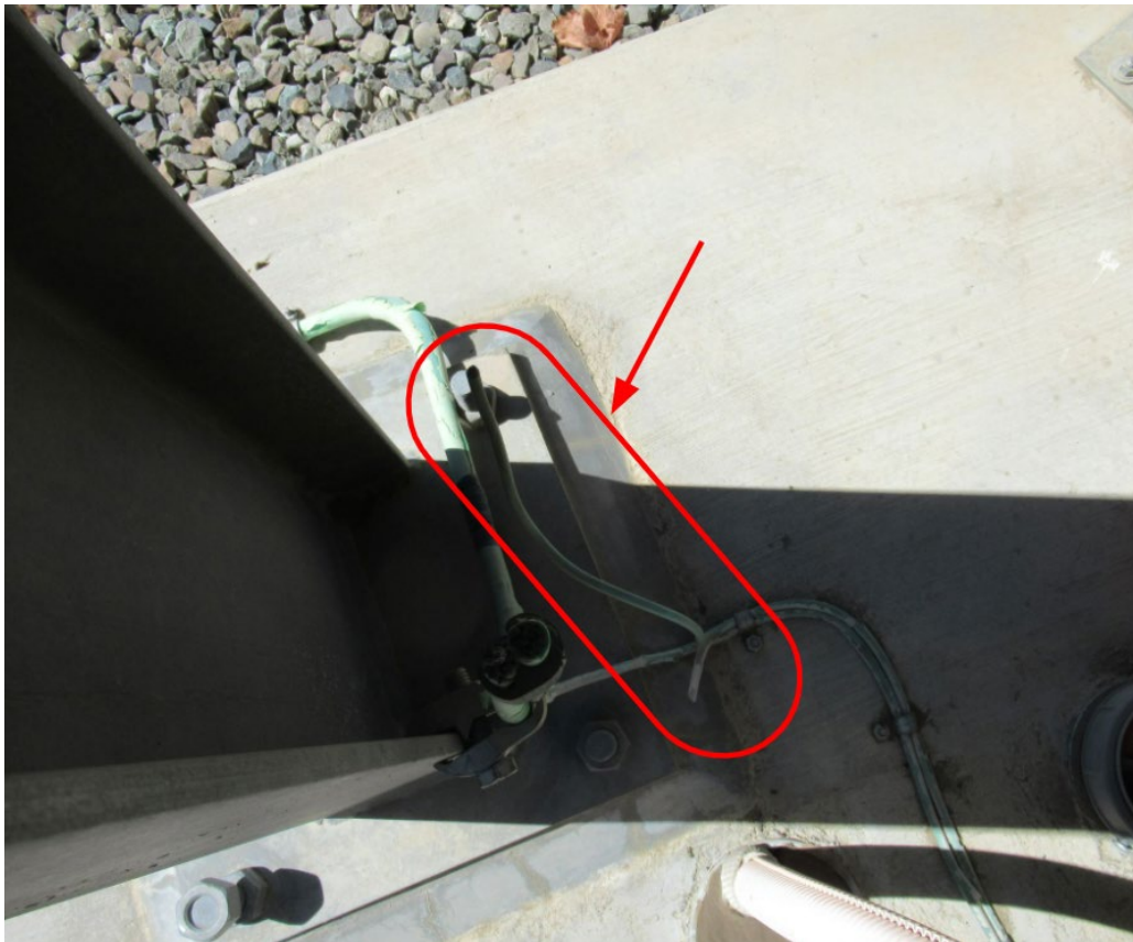
Figure 16: Unbonded ground wire on the Unit 3 PCM.
