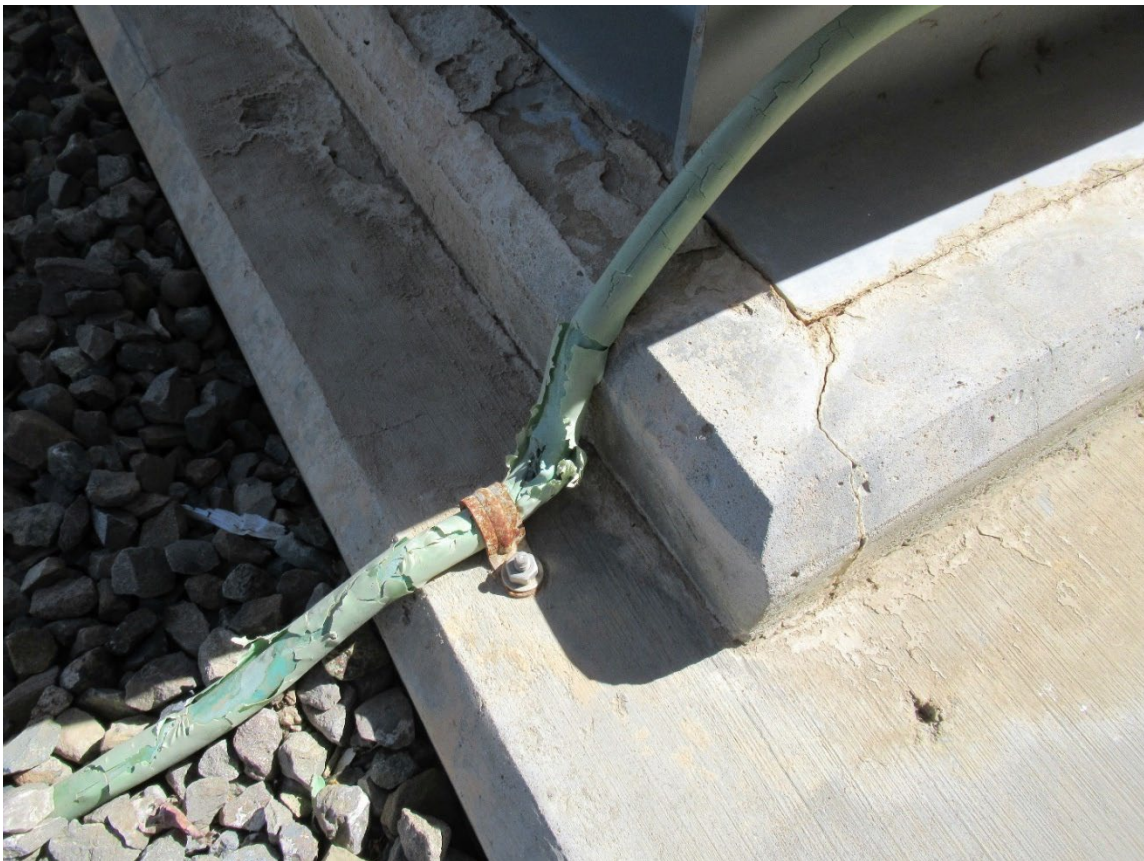
Figure 17: Ground wire with compromised insulation.
