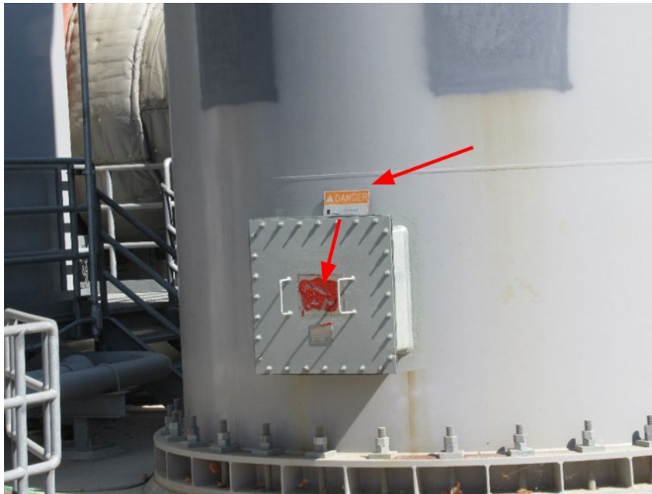
Figure 11 : The VBV at Unit 3 has a detached Confined Space Sign.
