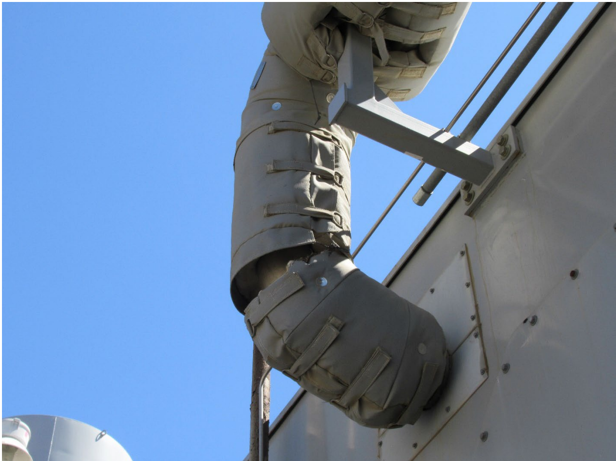
Figure 21: Insulation on the anti-icing system is coming apart.
