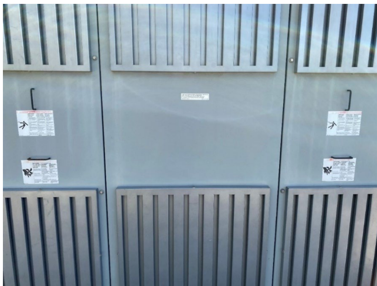
Figure 8 : The PCM transformer near Unit 4 has faded warning signs.
