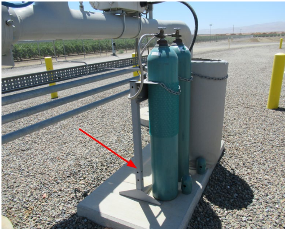
Figure 2: Cylinders in the gas yard are not equipped with two forms of securement.
