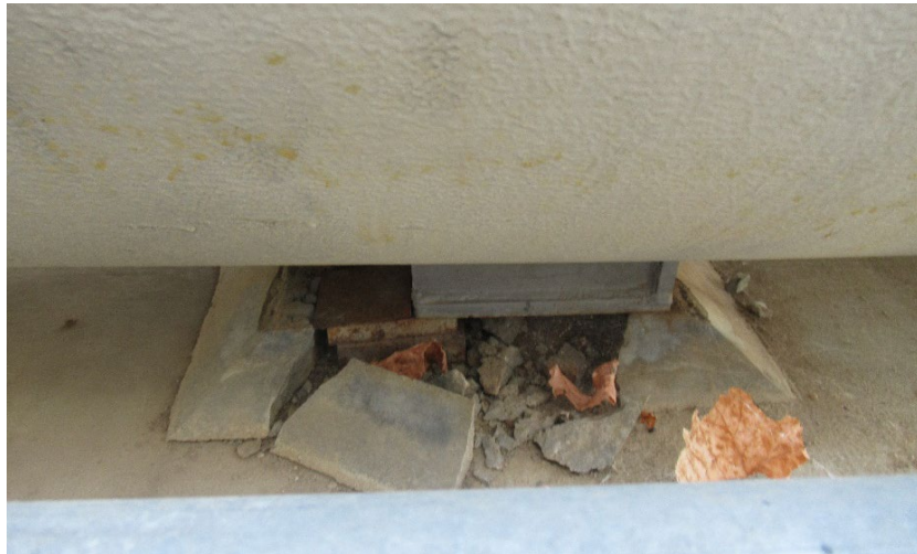
Figure 18 : Spalling concrete on the Unit 2 air fan structural support.
