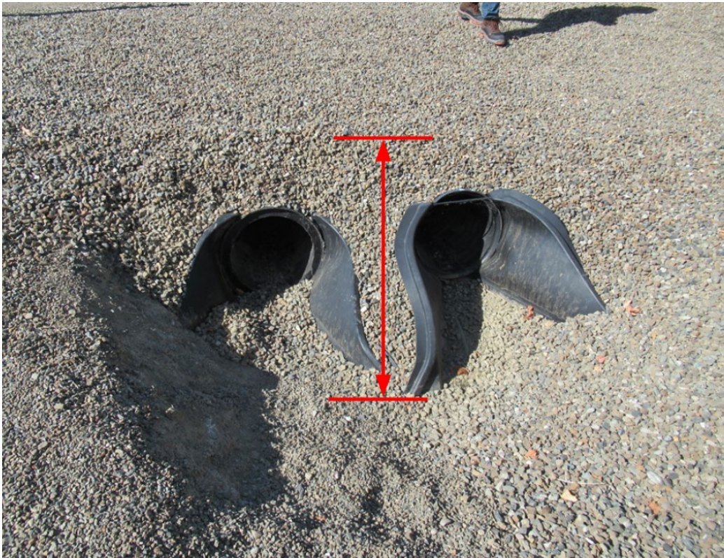
Figure 20: Example of a sudden vertical grade change near a storm drain at Unit 4. The vertical drop blends in with the terrain if standing from the top area of the drain.
