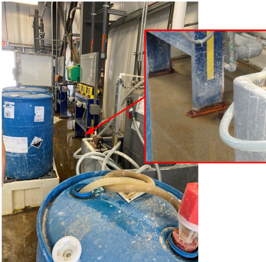
Figure 5: Standing water accumulating in the Enhanced Wastewater System building.
