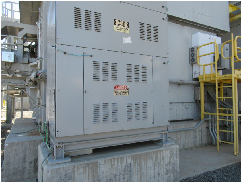
Figure 9: The neutral ground cabinet near the Unit 3 generator has faded and damaged High Voltage Signs
