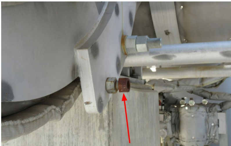
Figure 15 : Lock nut is rusted and loose.
