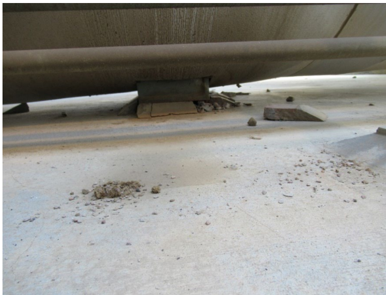
Figure 19 : Spalling concrete on the Unit 3 air fan structural support.
