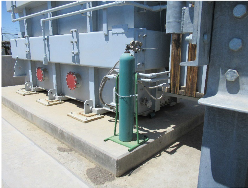
Figure 3 : The cylinder on the spare transformer is not equipped with two forms of securement.
