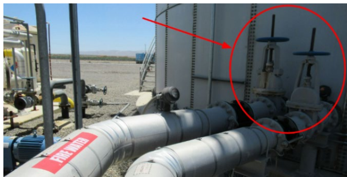
Figure 1: Fire water valves are not physically locked open.
