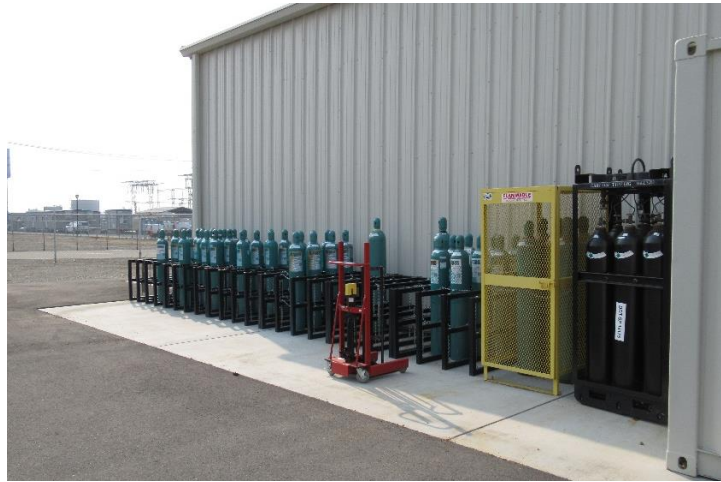
Figure 4: View of the existing high-pressure tank storage area
