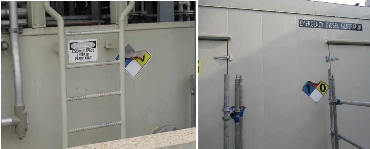
Figure 1: Deteriorated NFPA 704 Hazard Diamond on the (Left) Unit 4 Lube Oil skid and the (Right) emergency diesel generator skid
