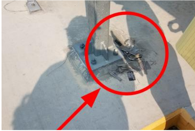
Figure 5: Pile of unattached equipment tags near the fuel gas regulating skid
