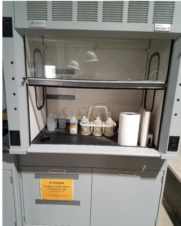
Figure 6: Chemistry lab fume hood is dysfunctional and used as a storage area.
