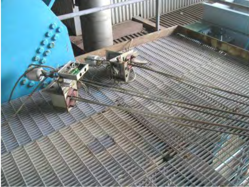
Figure 4 -- Disused equipment allowed to accumulate on Level 104 of Units 6 and 7.
