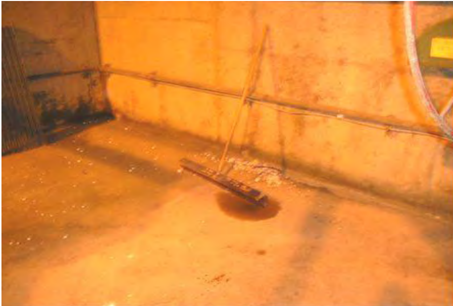
Figure 11 -- Insulation from the over head pipe; no asbestos containment precautions are evident.
