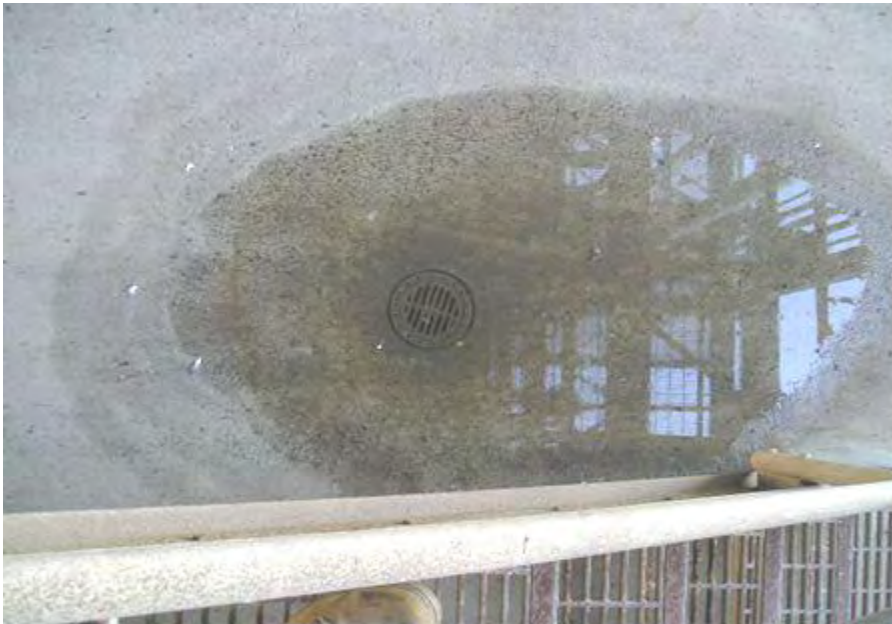
Figure 9 -- Standing water caused by a clogged drain on Level 88 of Units 6 and 7.
