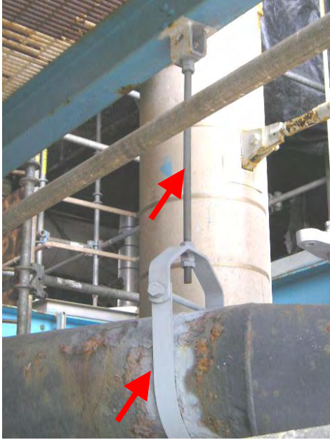
Figure 26 -- This is a photo of a new hanger and pipe support on an older pipe.
