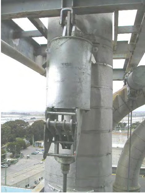
Figure 22 -- Close-up view of a new spring support.
