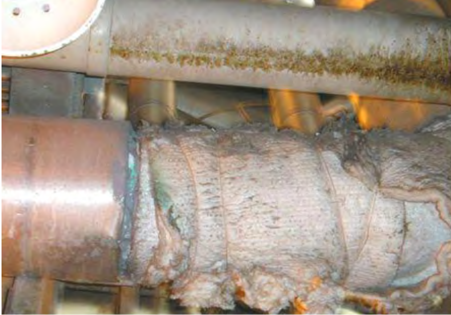
Figure 10 -- Frangible insulation falling off an exposed pipe in the basement of Units 6 and 7. The pipes lack blue banding, which would indicate the absence of asbestos. Therefore, asbestos is assumed to be present.
