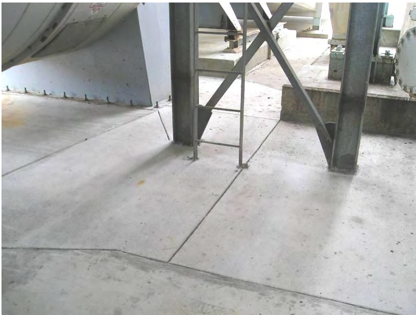
Figure 14 -- To prevent water accumulation, the plant used epoxy cement to re-grade the area for proper drainage.
