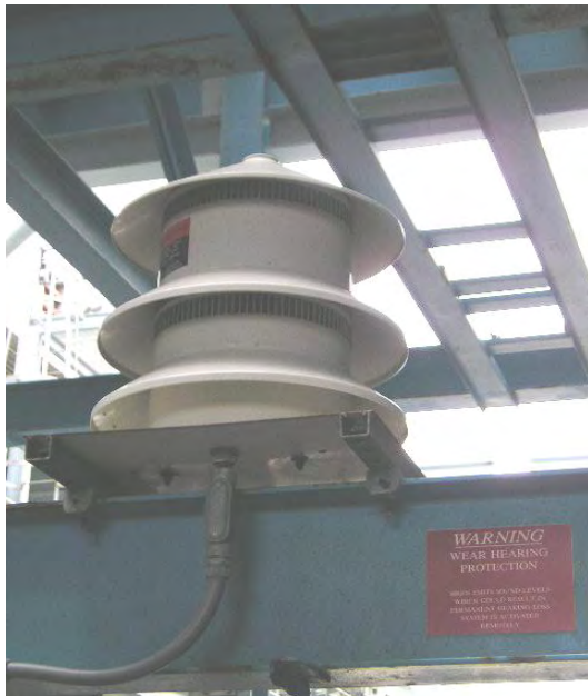
Figure 29 -- This is a photo of the new siren installed on Level 88 of Units 6 & 7.
