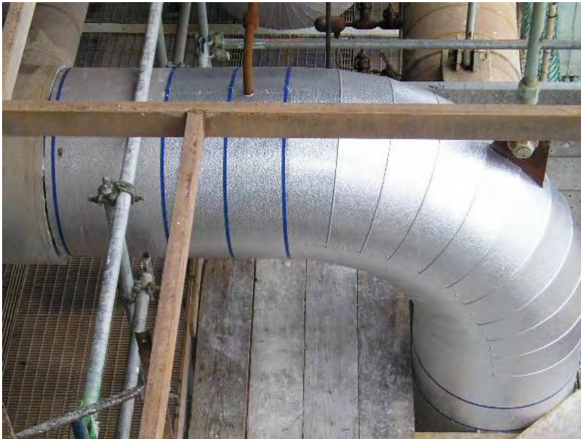
Figure 16 -- Plant staff used blue banding and dimpled aluminum wrapping to indicate non-asbestos pipe insulation.
