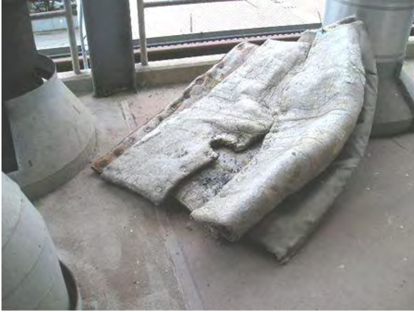
Figure 8 -- Insulation, possibly containing asbestos, on Level 104 of Units 6 and 7.
