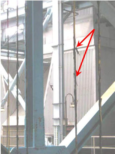
Figure 20 -- Severely deteriorated pipe hanger rods visible from Level 102 of Units 6 and 7.
