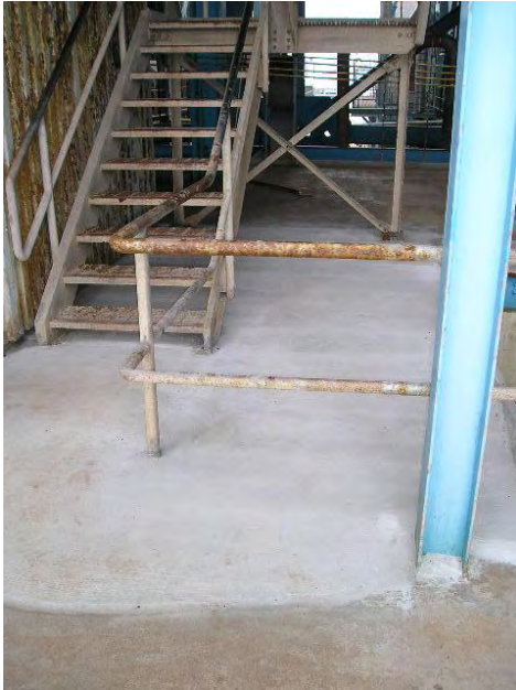
Figure 13 -- The plant was unable to unclog the plugged drain. Rather, the plant applied epoxy cement over it to correct the low spot and allow proper drainage. Also see Figure 9.
