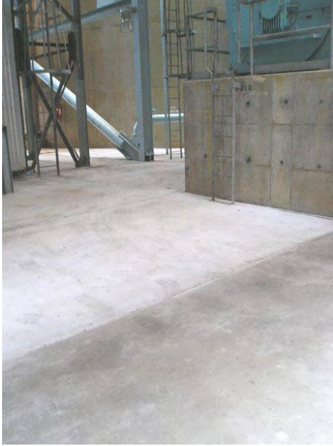
Figure 15 -- To prevent water accumulation, the plant used epoxy cement to re-grade the area for proper drainage.
