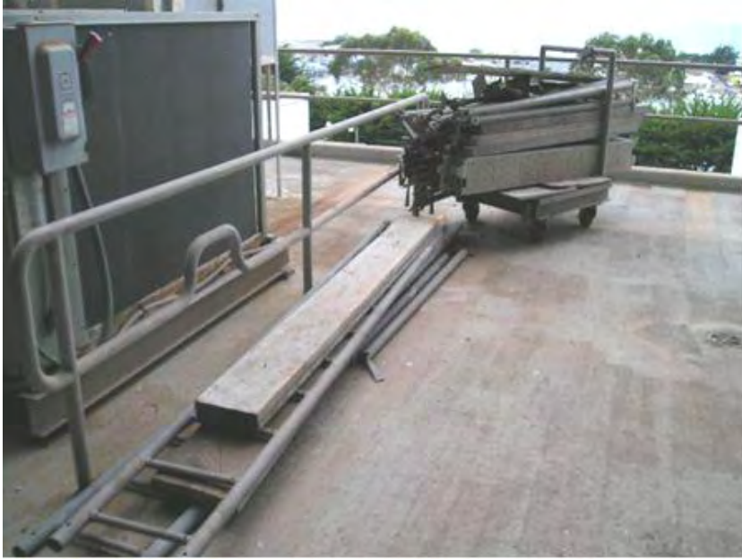
Figure 6 -- Disused scaffolds accumulating on Level 88 of Units 6 and 7.
