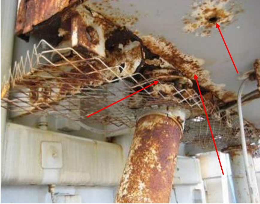
Photo 4: Severe corrosion at lower portion of heat exchanger housing.
