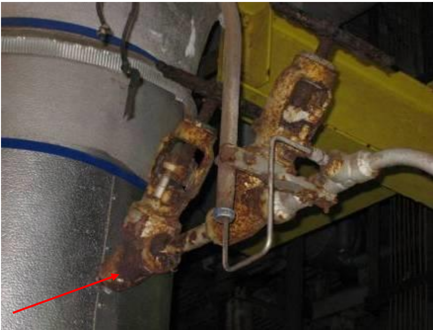
Photo 7: Severely corroded root valve.
