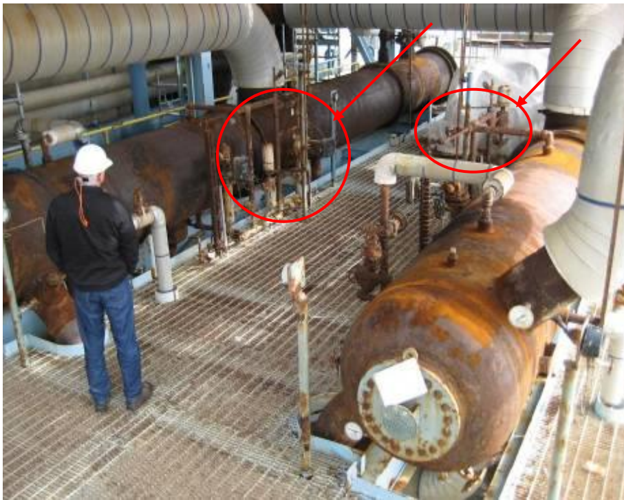
Photo 9: Corroded piping attached to two feedwater heaters
