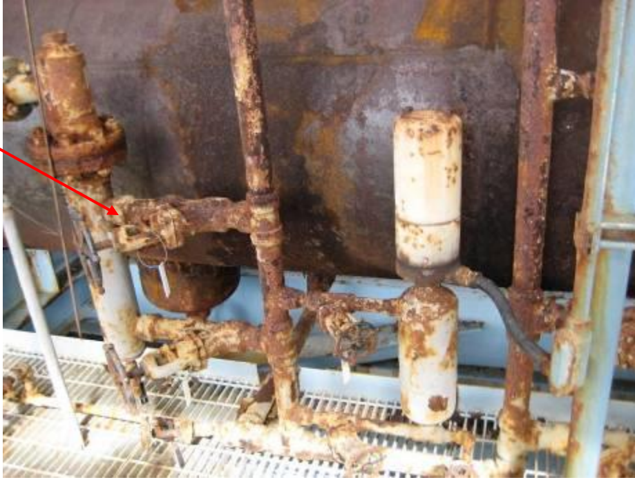
Photo 10: Corroded feedwater pipes.
