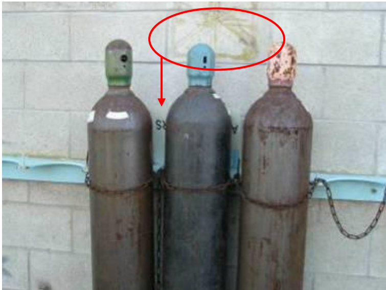
Photo 26: Identification sign not visible behind argon gas tanks.
