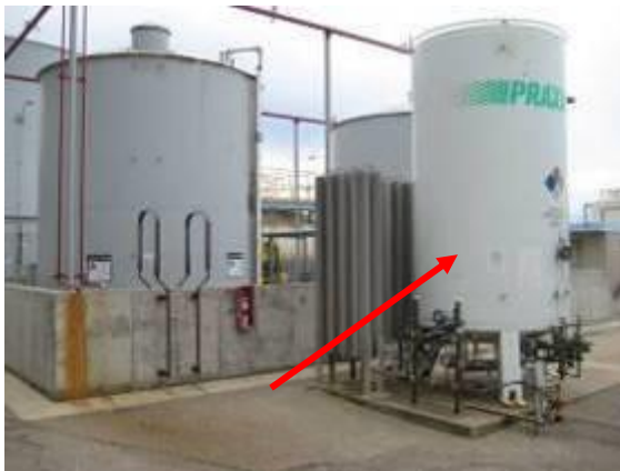
Photo 33: Bulk nitrogen storage tank is not recorded on plant schematic.
