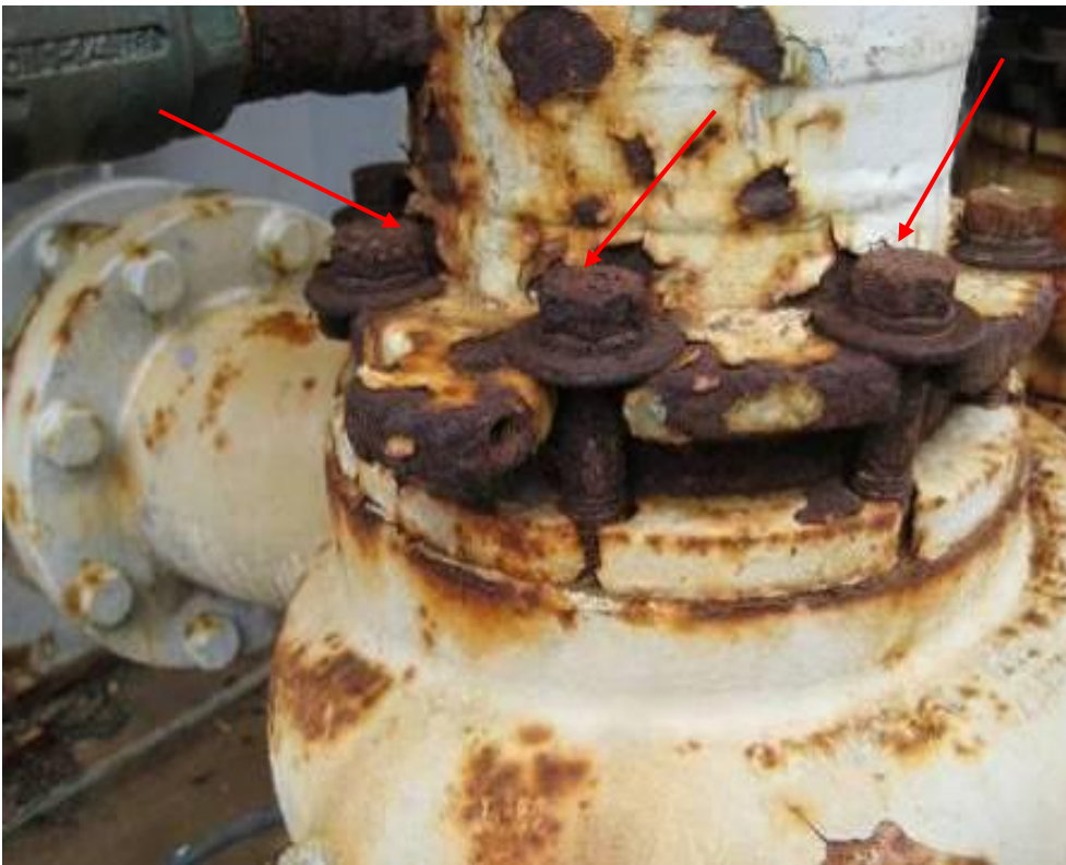
Photo 3: Severe corrosion at circulating oil pump flange bolts.
