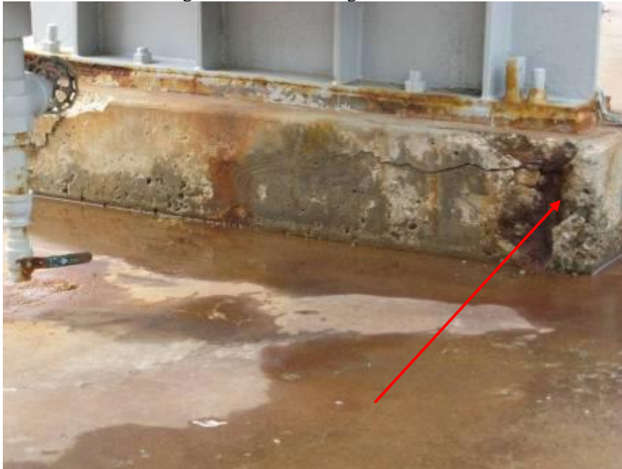
Photo 17: Cracked foundation exposes rusted rebar
