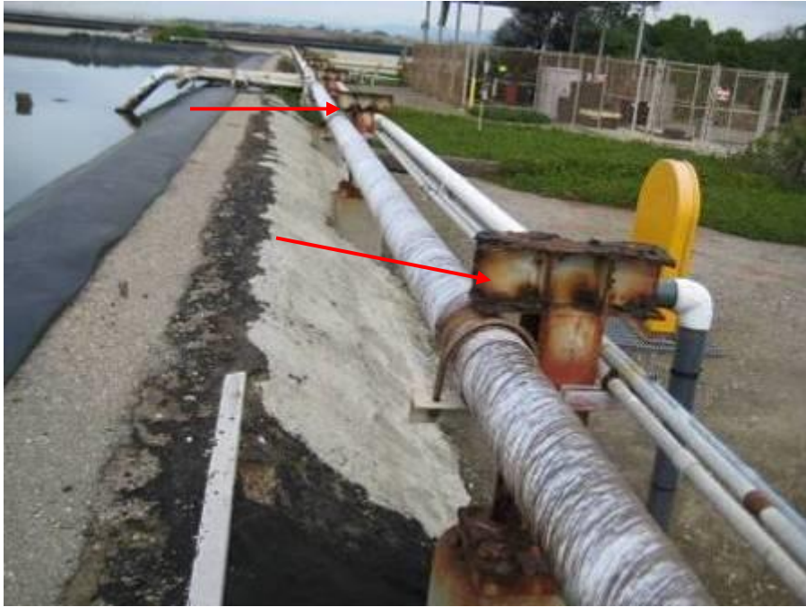
Photo 14: Corroded pipe supports and anchors along the RO discharge pipe.
