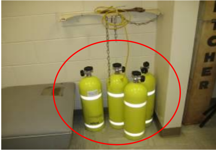
Photo 25: Unsecured, high pressure SCBA tanks in the First Aid room
