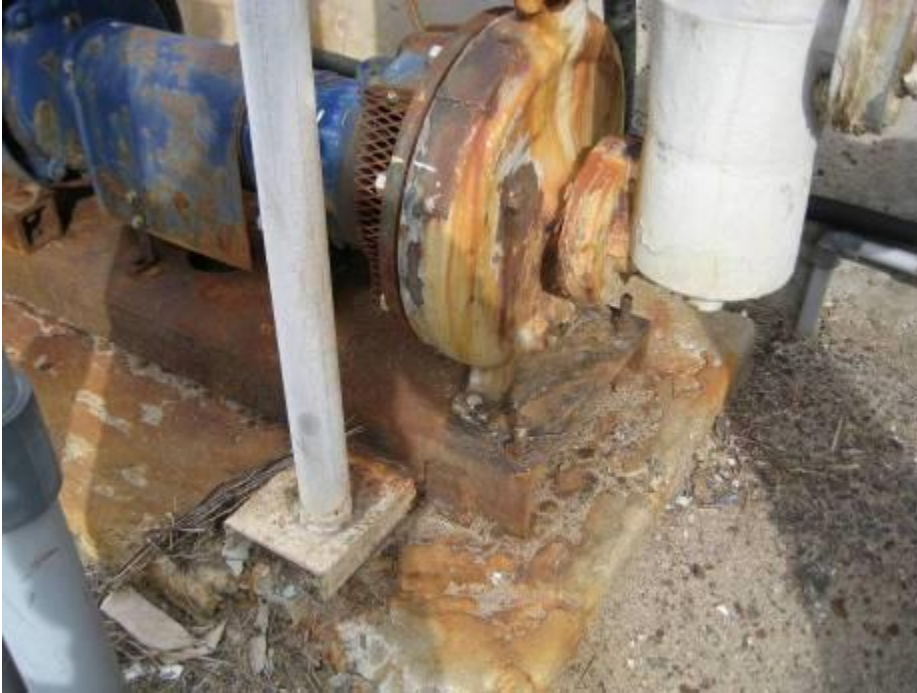
Photo 20: Crumbling pump foundation
