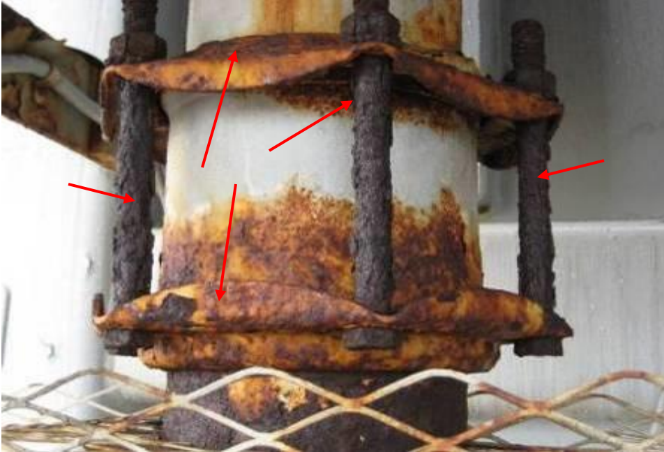
Photo 2: Severe corrosion of flange that connects bolts at lower housing.
