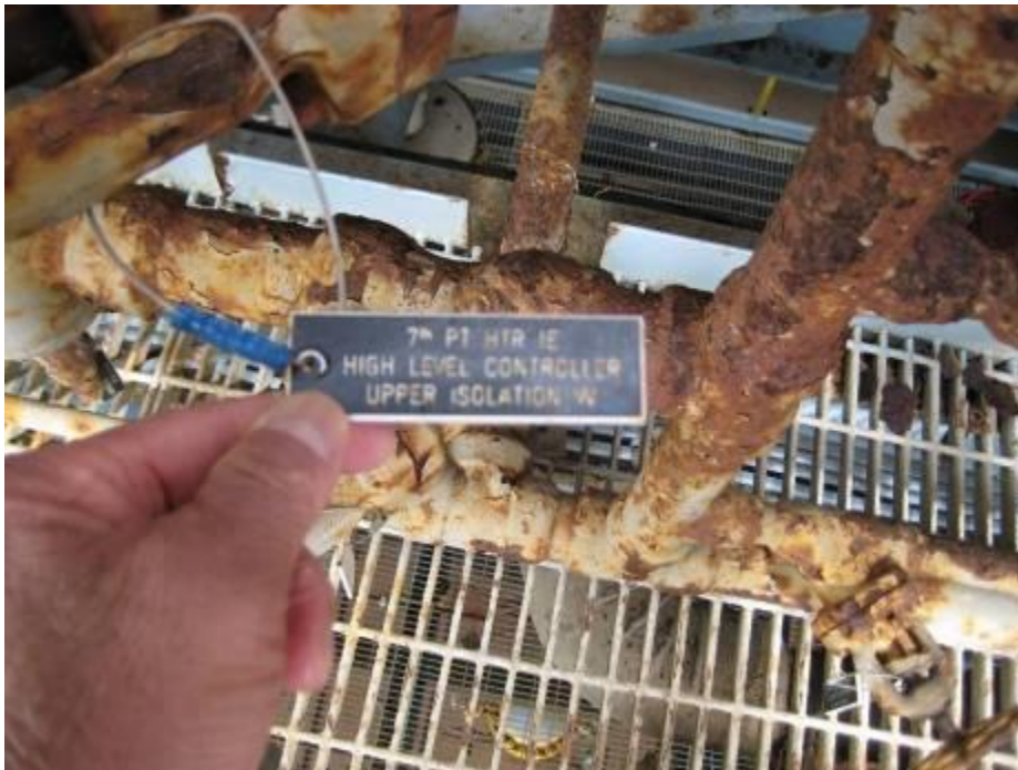
Photo 11: Close-up of corroded pipes.
