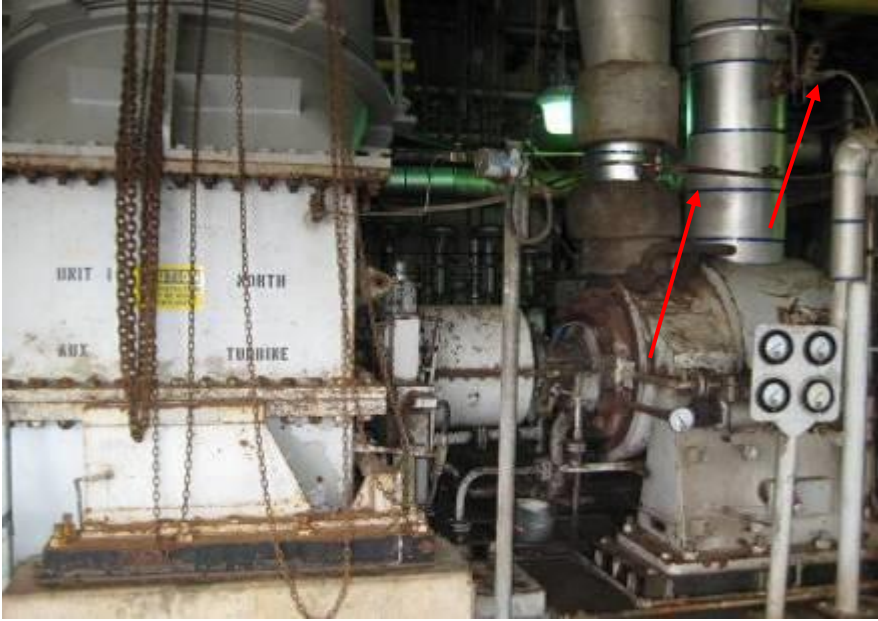
Photo 6: Pressure gauge sensing line; BFP suction and discharge.
