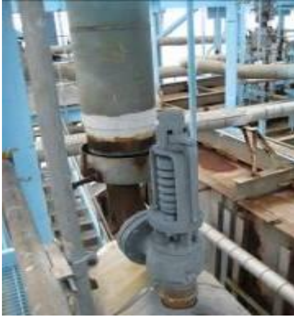
Photo 28: Safety valve number 02-PSV-3307 lacks identification tag
