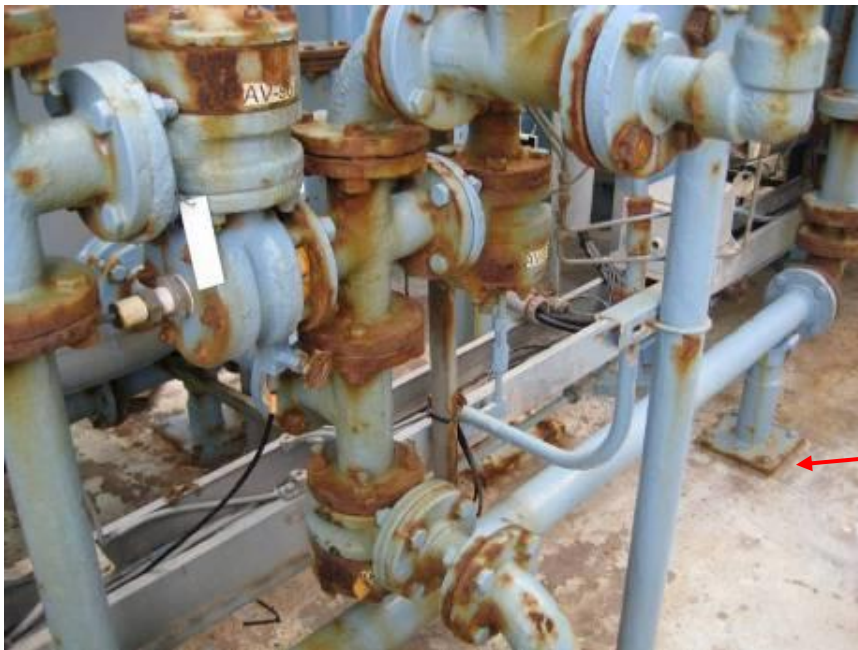
Photo 13: Piping support system; corrosion sheared bolt heads off stems.
