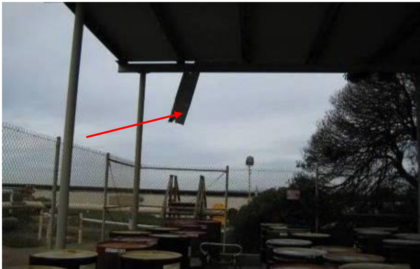
Photo 24: A loose roof panel hangs precariously over the storage area
