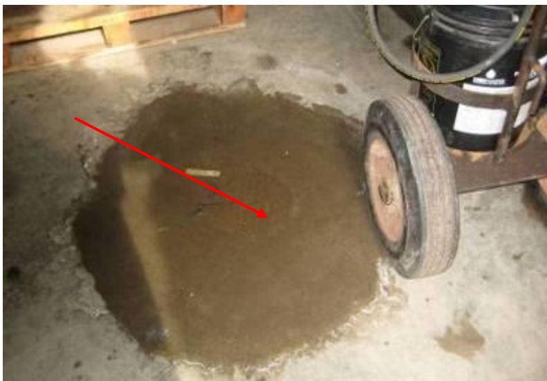
Photo 35: Clogged floor drain in the grease room.
