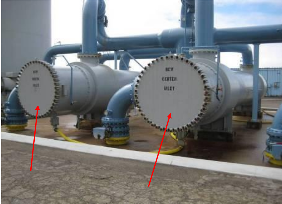
Photo 16: Two cooling water heat exchangers.
