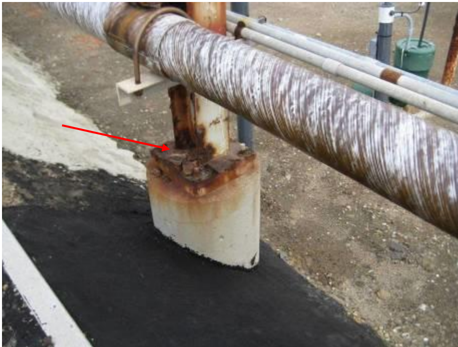
Photo 15: Corroded support and anchor
