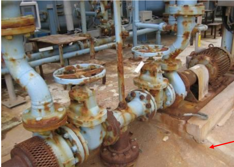
Photo 12: Cracked foundation beneath corroded pump and motor.
