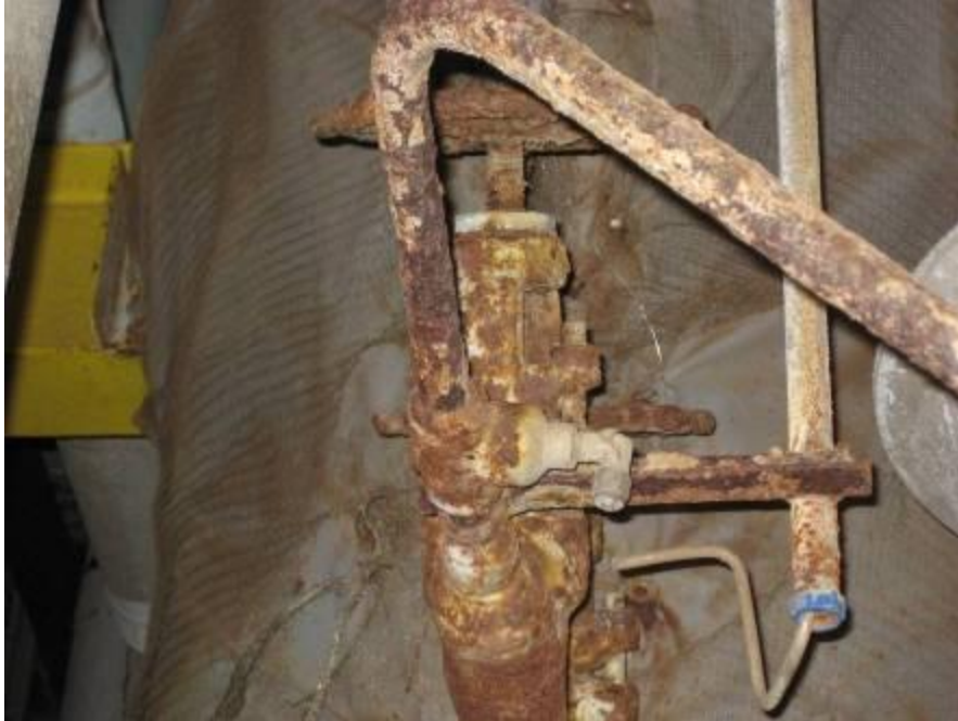
Photo 8: Corroded root valve and piping.
