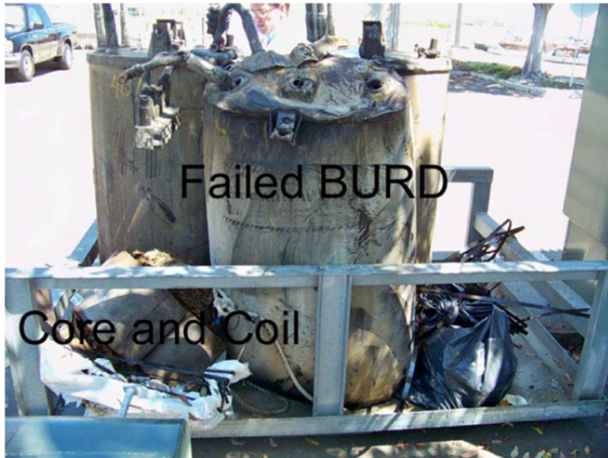
Figure II-6 D2 (BURD Transformer): Catastrophic Failure
