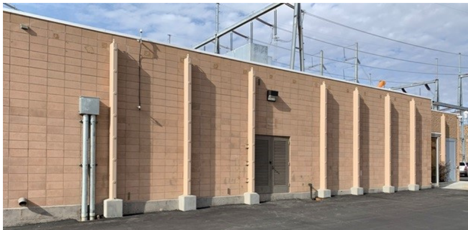
Figure III-6 Completed Seismic Retrofit of a Reinforced Masonry Wall at an SCE AA Substation; Vertical Pipes Added and Ties from Walls to Roof Added
