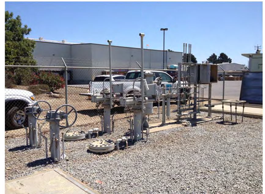
Harkins Rd. Regulator Station (Salinas)
