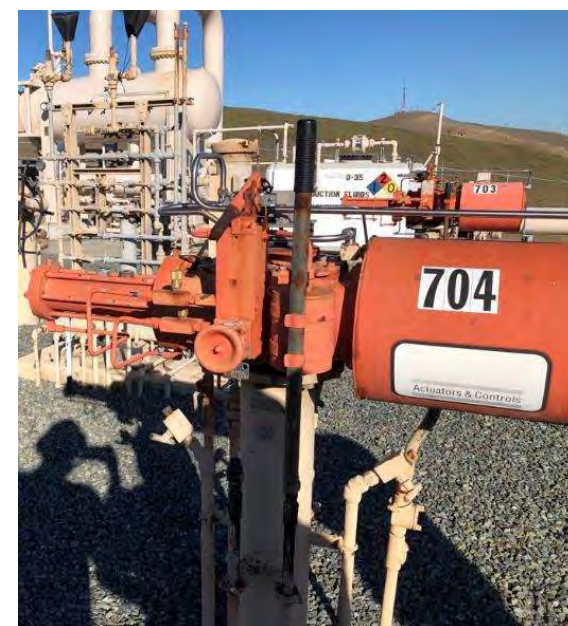
Continuous High Bleed Device (Los Medanos)
