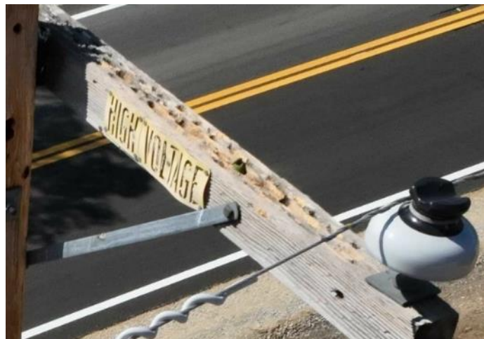
Figure 17: Crossarm integrity issues visible from aerial photos but not visible from the ground.
