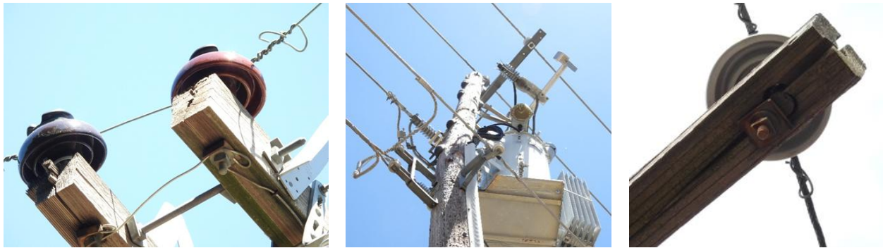
Figure 12: Representative B-Tag Field Observations (Conductor Strain on Insulators (left); Cracked Pole Below Voltage Regulator (middle); Crossarm Damage at Insulator (right))
