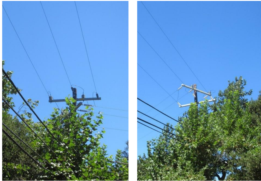
Figure 19: Representative VMOM Proactive Project Field Observations (Tree Approaching MDR With No Prescription in the System of Record)
