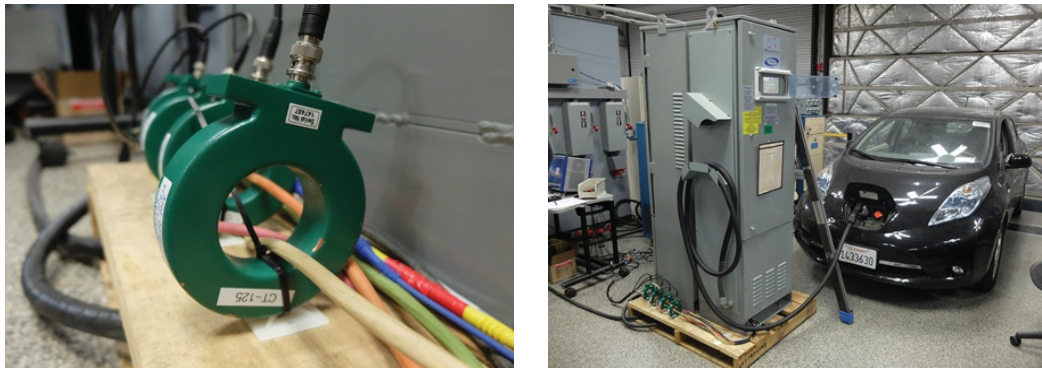
Figure J – Each bidirectional vehicle/charger system was tested prior to deployment: Nissan Leaf and Princeton Power Systems Charger under test
