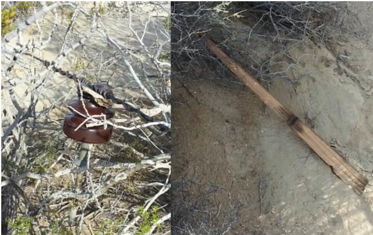
Figure 2. The left and right images show the insulator and crossarm that were supported on pole number 43502S.
