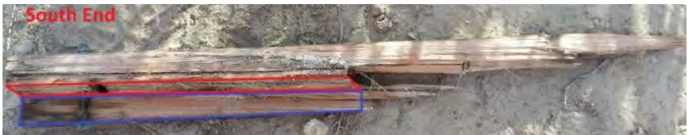
Figure A-10: "South End – Broken Piece 1" showing part of the Vertical Shearing Plane and part of the Horizontal Shearing Plane. It is clear from this figure that the "Anti-split" throughbolt caused the Horizontal Shearing Plane. Source: SED
