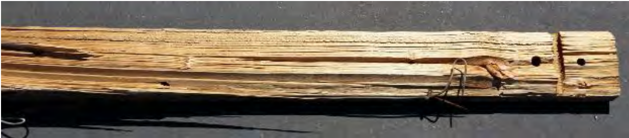
Figure B-8: The front face of Specimen 3 – right side close-up.
