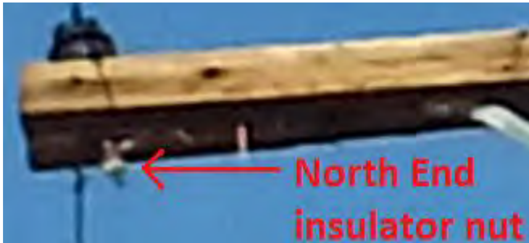
Figure A-8: The photo shows the insulator nut on the "North End" insulator. Source: SED.
