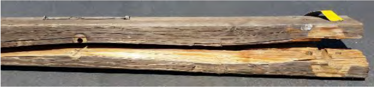
Figure B-6: The top face of Specimen 2 – right side close-up
