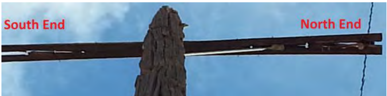
Figure A-1: The crossarm on SCE pole number 43502S. Source: SED
