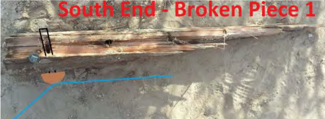
Figure A-6: "South End – Broken Piece 1" (photo 4/4) showing where the insulator & pin would have been installed. Source: SED.
