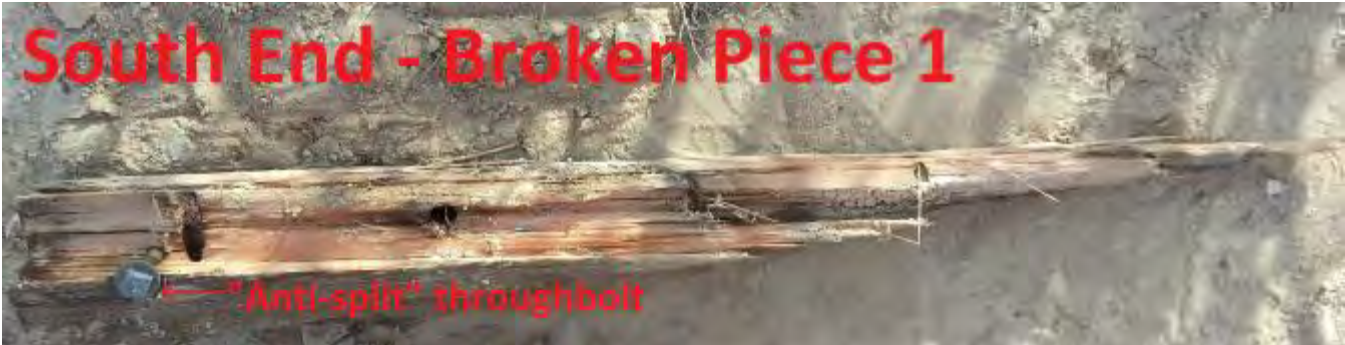
Figure A-5: "South End – Broken Piece 1" (photo 3/4). The "Anti-split" throughbolt did not support insulators. Source: SED
