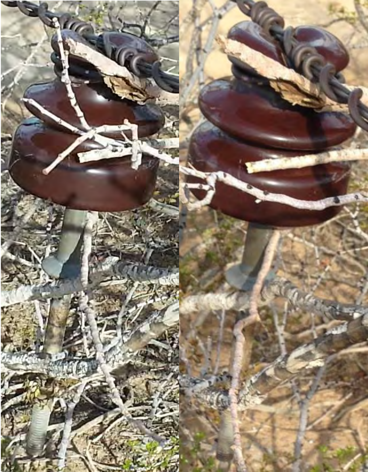
Figure A-12: Two views of the insulator that had been supported on the South End of the failed crossarm of pole number 43502S showing no nut attached to threaded portion of the insulator pin. Source: SED (left) and SCE (right)
