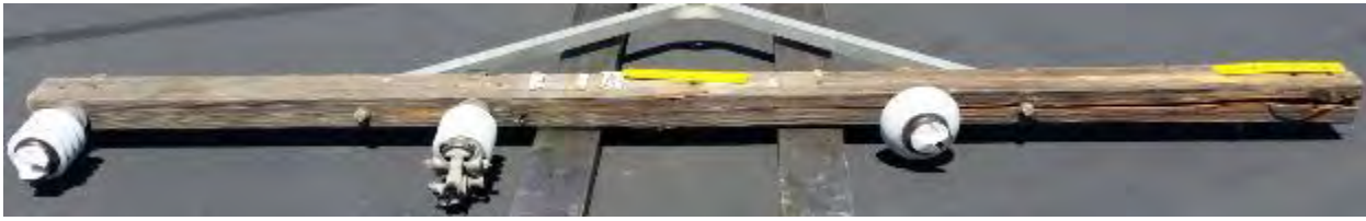
Figure B-10: The top face (the face supporting the three insulators) of Specimen 5.
